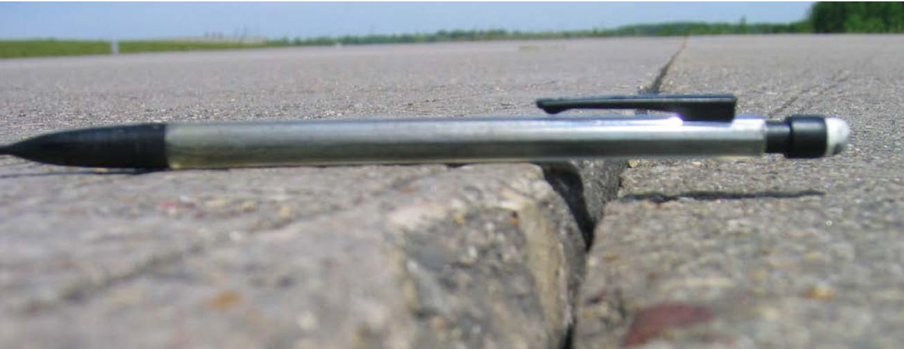
Closeup of transverse joint faulting. Source: APTech.
