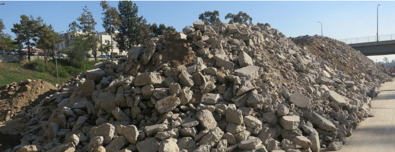
This stockpile of concrete rubble from pavement reconstruction is ready for crushing into recycled aggregate. Source: APTech.
