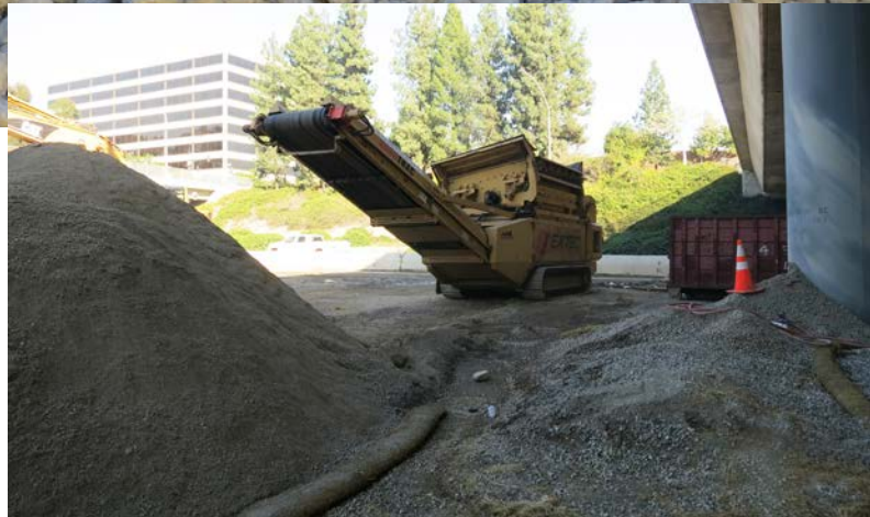
This mobile concrete crusher on a jobsite is used to break down the concrete rubble. Source: APTech.
