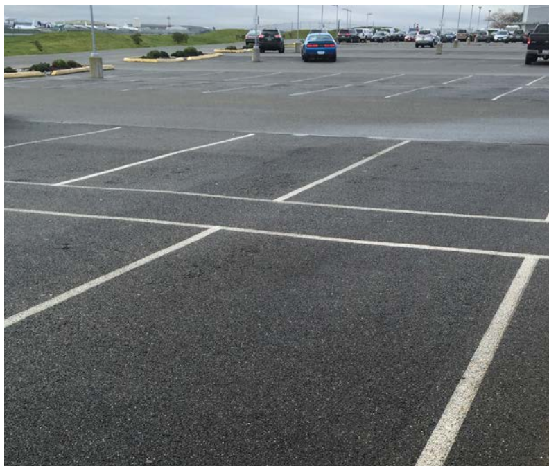
Porous pavements have been used extensively in parking lots like this one in Everett, WA. Source: APTech.
