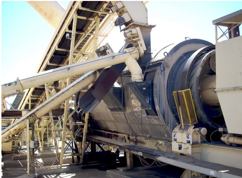
Shown here is a double barrel hot mix plant with drum injection ports for baghouse fines and recycled materials (RAP and RAS). The recycled materials are added between the inner and outer barrels to protect them from the intense heat and direct flame located within the inner barrel. Source: Ray Bonaquist, Advanced Asphalt Technologies, LLC.
