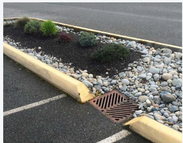
Drainage structures like this one carry away storm water flow that exceeds the holding capacity of the porous pavement and stone reservoir. Source: APTech.
