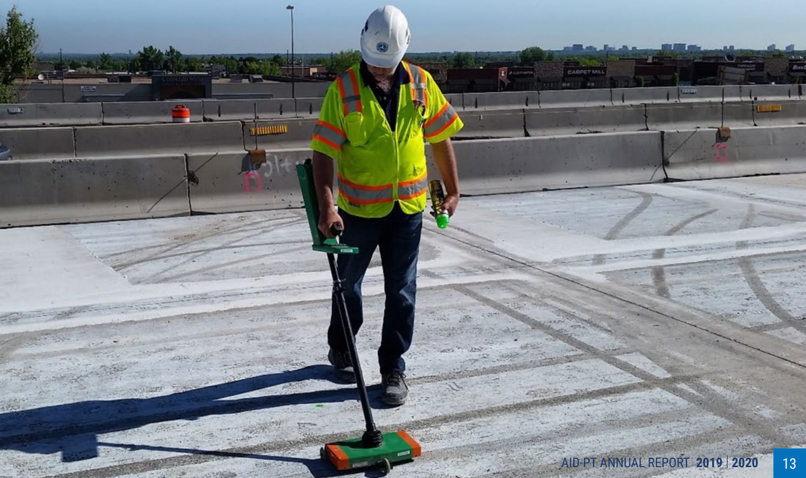
Pulse induction technology scanning for determining thickness of hardened concrete. Source: FHWA
