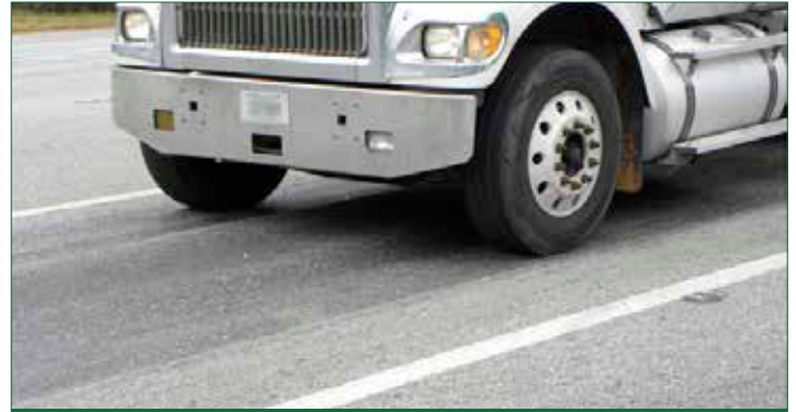
Figure 2(a): Typical rutting of existing asphalt.
