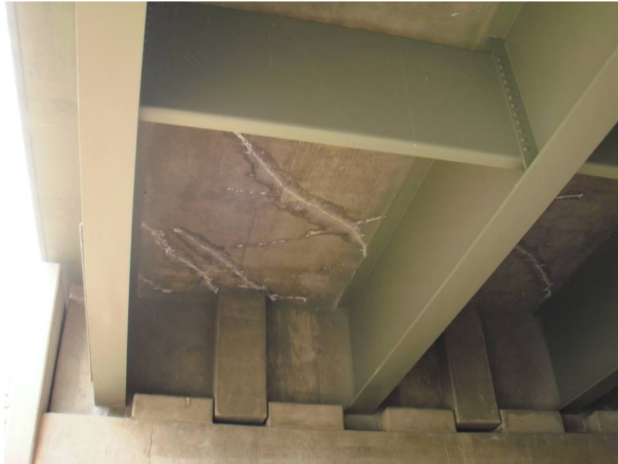
Figure 8.2.1.3-2 Typical Cracking on the I-80 Bridges (source: Utah DOT)
