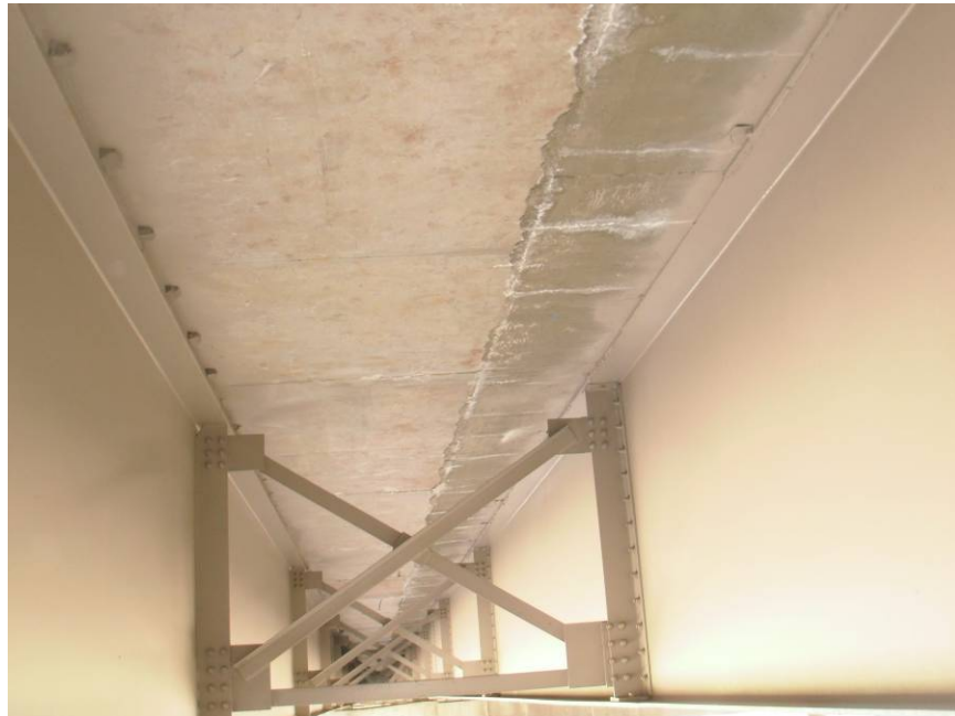
Figure 7.8-1 Cracking in Closure Pour Concrete
