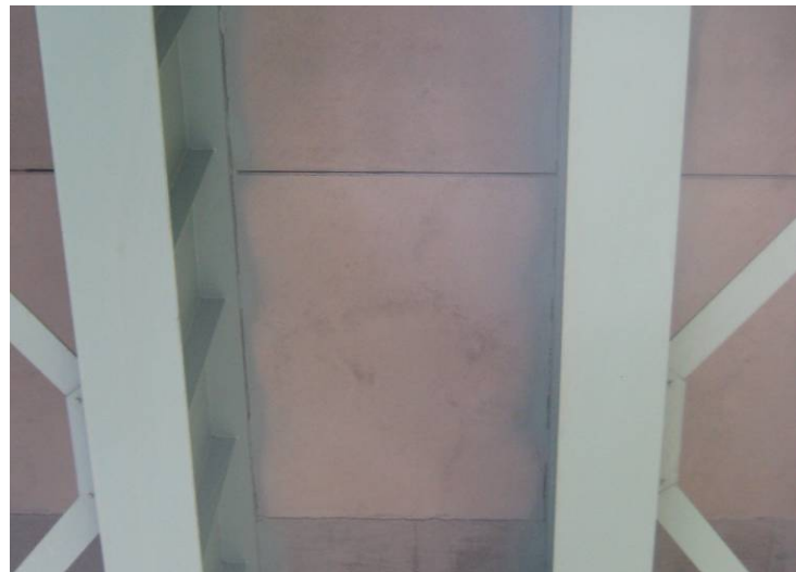
Figure 2.6.1.1-2 Underside of Full Depth Precast Deck Panels (after 20 years in service)
