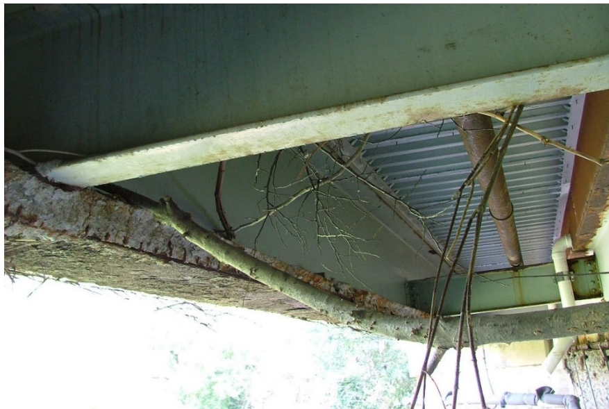
Figure 16.1.38 Drift Lodged in a Superstructure
