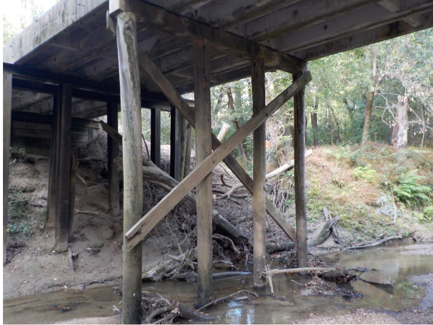
Figure 14.5.37 Timber Pile Bents with Debris Accumulation
