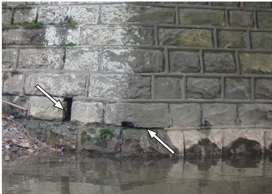
Figure 14.5.36 Stone Masonry Abutment with Deteriorated Joints
