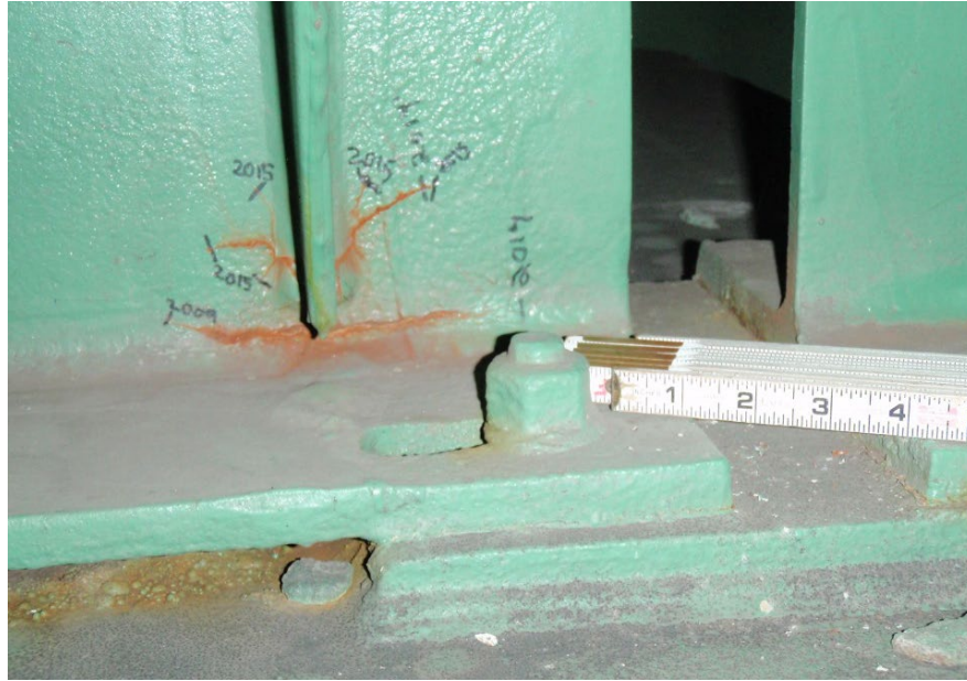
Figure 7.3.36 Web Gap Crack between Bottom Flange and Vertical Stiffener
