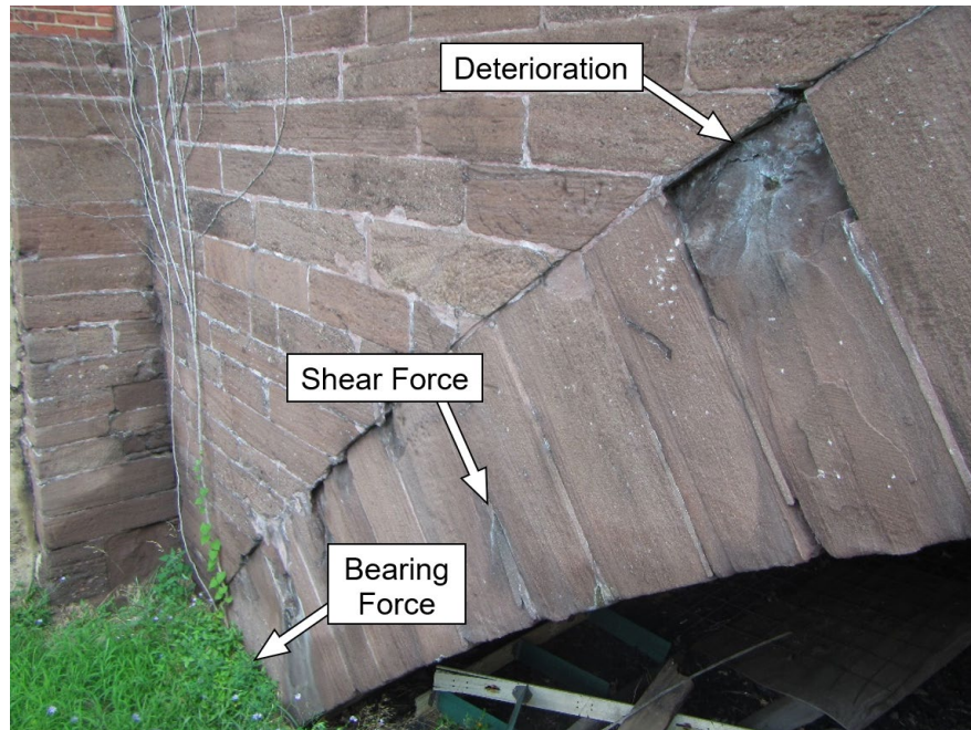
Figure 11.5.11 Masonry Stone Arch with Deterioration
