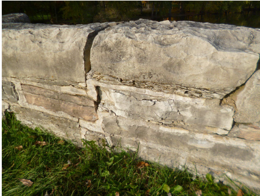
Figure 11.5.14 Top of Spandrel Wall Exposed to Traffic
