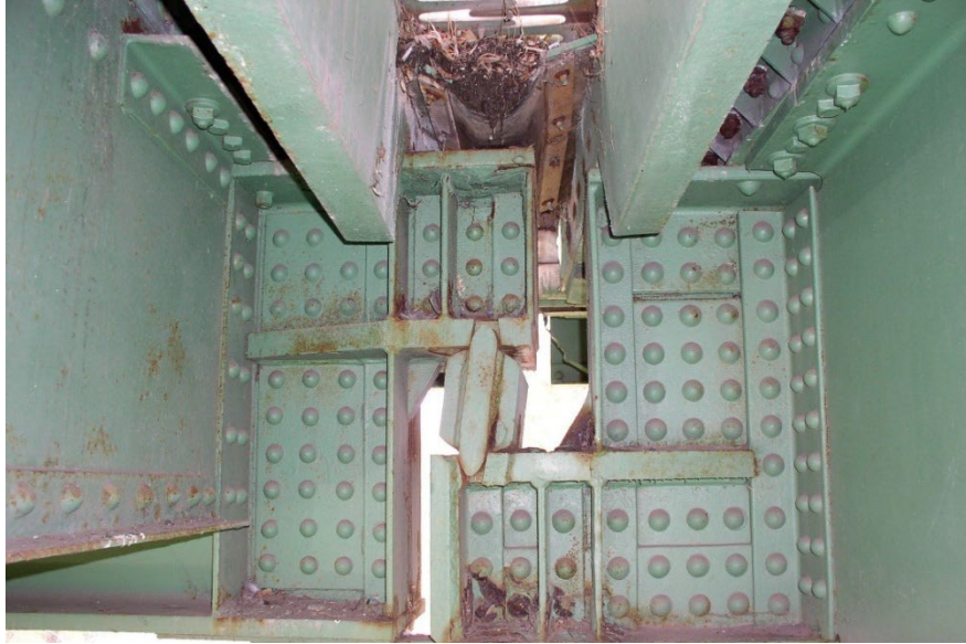
Figure 8.5.33 Drainage Trough with Debris Accumulation
