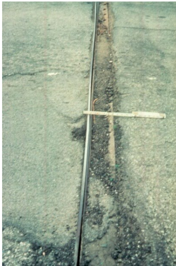
Figure 8.5.25 Deck Joint with Dirt and Debris Accumulation
