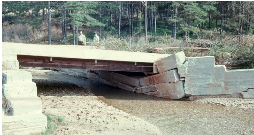
Figure 14.5.27 Abutment Failure from Undermining due to Scour
