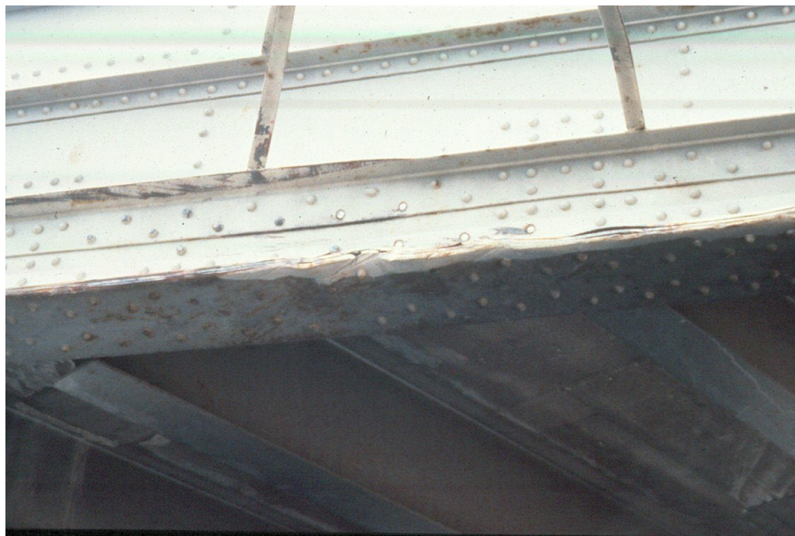
Figure 10.4.22 Collision Damage to Flange on a Through Girder Bridge
