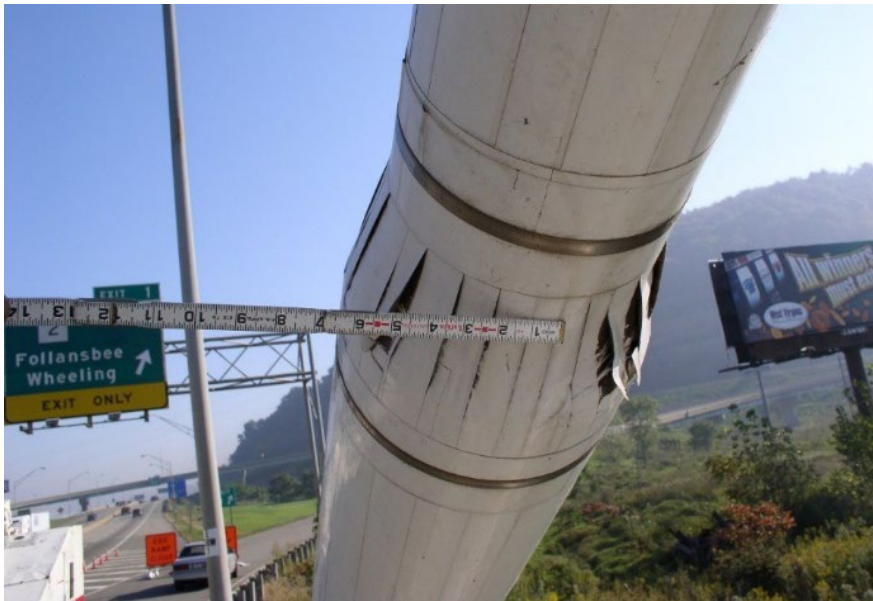
Figure 12.2.5 Deformed Cable Wrapping – Possible Broken or Corroded Wires
