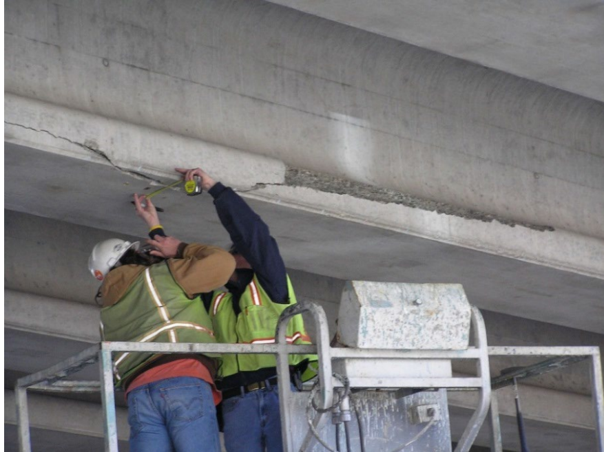
Figure 9.4.43 Inspectors Evaluating Collision Damage on Prestressed Concrete I-beam
