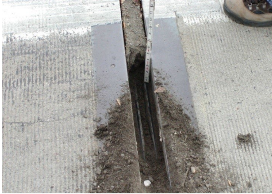
Figure 8.5.26 Soil and Debris in a Compression Seal Joint
