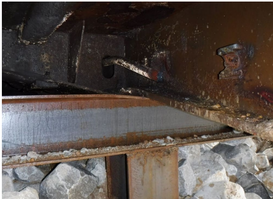
Figure 10.4.62 Flat Car Channel Beam and Bent Cap with Distortion
