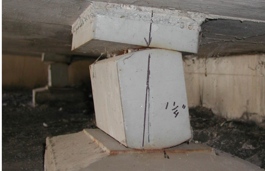
Figure 13.6.7 Excessive Tilt in a Segmental Rocker
