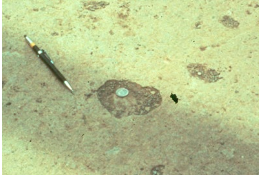
Figure 7.1.19 Light or Minor Scaling
