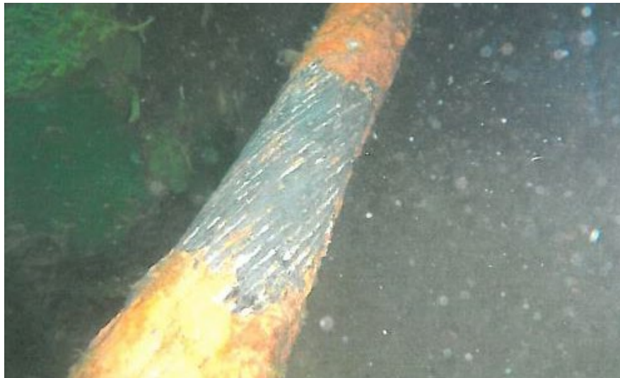
Figure 12.4.3 Cable Corrosion within Pontoon Port
