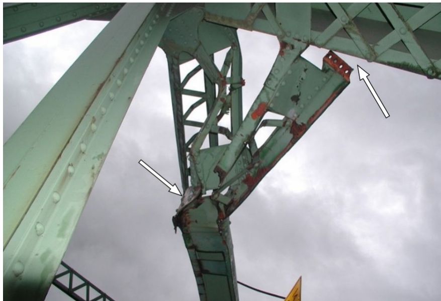
Figure 10.4.64 Collision Damage to Portal Bracing
