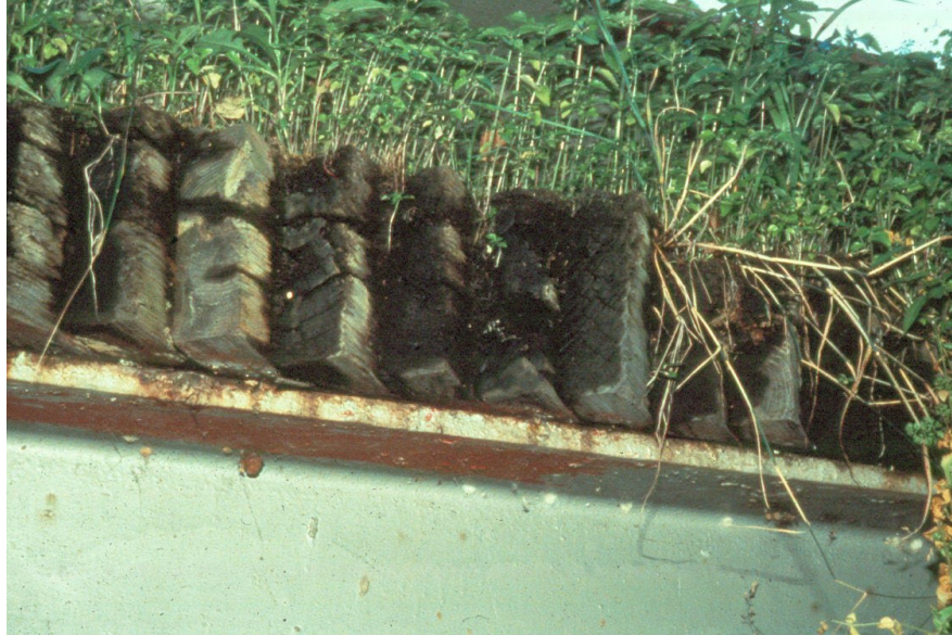
Figure 8.3.10 Timber Deck Exposed to Drainage, Resulting in Decay and Plant Growth
