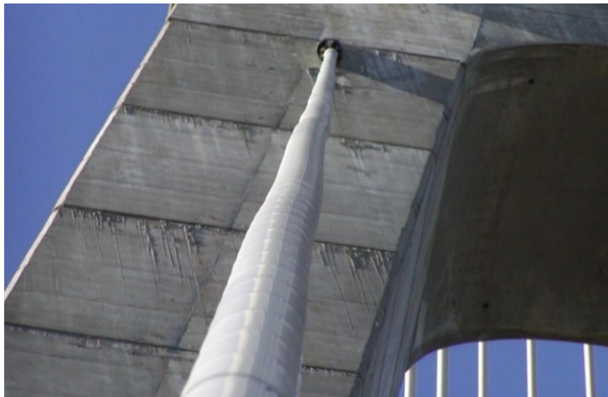
Figure 12.2.9 Bulging of Cable Sheathing
