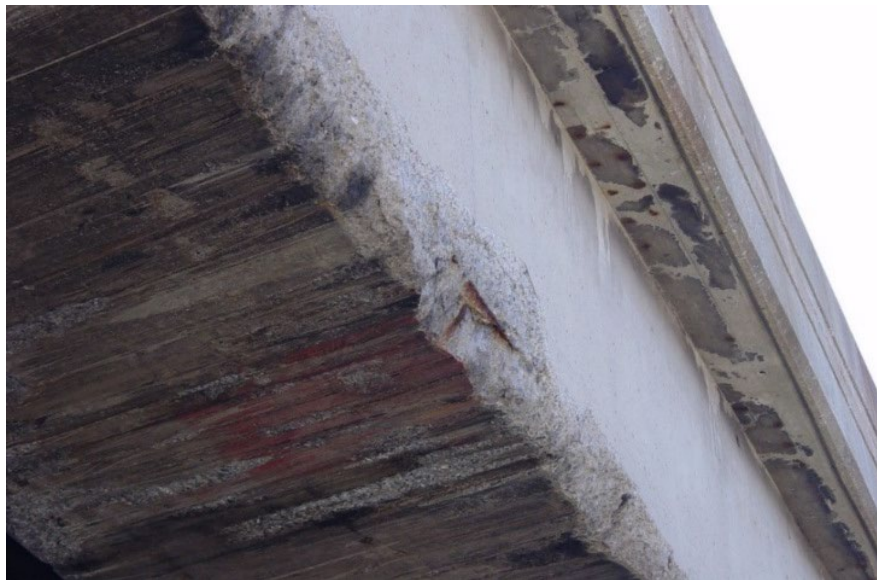
Figure 9.4.42 Collision Damage to Tee Beam Bridge over a Highway
