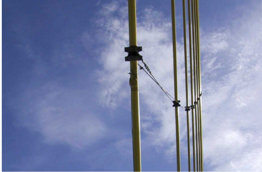
Figure 5.2.33 Crossties between Cables
