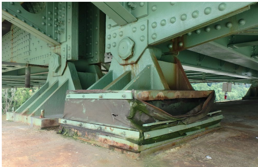
Figure 13.3.6 Failed Roller Nest Skirt
