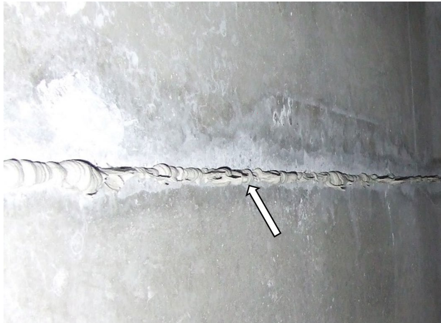
Figure 9.4.50 Close-up View of Box Girder Top Flange Joint with Epoxy Joint Material
