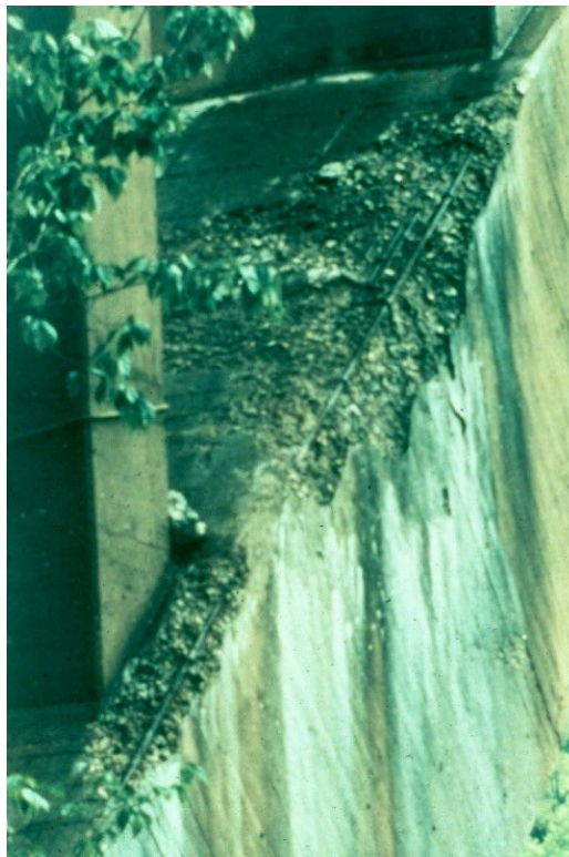
Figure 9.4.37 Scaling and Contamination on an Arch Rib Due to a Failed Drainage System
