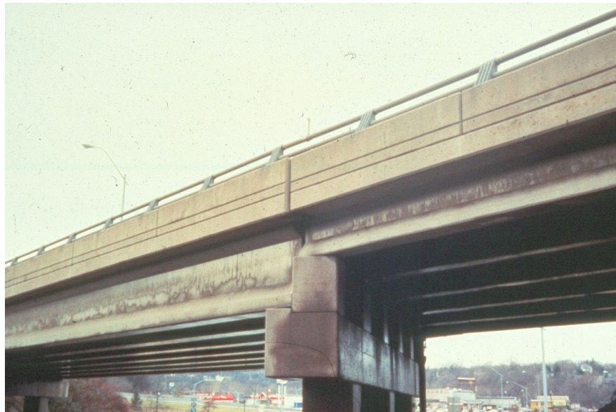
Figure 9.4.39 Water Leakage at Deck Joint Between Spans
