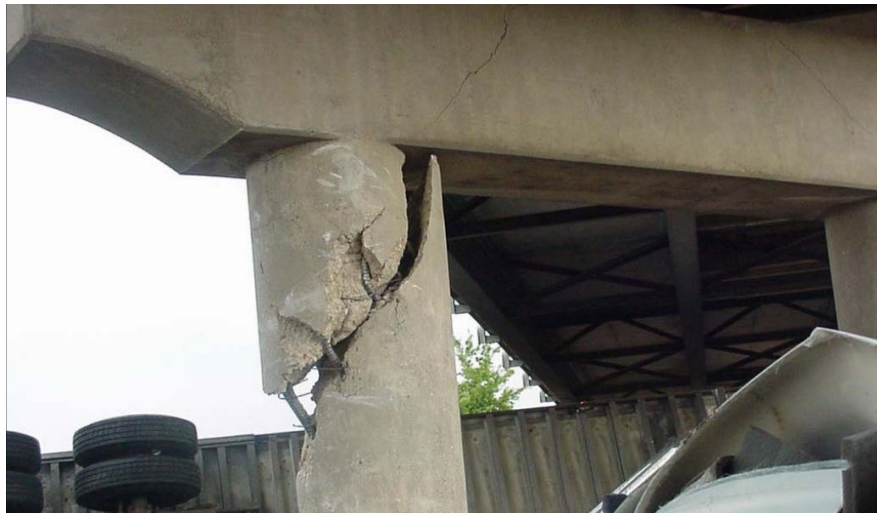
Figure 14.5.25 Collision Damage to Concrete Pier Column
