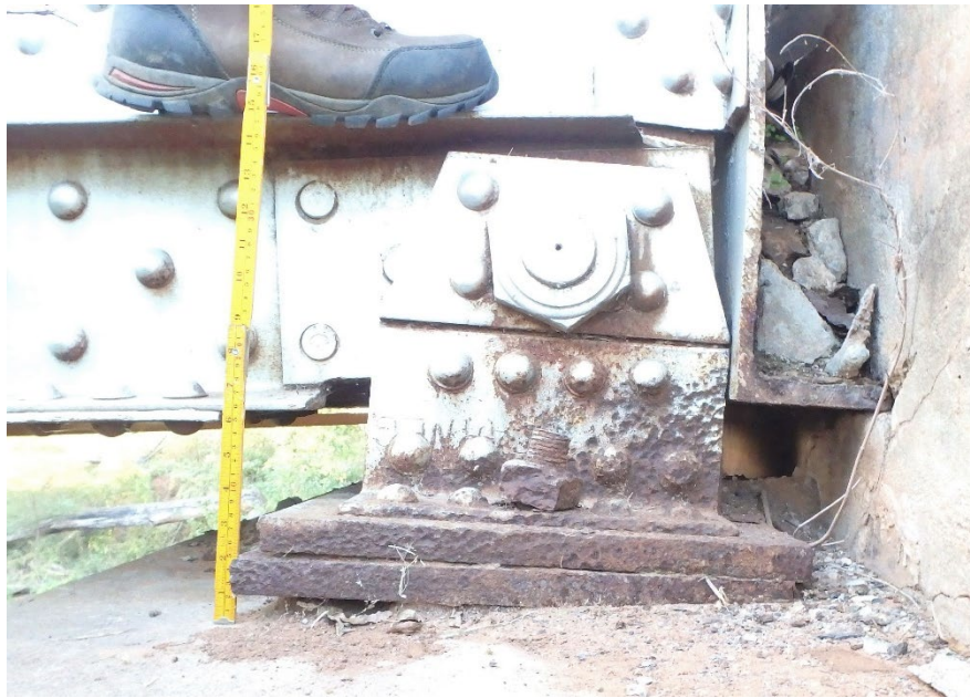
Figure 14.5.8 Bearing Displacement Indicating Possible Movement of Abutment
