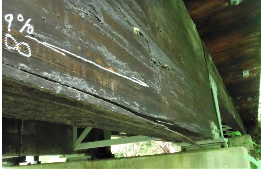
Figure 11.5.4 End of a Laminated Timber Beam Showing Delaminations
