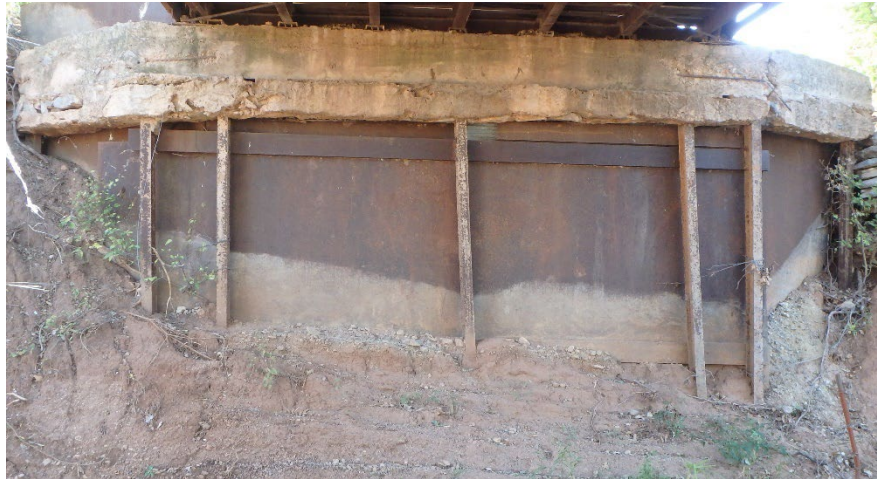
Figure 14.2.58 Stub Abutment on Piles with Piles Exposed
