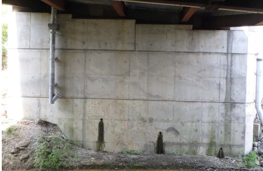
Figure 14.5.24 Abutment with Weep Holes and Staining Underneath
