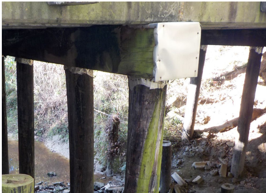
Figure 14.5.23 Timber Bent Cap with Protective Flashing and Decay Due to Drainage
