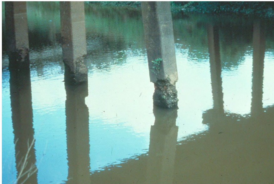
Figure 16.2.11 Concrete Pile Deterioration
