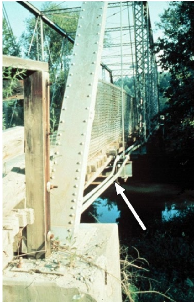
Figure 10.4.48 Buckled Eyebar due to Abutment Movement
