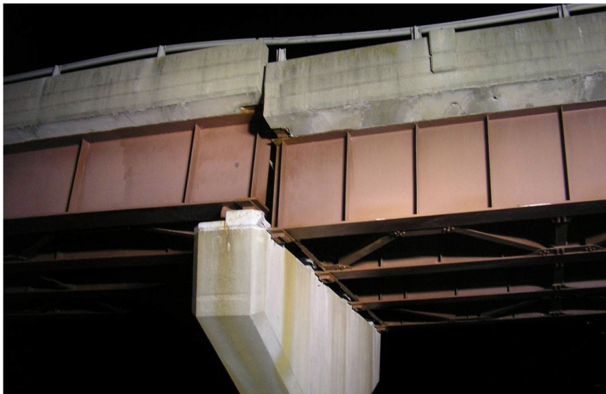
Figure 13.6.10 Dropped Span and Loss of Bearing Area due to Rocker Bearing Failure
