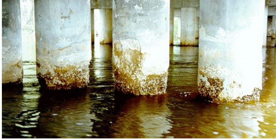
Figure 16.1.35 Pile Bent Deterioration Typically Hidden Underwater
