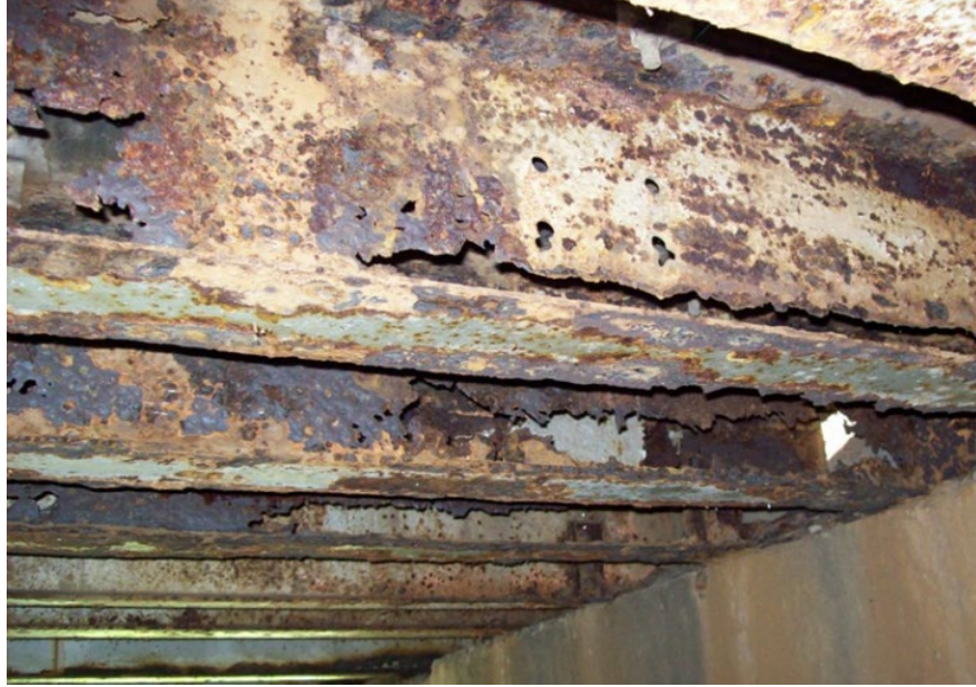
Figure 7.2.10 Steel Corrosion and Complete Section Loss on Girder Webs
