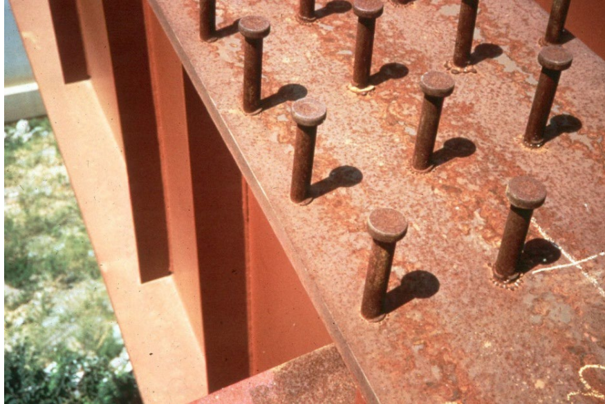
Figure 4.1.32 Shear Studs on Top Flange of Girder (before Concrete Deck is Placed)
