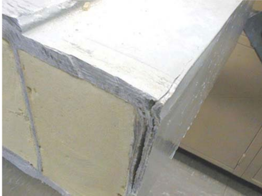
Figure 7.6.13 Voids Resulting in Surface Cracks
