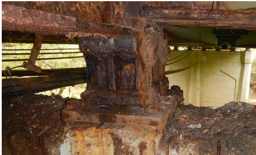
Figure 13.6.2 Heavy Corrosion on a Steel Rocker Bearing
