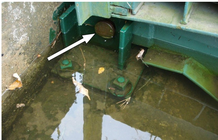
Figure 5.5.3 Fixed Pin Bearing
