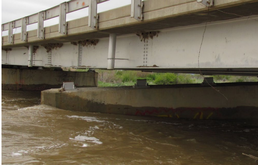
Figure 16.1.3 Pier Settlement due to Undermining
