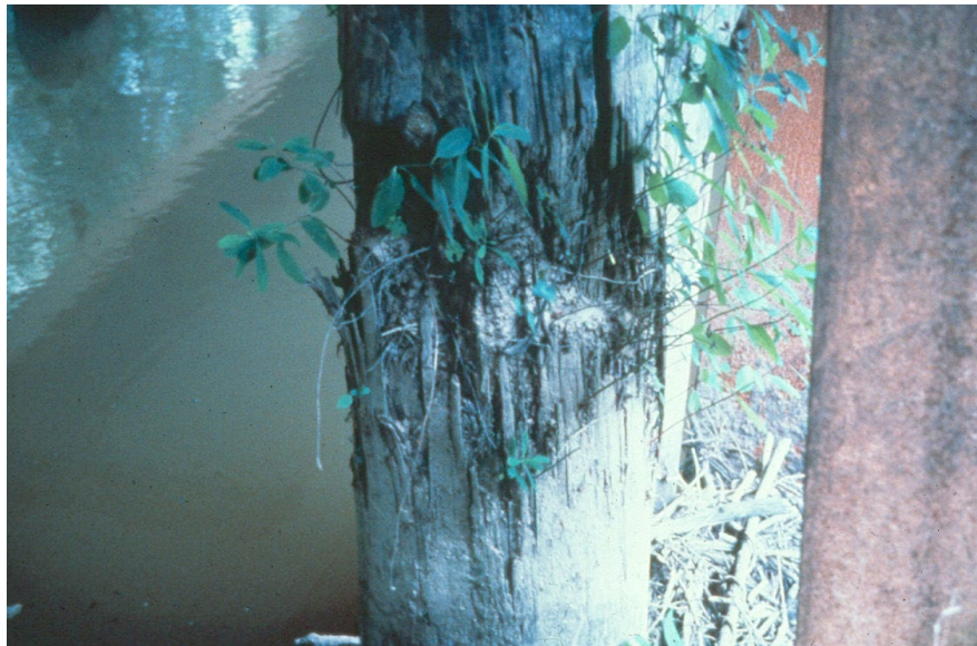
Figure 16.2.12 Timber Pile Deterioration
