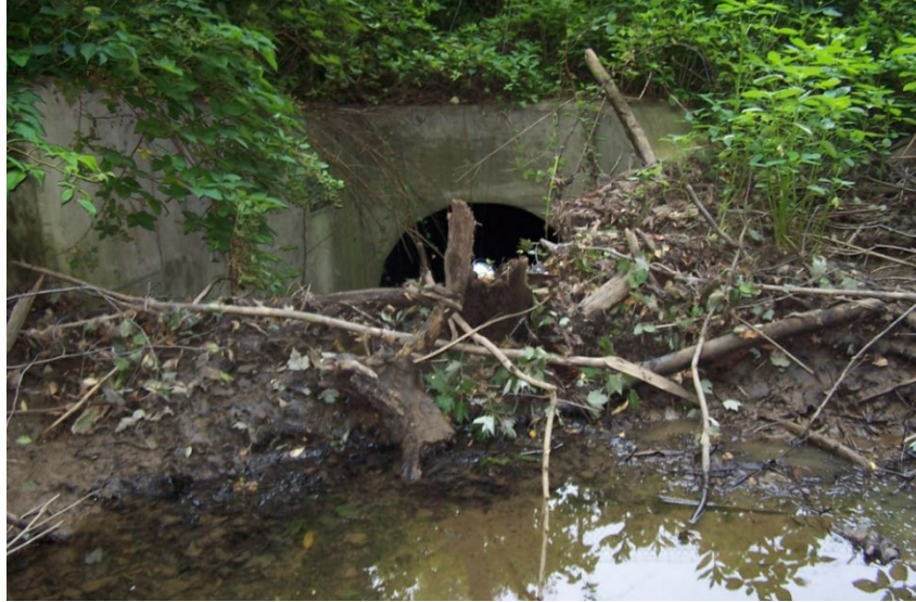
Figure 15.5.23 Debris and Sediment Build-up
