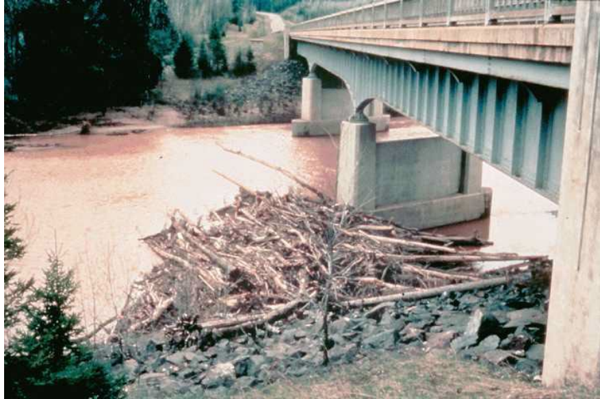
Figure 16.1.12 Debris Build-up in the Waterway
