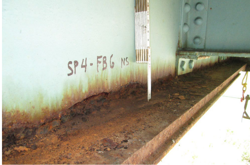
Figure 10.4.19 Corrosion on Top of Floorbeam Bottom Flange
