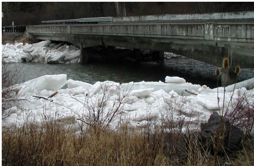
Figure 16.1.11 Ice in Stream Resulting in Possible Contraction Scour
