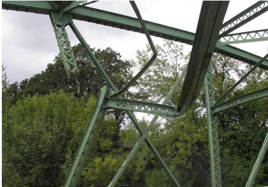
Figure 7.2.13 Collision Damage on a Steel Bridge
