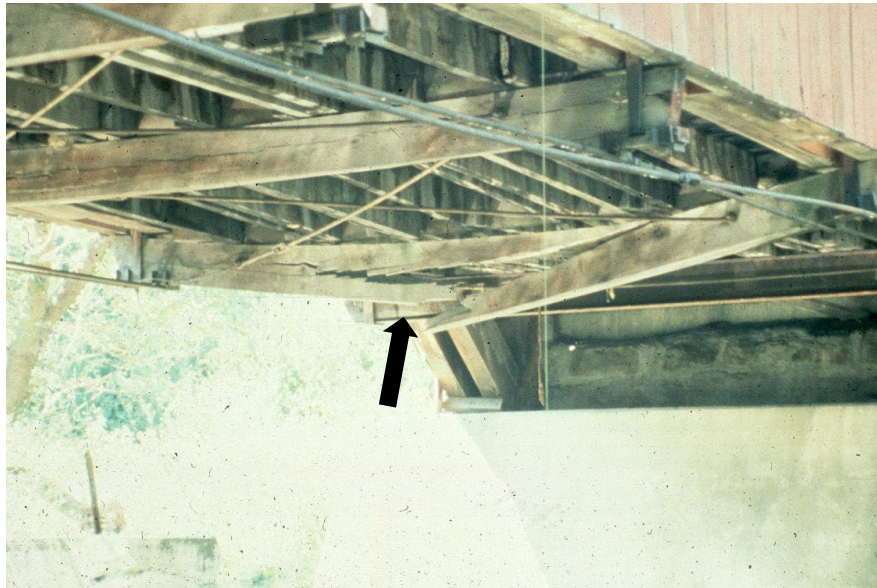
Figure 7.4.24 Failed Timber Floorbeam due to Bending Stress Overload
