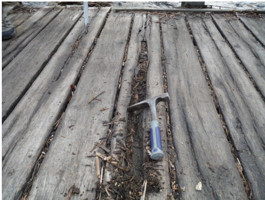
Figure 7.4.26 Weathering on Timber Deck
