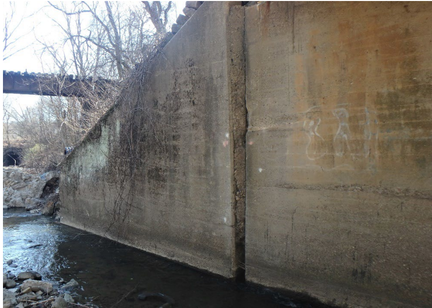
Figure 14.5.16 Rotational Movement of a Concrete Wingwall
