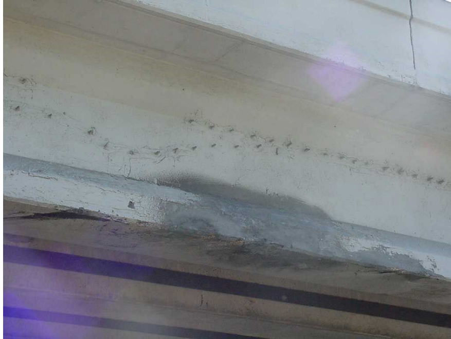
Figure 9.4.45 Collision Damage Repair on Prestressed Concrete I-Beam
