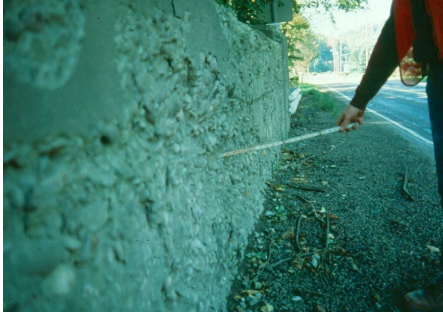
Figure 9.4.32 Interior Face of a Through Girder with Scaling
