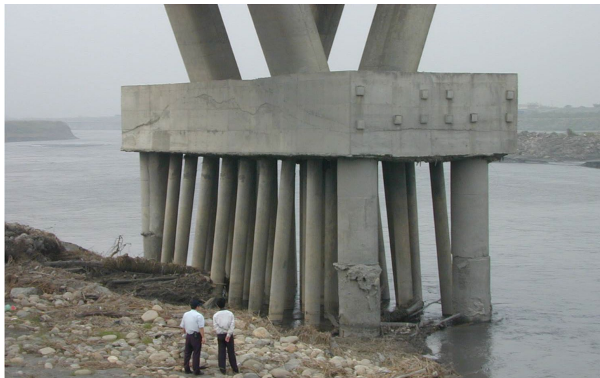
Figure 16.1.16 Pier Foundation Exposed by Scour
