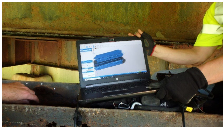
Figure 17.6.6 Laser Scan of Deteriorated Bridge Member
