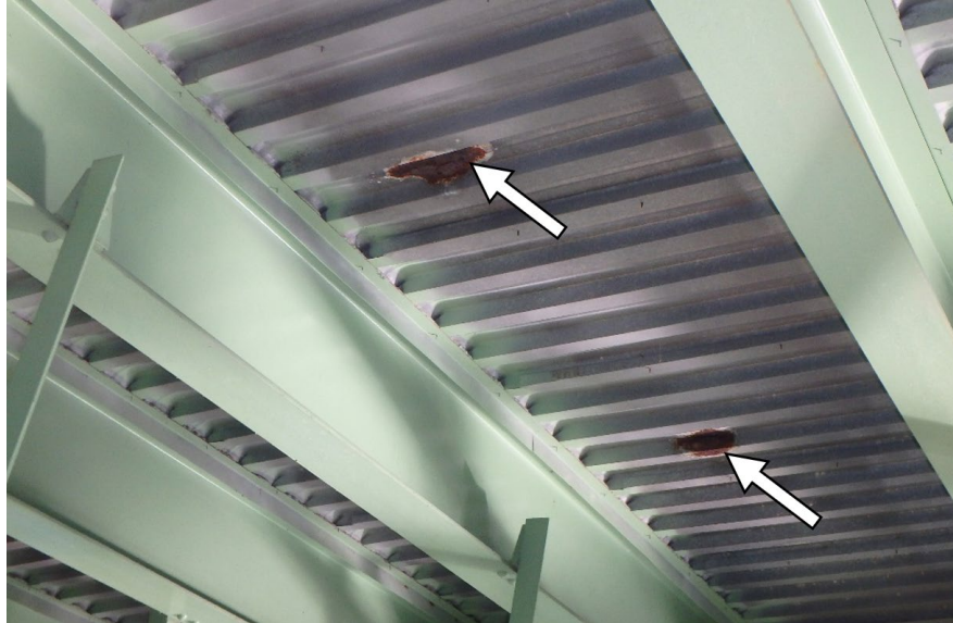
Figure 8.1.9 Stay-in-Place Form with Isolated Rusting
