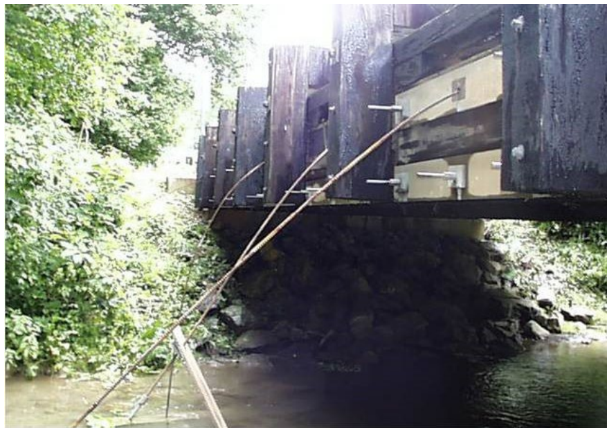
Figure 8.3.11 Failed Post-Tensioning Tendons
