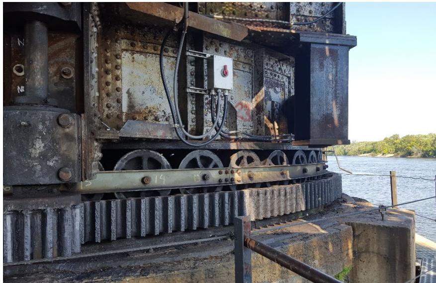
Figure 5.3.5 Rim-Bearing Swing Span Rollers
