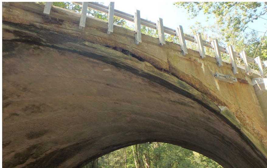
Figure 9.4.24 Deteriorated Arch/Spandrel Wall Interface
