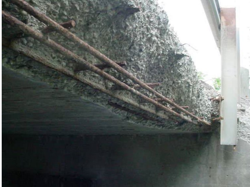
Figure 7.1.34 Corroded Reinforcing Bars with Severely Spalled Concrete
