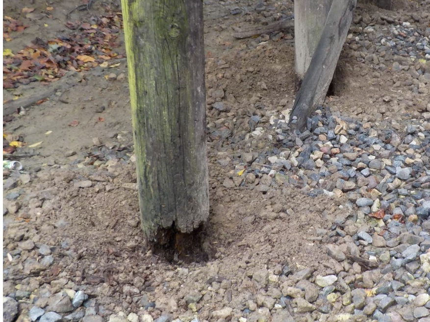
Figure 14.5.35 Timber Bent Column Decay at Ground Line
