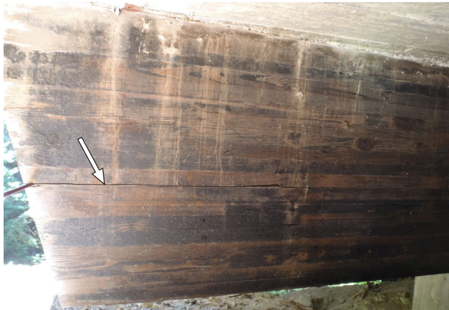
Figure 11.5.3 Glulam Floorbeam Showing with Delamination
