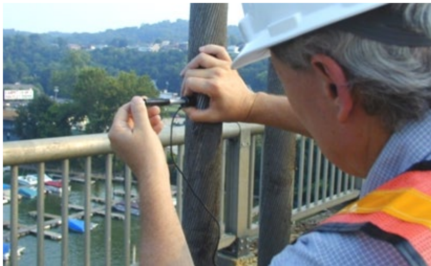
Figure 10.4.16 Hardness Test on Fire Damaged Arch Cables
