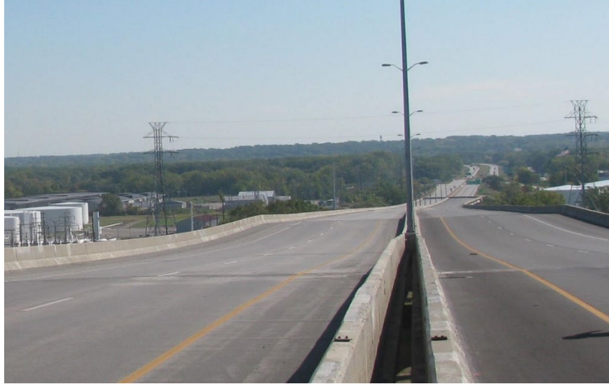
Figure 14.5.6 Deck and Railing Evidence of Pier Settlement
