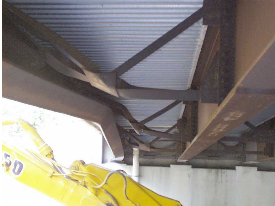
Figure 7.3.27 Severe Collision Damage on a Fascia Girder
