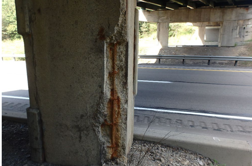
Figure 14.5.22 Concrete Spalling on Concrete Column
