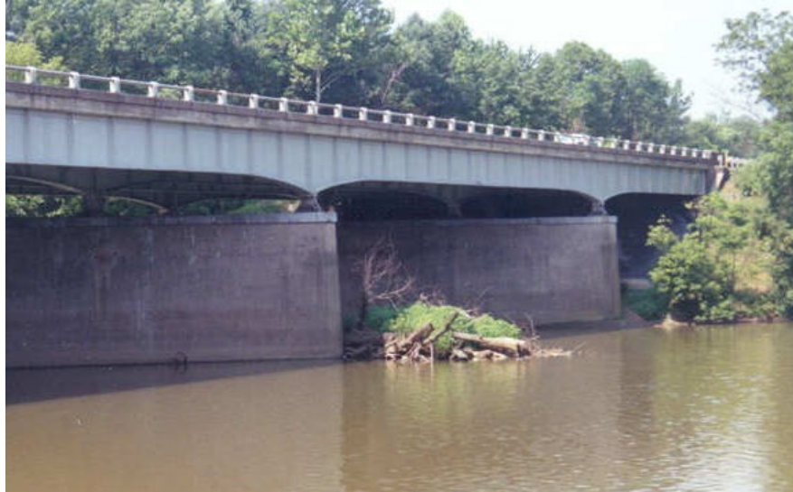
Figure 16.2.9 Buildup of Debris at Pier
