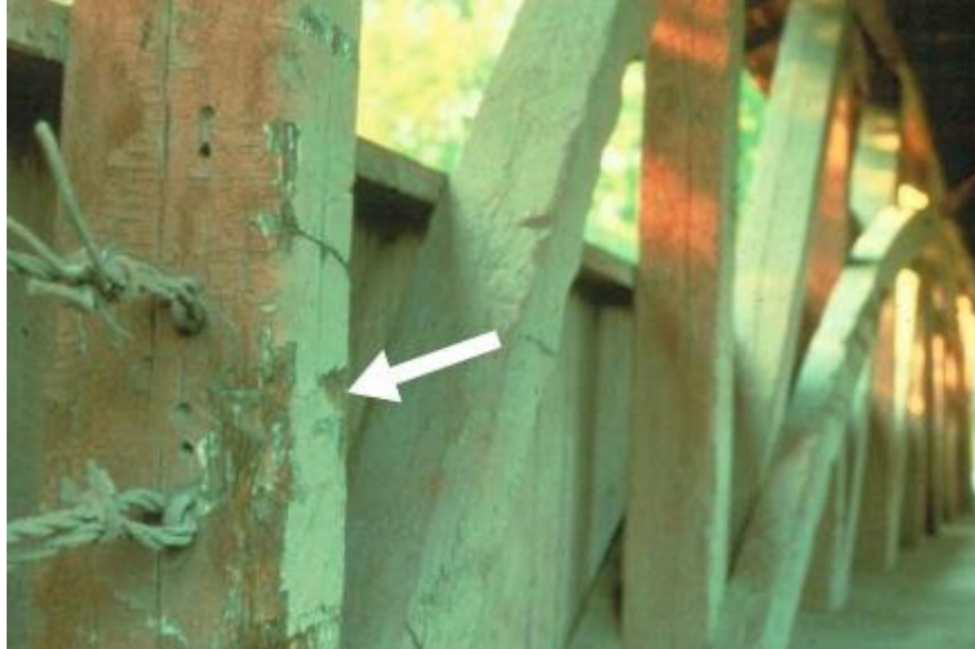
Figure 7.4.21 Impact/Collision Damage to a Timber Member
