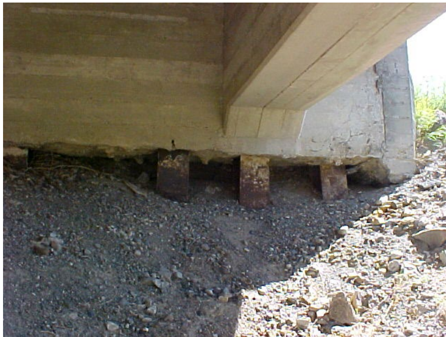
Figure 16.1.55 Exposed Piling Due to Scour
