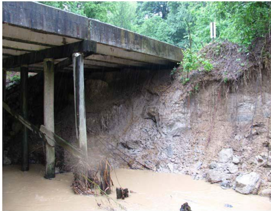
Figure 16.1.17 Lateral Stream Migration Endangering an Abutment
