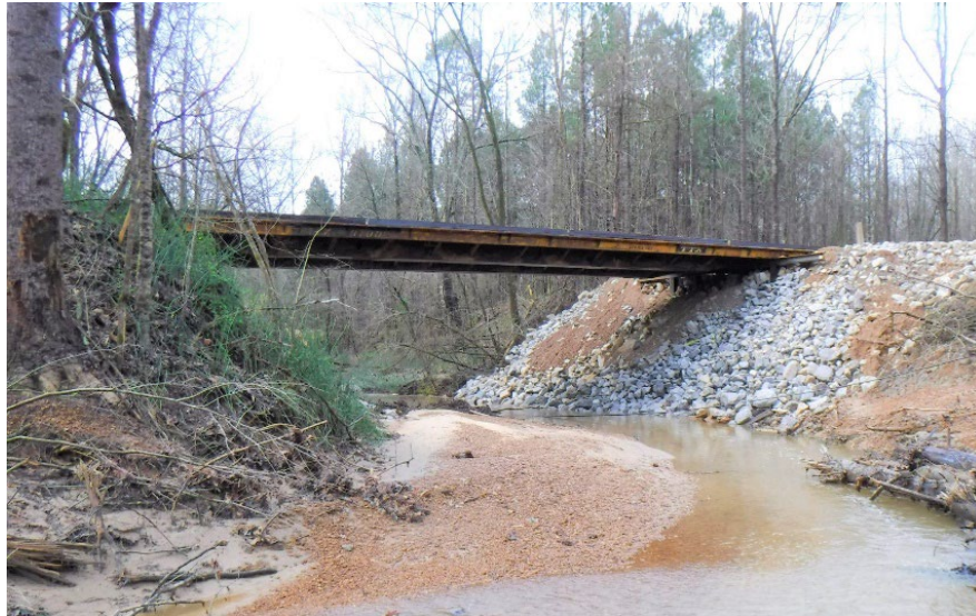
Figure 10.1.114 Railroad Car Converted Bridge without Bridge Railing
