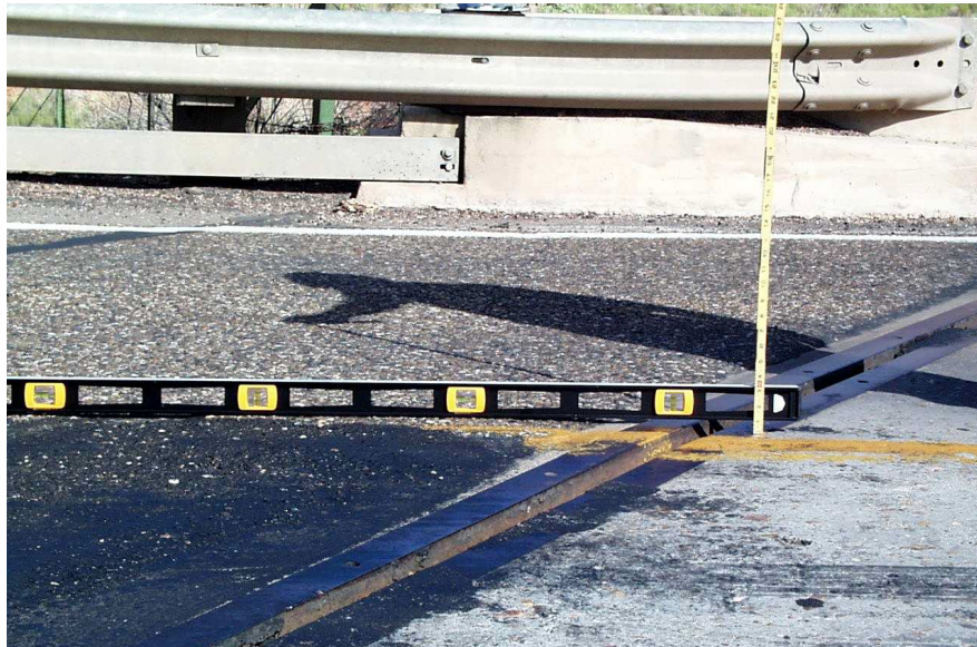
Figure 14.5.10 Vertical Misalignment Between Approach Slab and Bridge Deck
