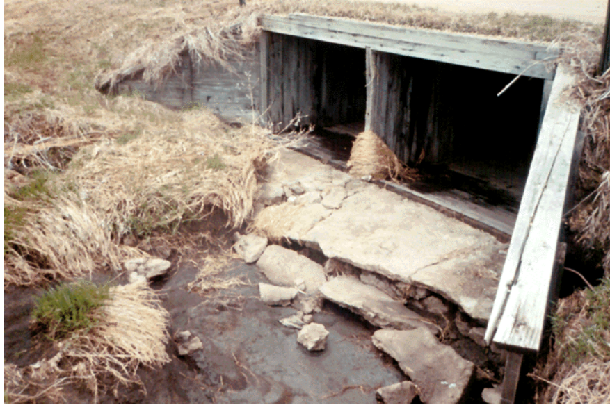
Figure 15.5.10 Scour and Undermining at Culvert Inlet
