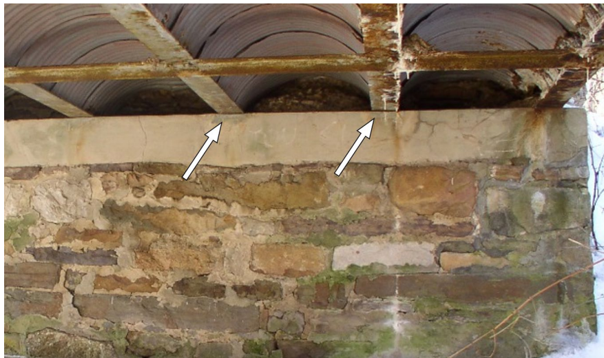
Figure 14.5.18 Cracking in Bearing Seat of Concrete and Stone Abutment
