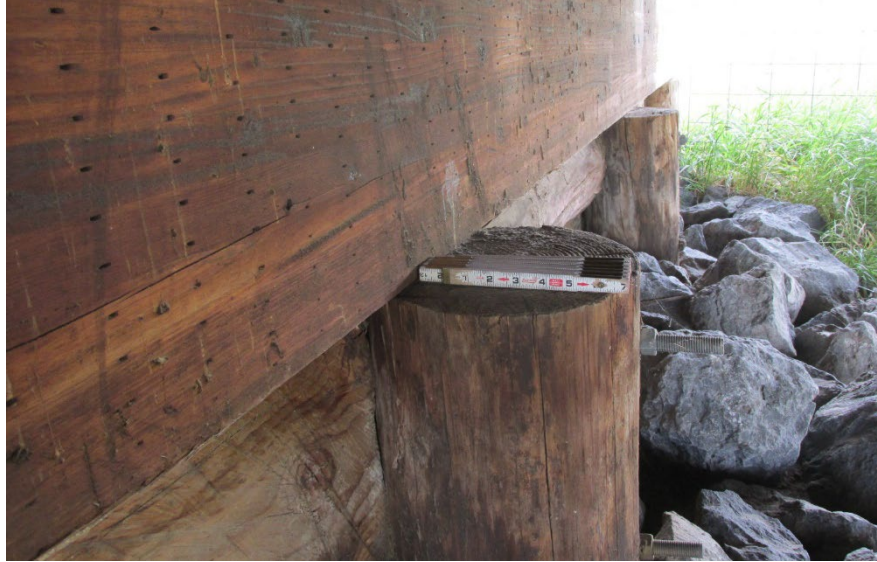
Figure 14.5.9 Local Failure in Timber Pile/Abutment Seat Interface Indicating Possible Movement of Abutment
