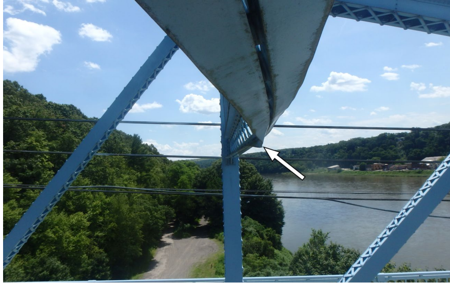
Figure 10.1.119 Truss Bridge Sway Bracing with Collision Damage
