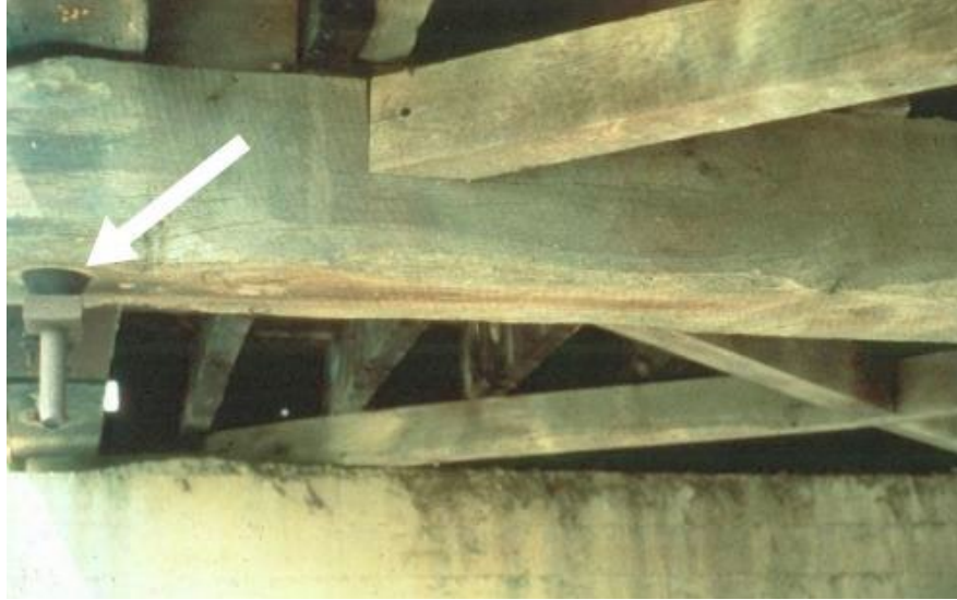
Figure 7.4.19 Loose Hanger Connection Between the Timber Truss and Floorbeam
