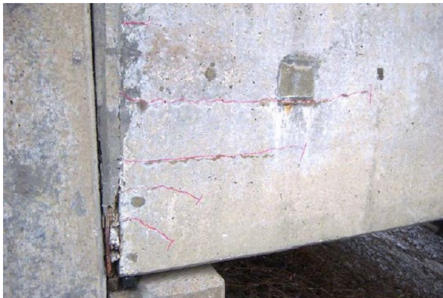
Figure 9.4.6 Bearing Area: Longitudinal Cracks in Web of Box Beam
