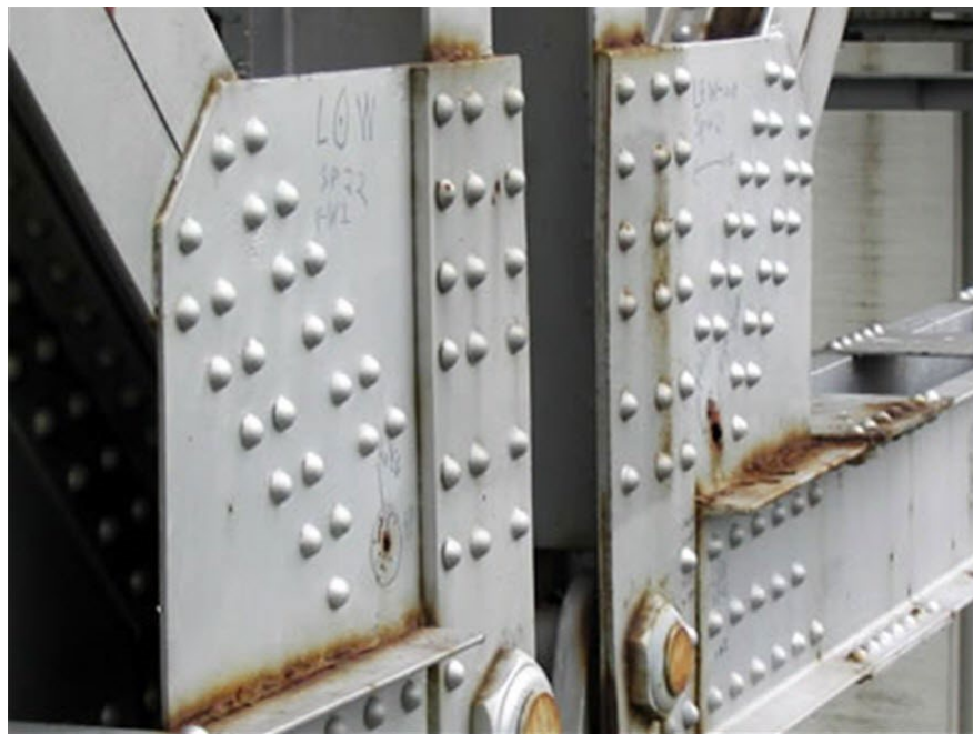
Figure 10.4.36 General Corrosion of Gusset Plates
