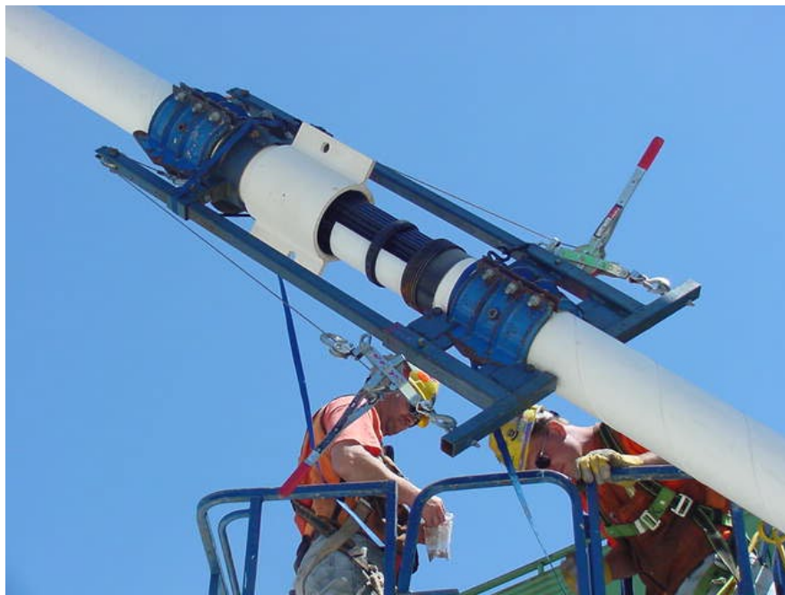
Figure 5.2.34 Anti-Rattling Device Installed on Cable
