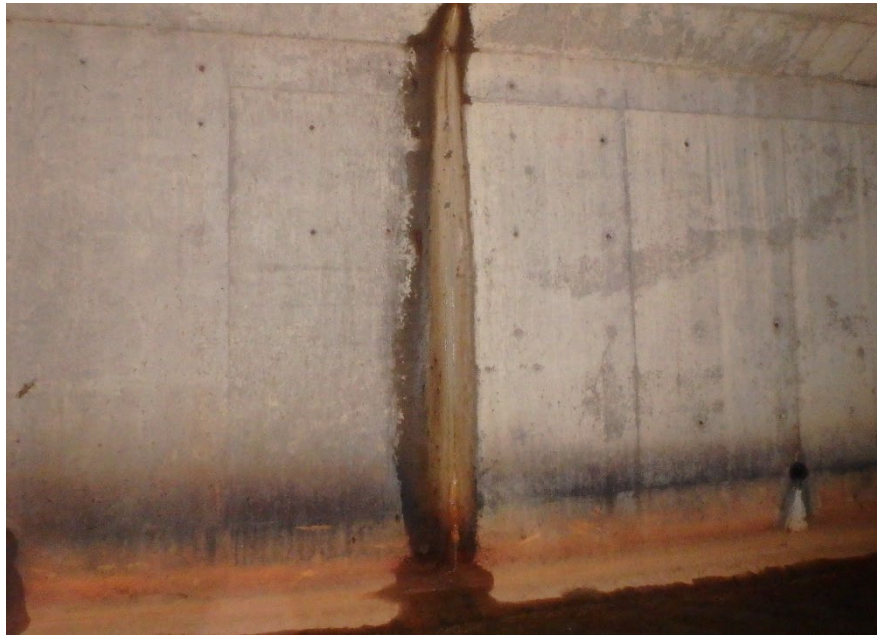
Figure 15.5.11 Precast Concrete Box Culvert Joint with Infiltration
