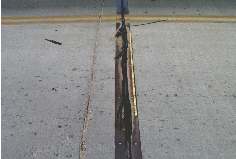
Figure 8.5.28 Failed Compression Seal
