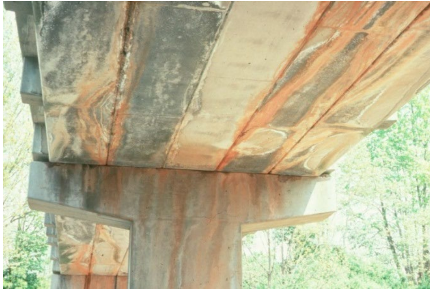
Figure 9.4.40 Joint Leakage and Rust Staining
