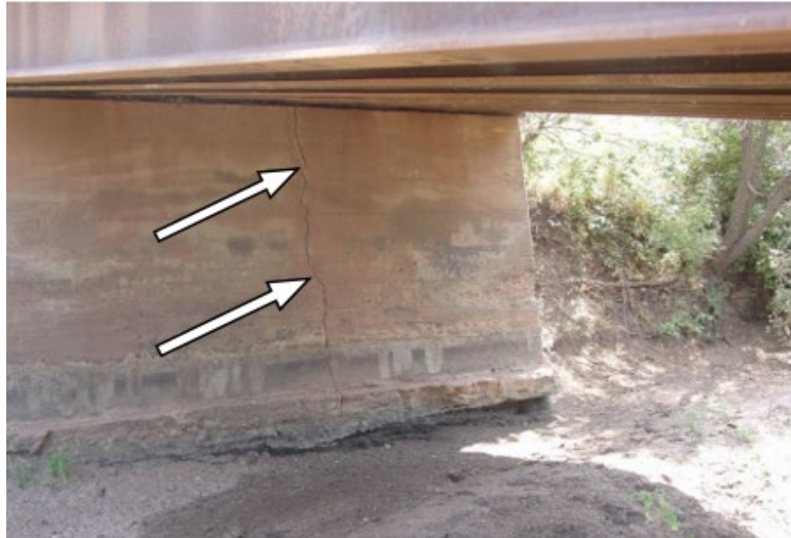
Figure 14.5.5 Crack in Abutment due to Differential Settlement
