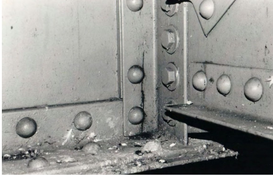
Figure 10.4.24 Crack in Angle at Floorbeam-Stringer Connection
