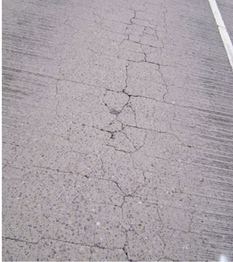
Figure 7.1.18 Pattern or Map Cracks
