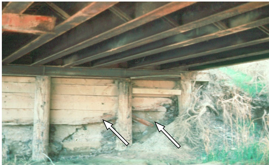
Figure 14.5.31 Decayed Timber Lagging and Abrasion Exposed by Scour
