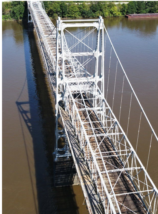
Figure 5.2.22 Steel Portal Tower
