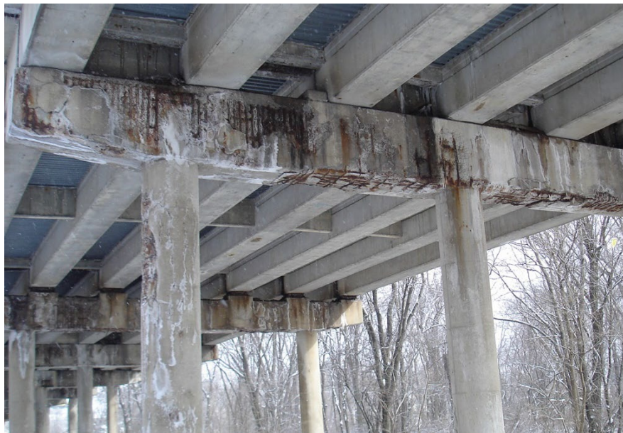
Figure 14.5.21 Widespread Concrete Spalling on Bent Cap due to Drainage
