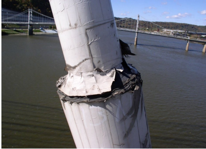
Figure 12.2.6 Deteriorated Cable Wrapping Allowing Water Penetration into Sheath
