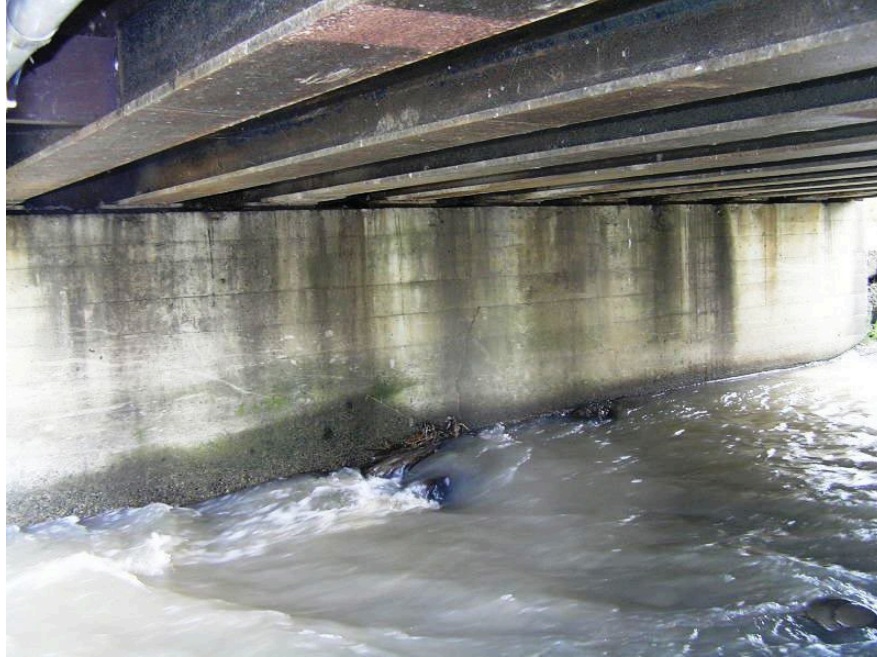
Figure 16.1.56 Accelerated Flow Due to Constricted Waterway
