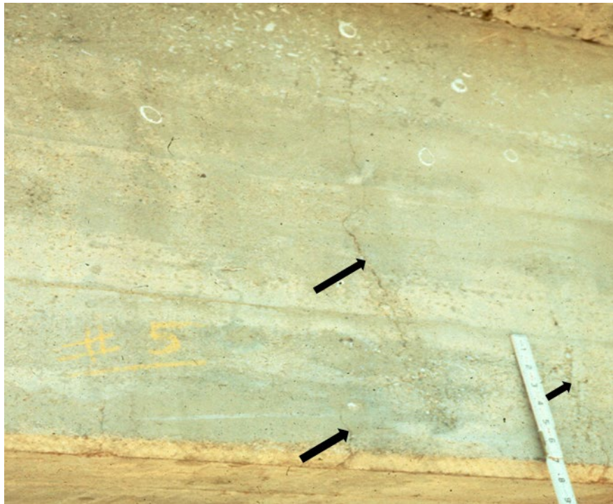
Figure 7.1.11 Flexural Cracks on a Tee Beam
