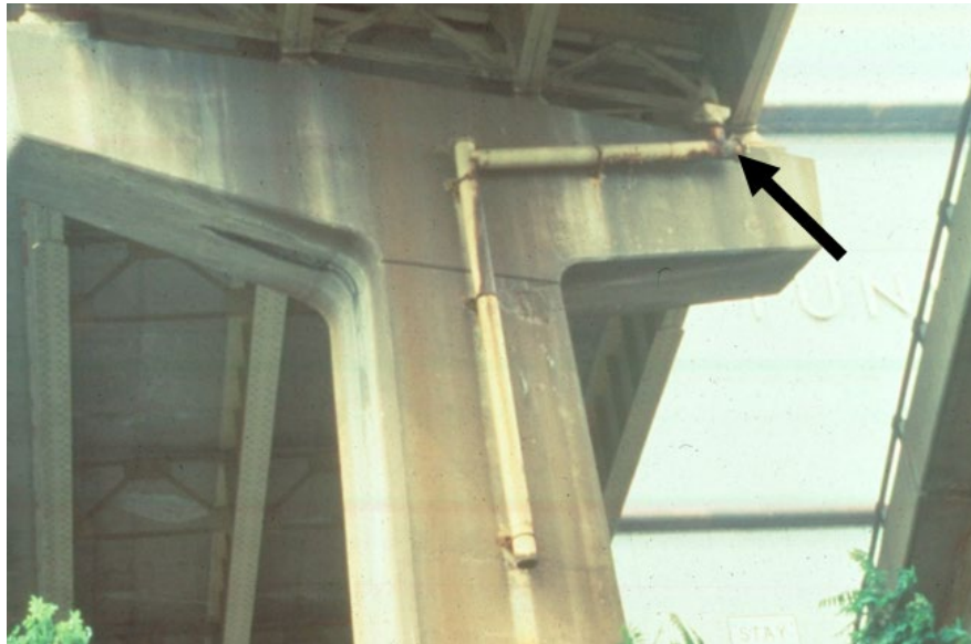
Figure 8.5.32 Damaged Outlet Pipe with Cleanout Plug
