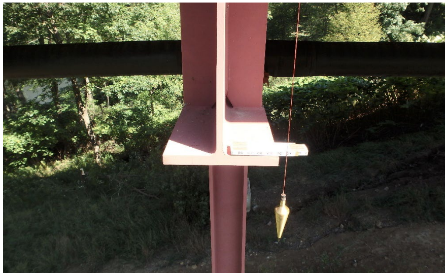
Figure 16.1.36 Out of Plumb Bent
