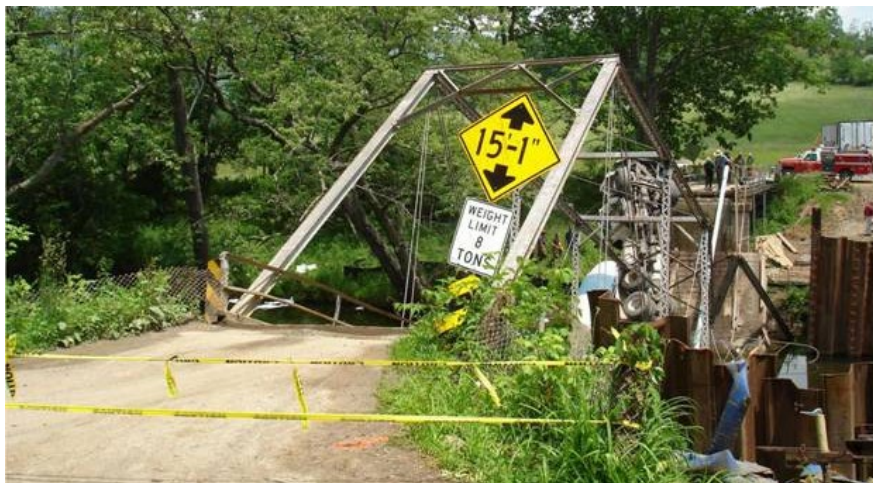
Figure 6.2.23 Damaged Bridge Due to Failure to Comply with Bridge Posting
