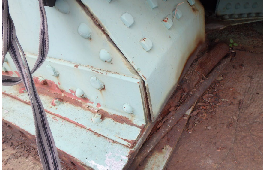
Figure 13.6.6 Damaged Roller Nest Bearing
