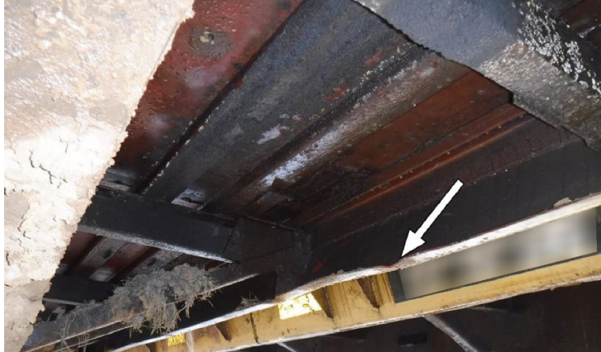
Figure 10.4.57 Existing Distortion to Channel Beam
