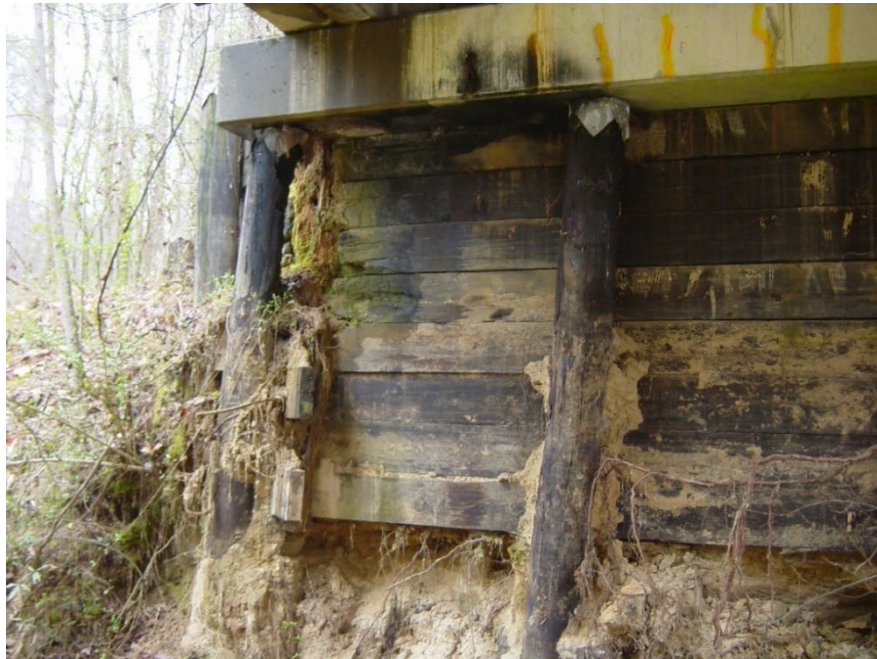
Figure 16.1.48 Bridge Abutment Affected by Scour
