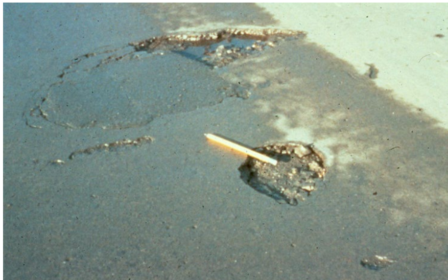
Figure 7.1.24 Spalling on a Concrete Deck
