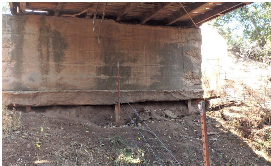
Figure 14.5.12 Erosion at Abutment Exposing Piles
