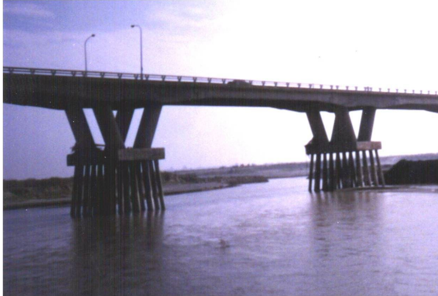
Figure 16.1.15 Micro-piles Exposed by Scour
