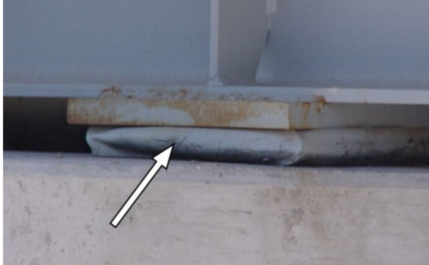
Figure 13.6.13 Neoprene Bearing Pad Excessive Bulging and Splitting
