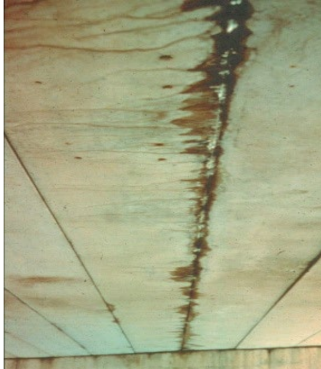
Figure 9.4.13 Shear Key Leaking Joint Between Adjacent Box Beams
