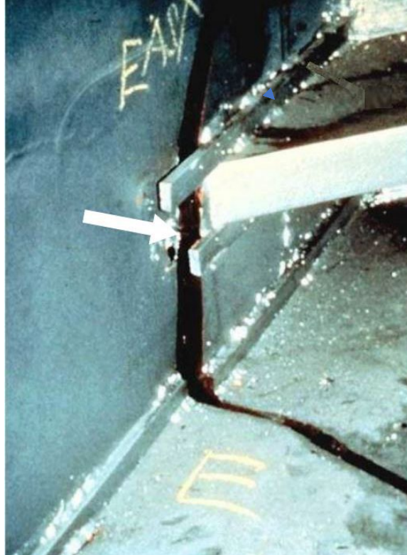
Figure 7.3.39 Poor Quality Welds Inside Cracked Cross Girder
