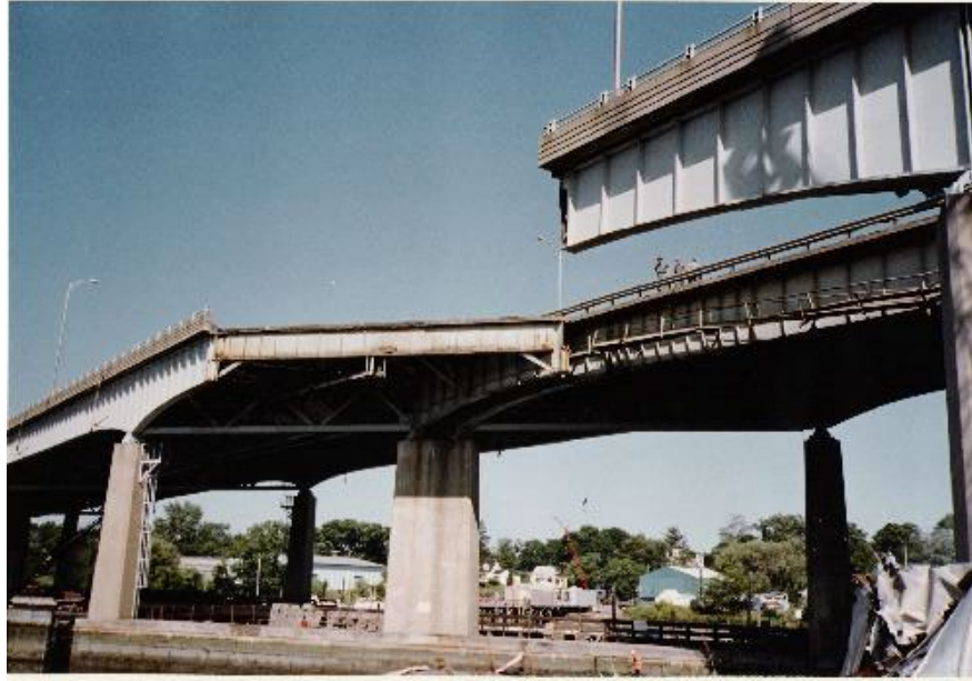
Figure 10.5.3 Mianus River Bridge Failure - From Ground
