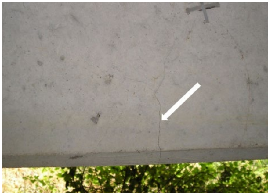
Figure 9.4.18 Flexure Cracks on a Tee Beam Stem
