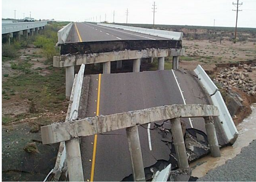
Figure 14.5.13 Pier Movement and Superstructure Damage due to Scour/Undermining
