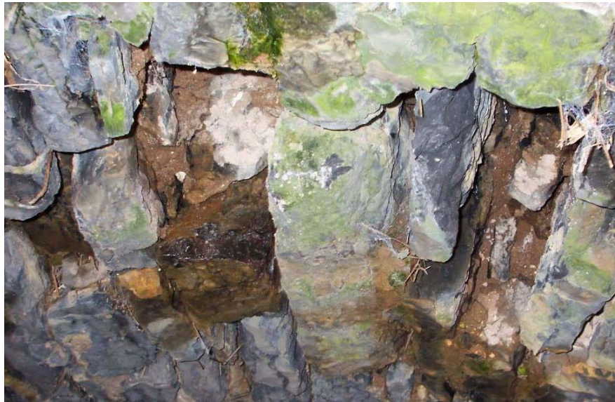
Figure 15.5.8 Drainage Through Missing Stones in Masonry Culvert
