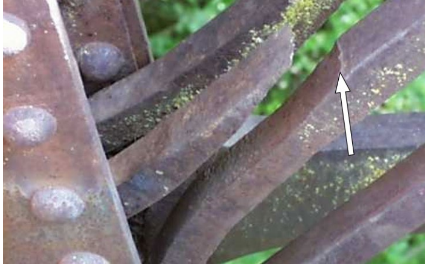
Figure 10.4.46 Cracked Forge Zone on a Loop Rod
