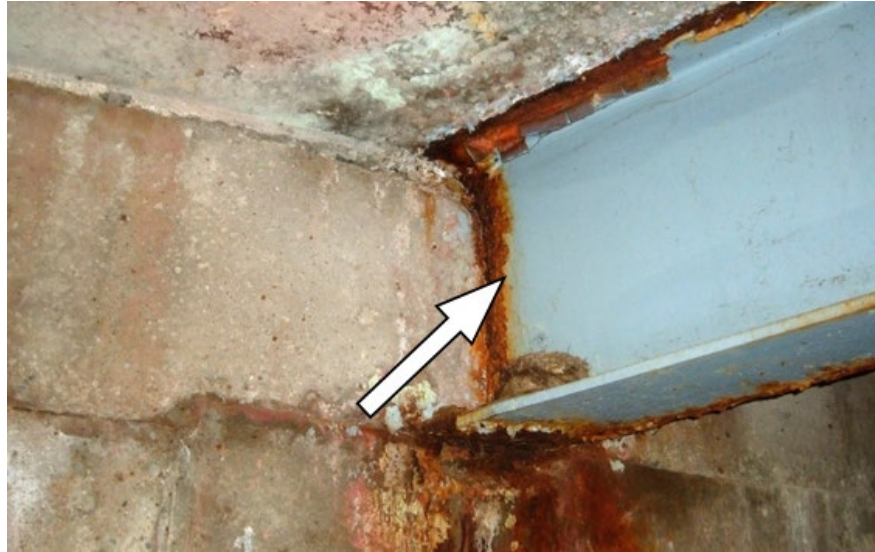
Figure 10.4.2 Corroded Shear Zone on a Rolled Beam Bridge
