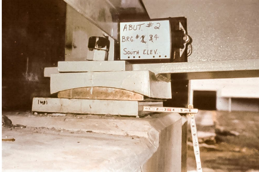
Figure 13.6.5 Longitudinal Misalignment in Bronze Sliding Plate Bearing
