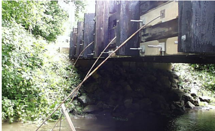
Figure 11.5.9 Broken Stressing Rods
