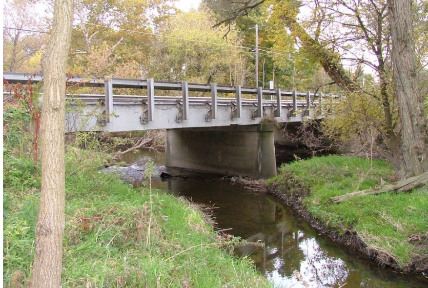
Figure 16.1.42 Sediment Accumulation Redirecting Streamflow
