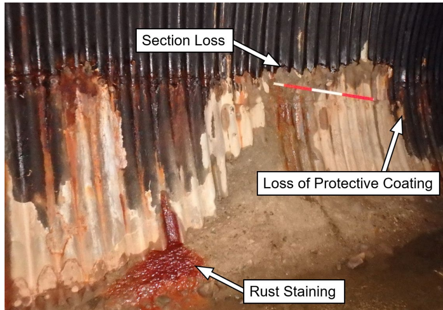
Figure 15.4.1 Advanced Deterioration of a Flexible Culvert Section
