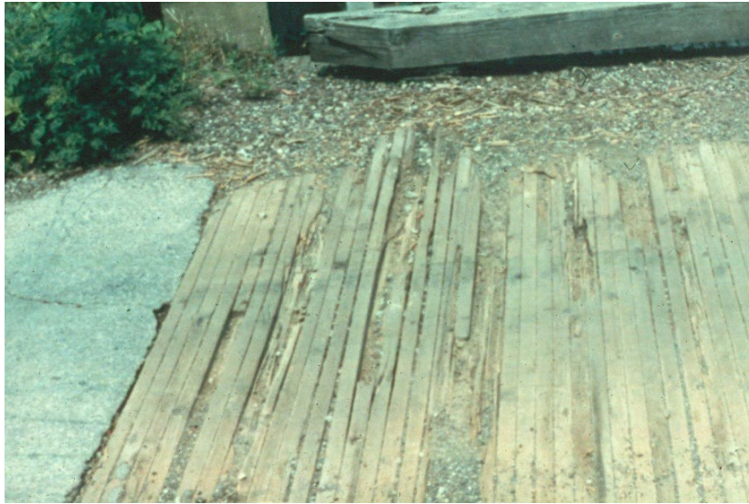
Figure 8.3.8 Wear and Weathering on a Timber Deck
