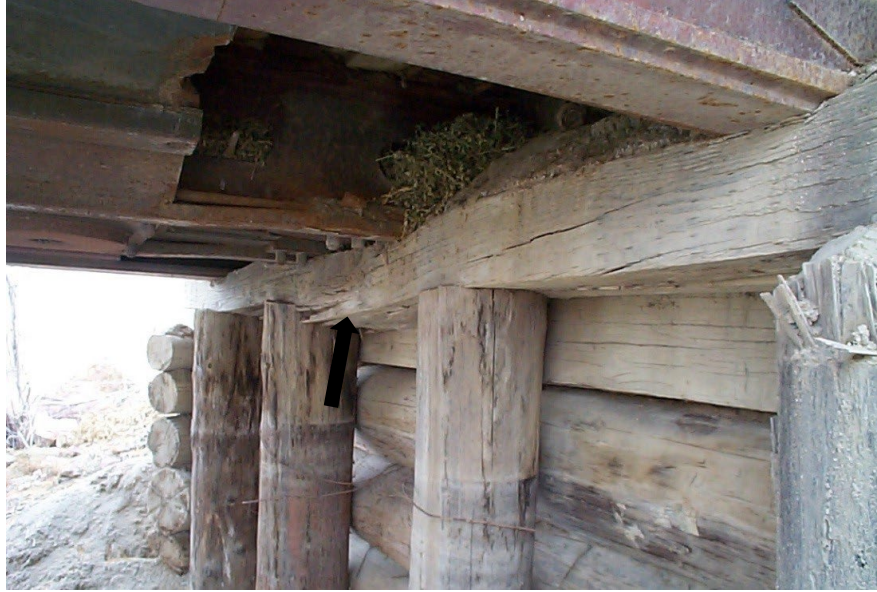
Figure 7.4.25 Decayed Timber Member Subjected to Crushing and Overstress
