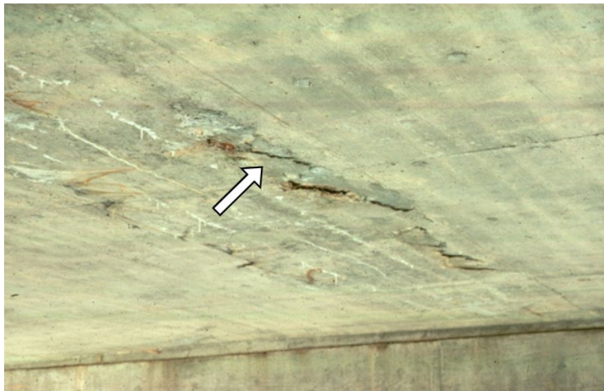
Figure 9.4.22 Slab Max. Moment Area: Delamination, Efflorescence, Rust Stains
