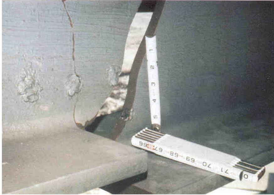
Figure 7.3.21 Crack Resulting from Plug Welded Holes
