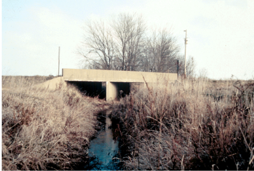
Figure 16.1.10 Vegetation Constricting the Waterway
