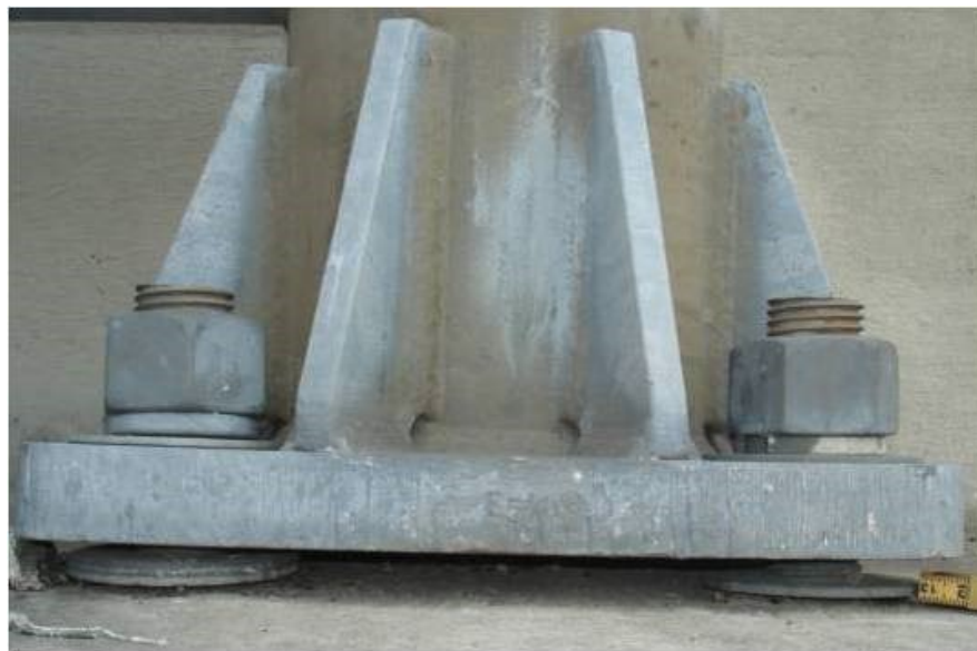
Figure 8.5.35 Sign Attachment Exhibiting Anchor Pullout
