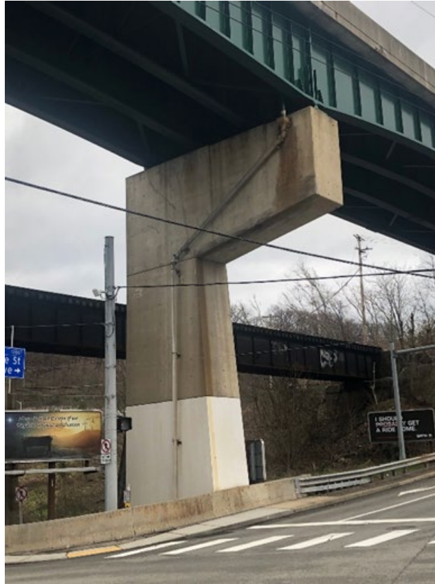
Figure 4.1.3 Unusual Concrete Shapes
