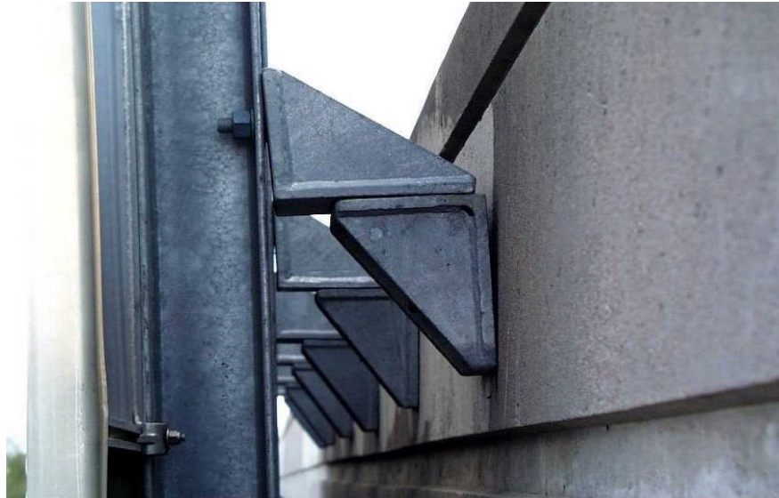
Figure 8.5.36 Sign Mount with Loose Adhesive Anchorage
