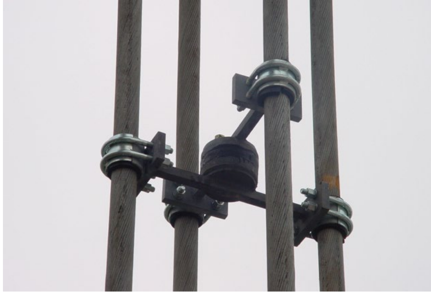
Figure 5.2.20 Cable Damper System
