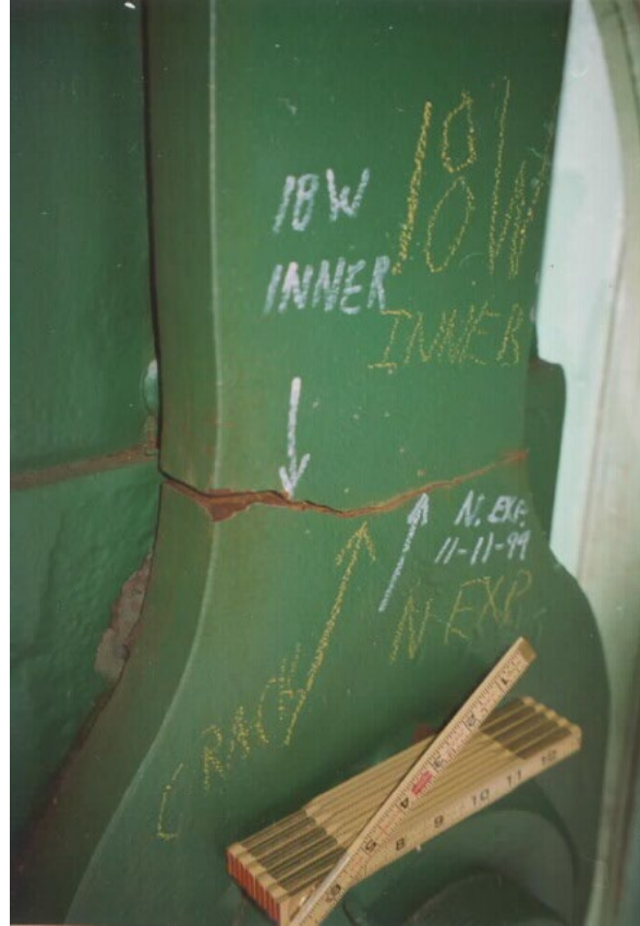
Figure 10.4.31 Cracked Forge Zone on an Eyebar
