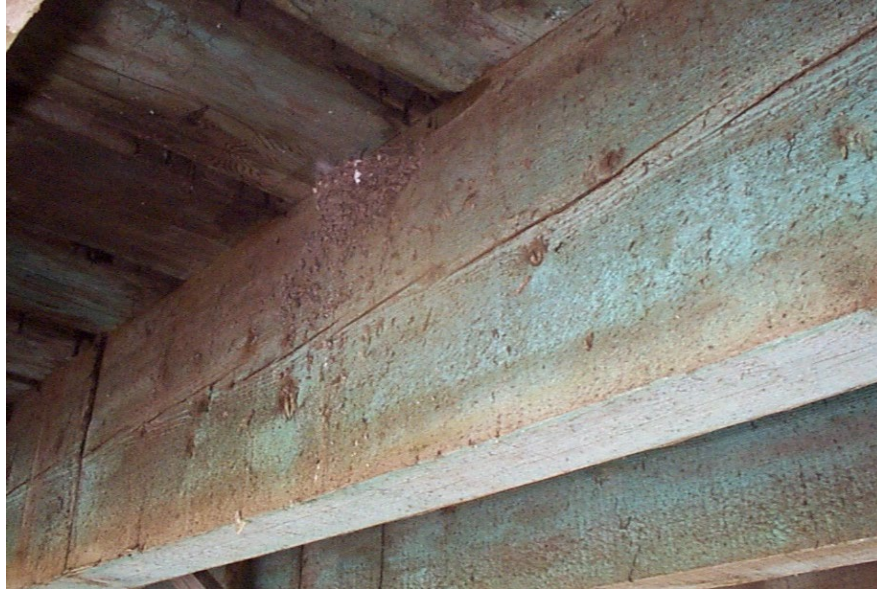
Figure 7.4.23 Horizontal Shear Failure in Timber Member
