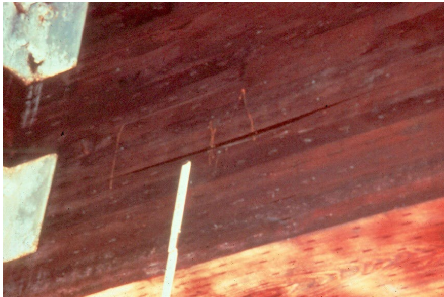
Figure 7.4.18 Delamination in a Glue Laminated Timber Member
