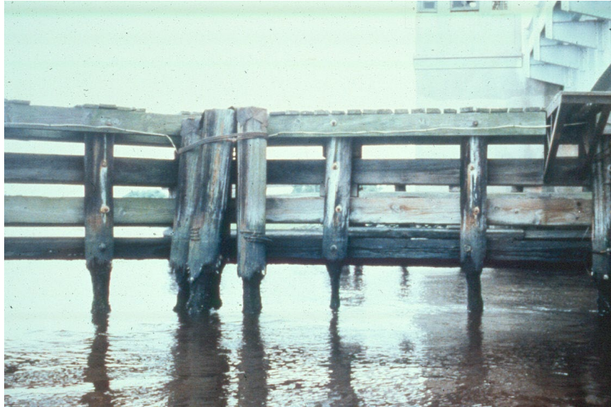
Figure 14.5.32 Timber Fender System with Deteriorated Piles
