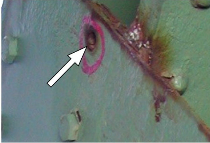
Figure 10.4.45 Missing Bolts on a Gusset Plate
