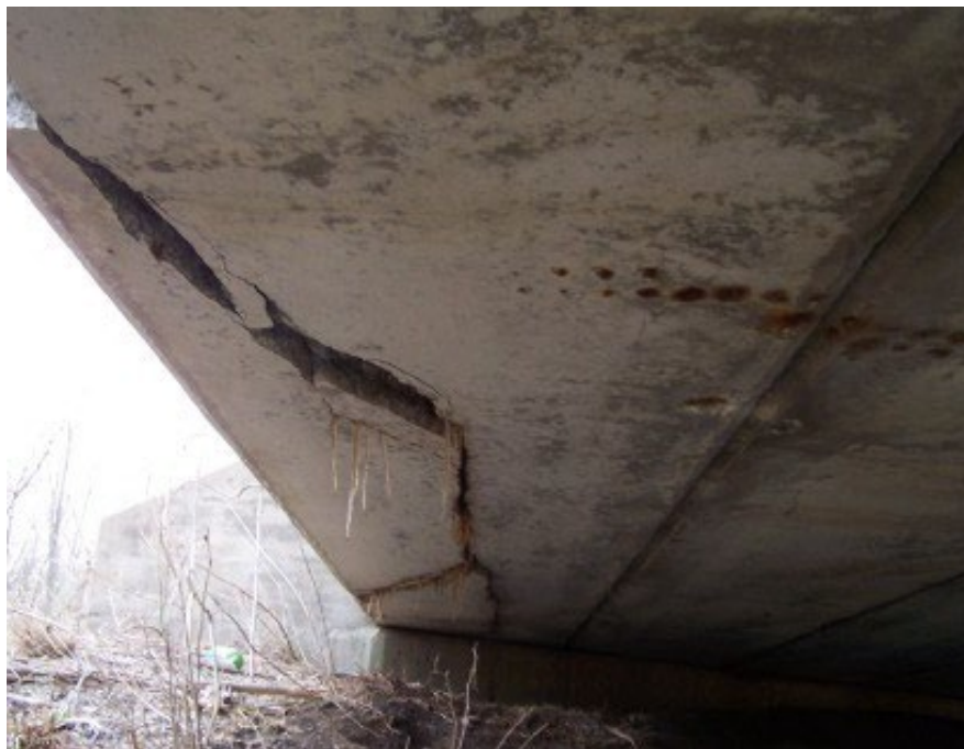
Figure 9.4.44 Box Beam Damage Caused by Vehicle Striking Attached Railing
