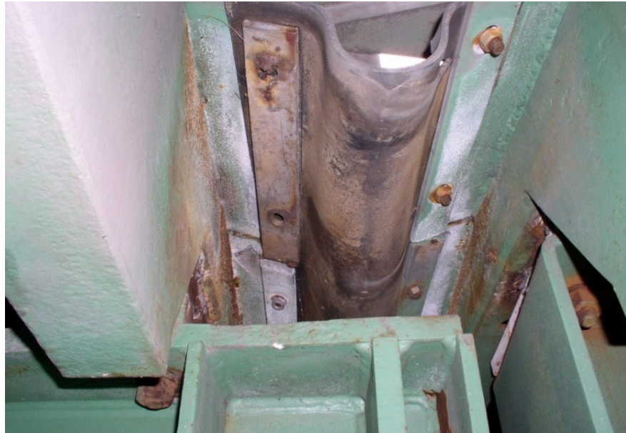
Figure 8.5.23 Drainage Trough with Missing Bolts
