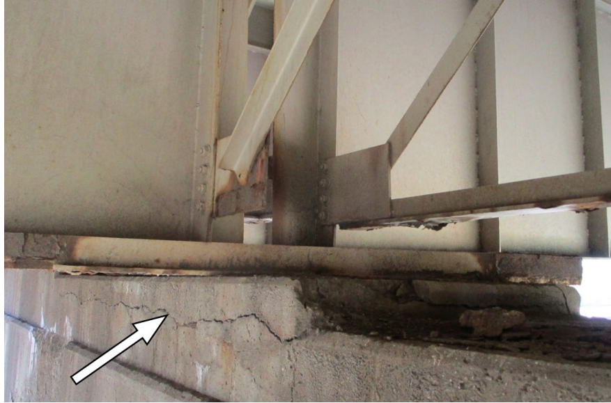
Figure 14.5.17 Crack in Concrete Pedestal at Bearing Location
