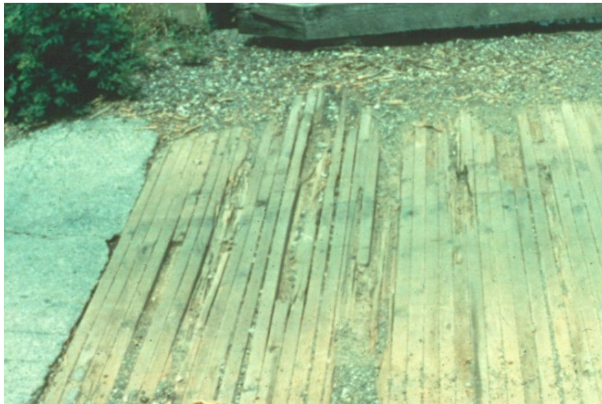
Figure 7.4.22 Wear of a Nail-Laminated Timber Deck
