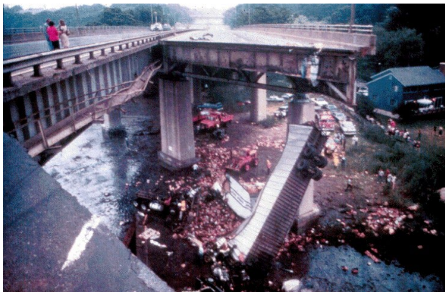
Figure 7.3.2 Mianus River Bridge Collapse
