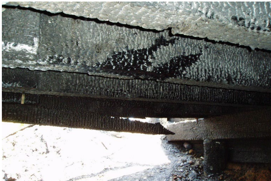
Figure 7.4.20 Fire Damaged Timber Members
