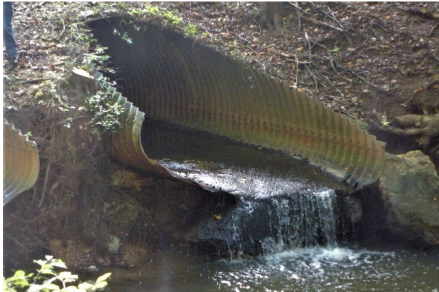
Figure 15.5.22 Unsupported Mitered Culvert End
