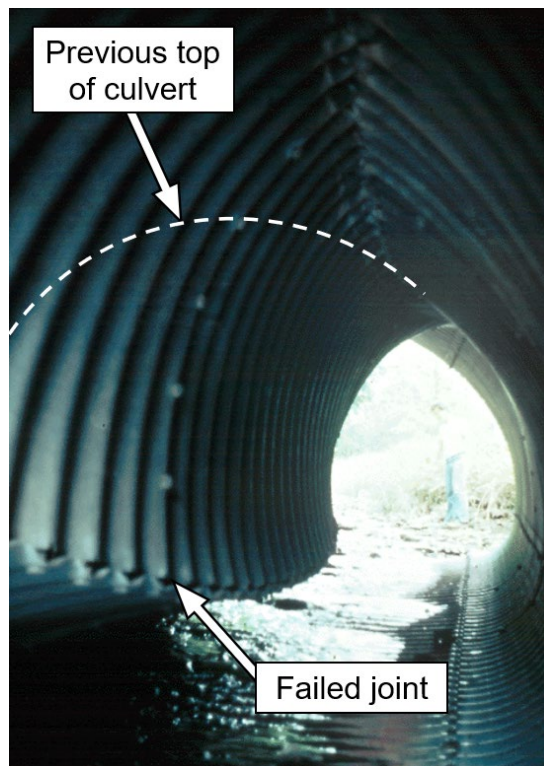
Figure 15.5.7 Flexible Pipe Culvert Bending Failure
