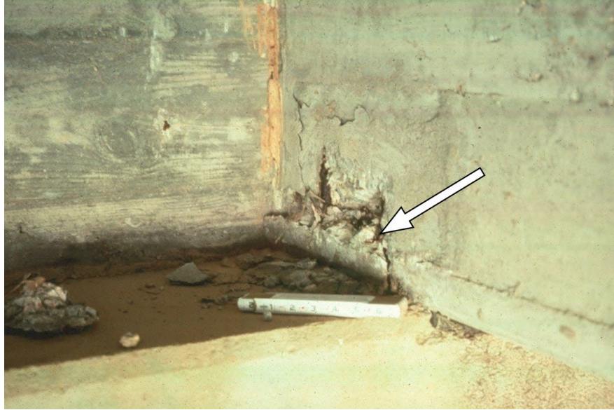
Figure 9.4.3 Bearing Area: Spalling and Exposed Tee Beam Reinforcement
