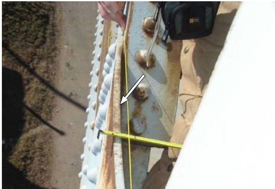
Figure 10.4.44 Gusset Plate Out-of-Plane Distortion
