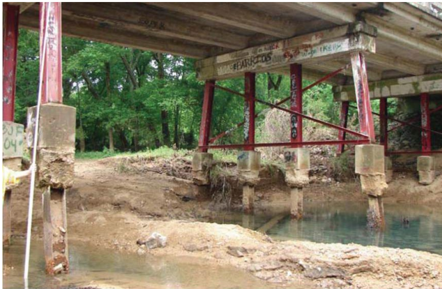
Figure 16.1.40 Severe Streambed Scour Evident at Low Water Flow
