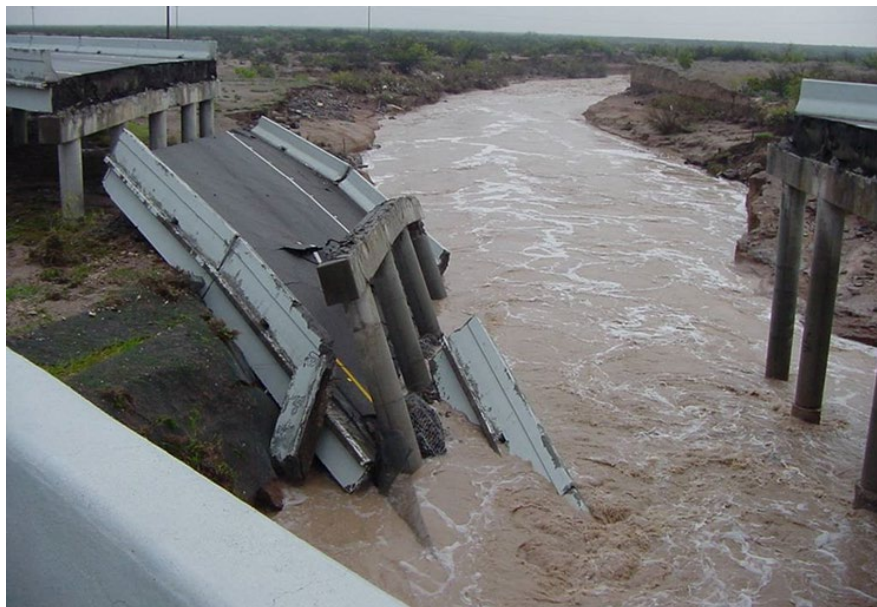
Figure 4.3.3 Pier Foundation Failure
