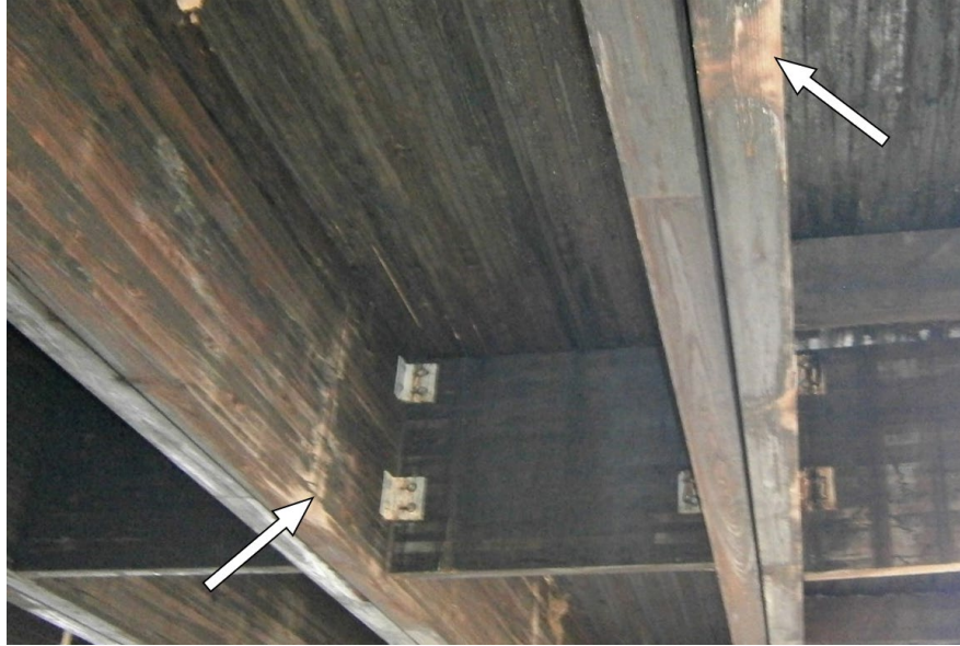
Figure 11.5.6 Decay on Glulam Beam
