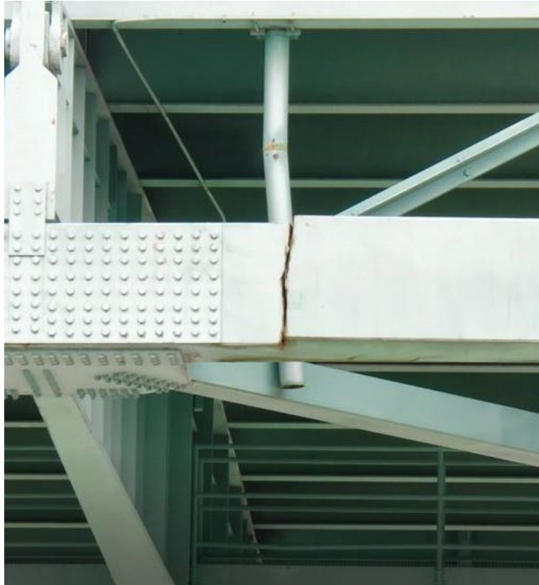
Figure 10.5.11 I-40 Hernando DeSoto Bridge Fracture
