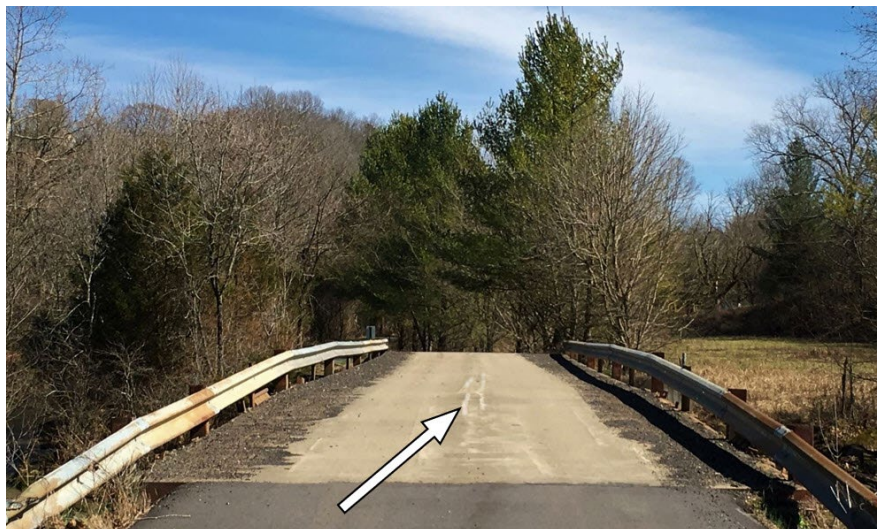
Figure 10.4.58 Railroad Car Converted Bridge Deck with Cracking
