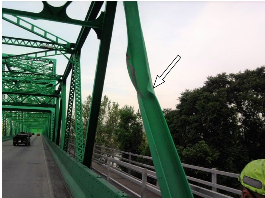
Figure 10.4.17 Buckled End Post
