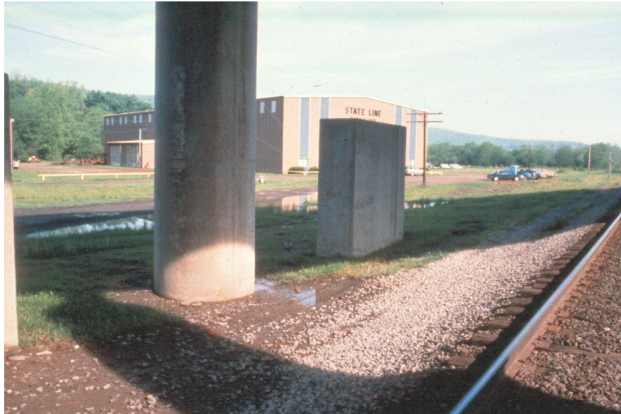
Figure 14.2.62 Concrete Collision Protection Block
