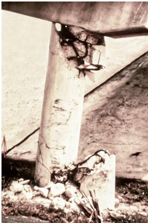
Figure 7.1.31 Concrete Column Collision Damage
