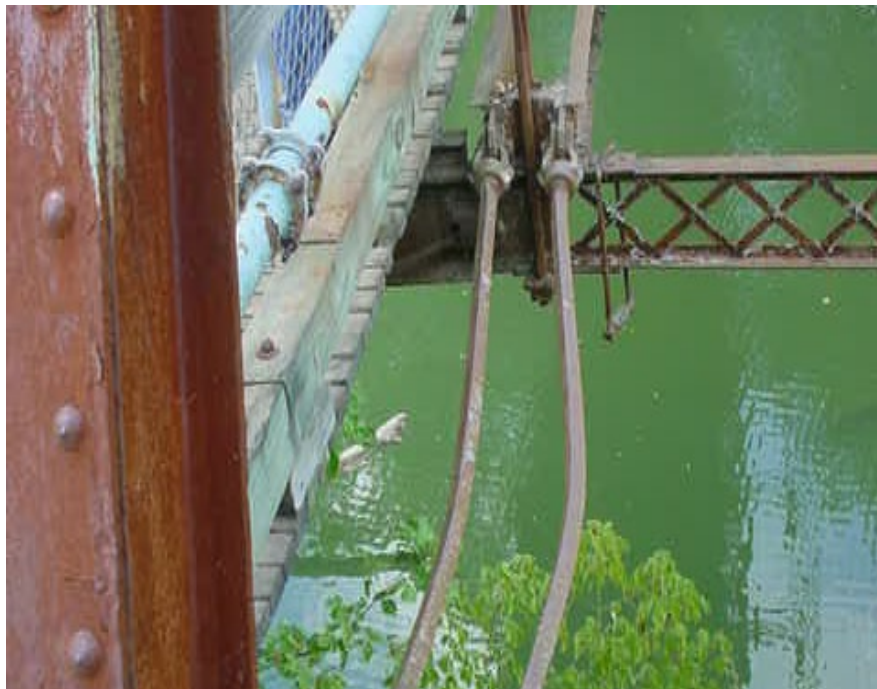
Figure 10.4.14 Bowed Bottom Chord Eyebar Member
