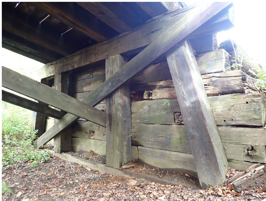
Figure 14.5.34 Decay on Timber Abutment
