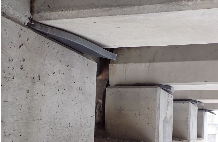
Figure 13.6.15 Plain Bearing Pads Walking Out from Under Beams
