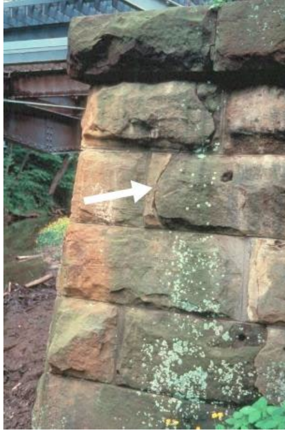
Figure 7.5.2 Splitting in Stone Masonry
