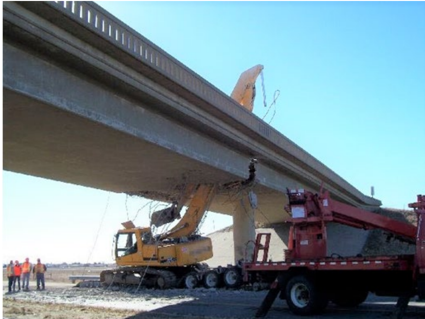
Figure 18.5.1 Bridge Damage from Construction Equipment
