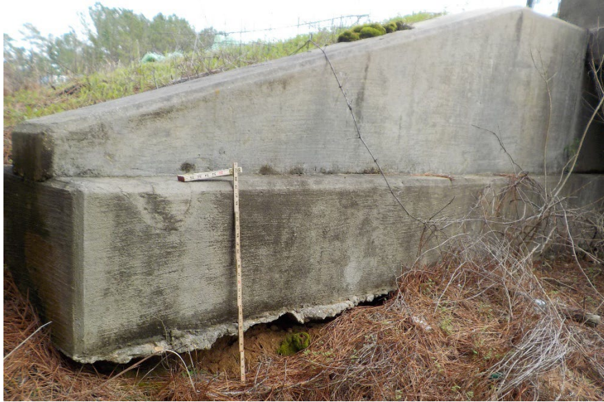
Figure 14.5.30 Undermining of Concrete Wingwall
