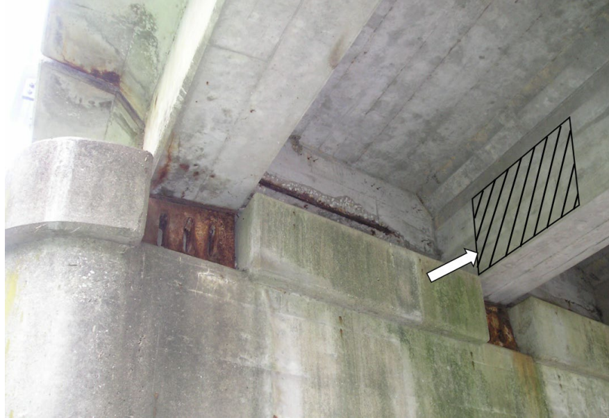
Figure 9.4.11 Shear Zone of Cast-in-Place Concrete Tee Beam Bridge
