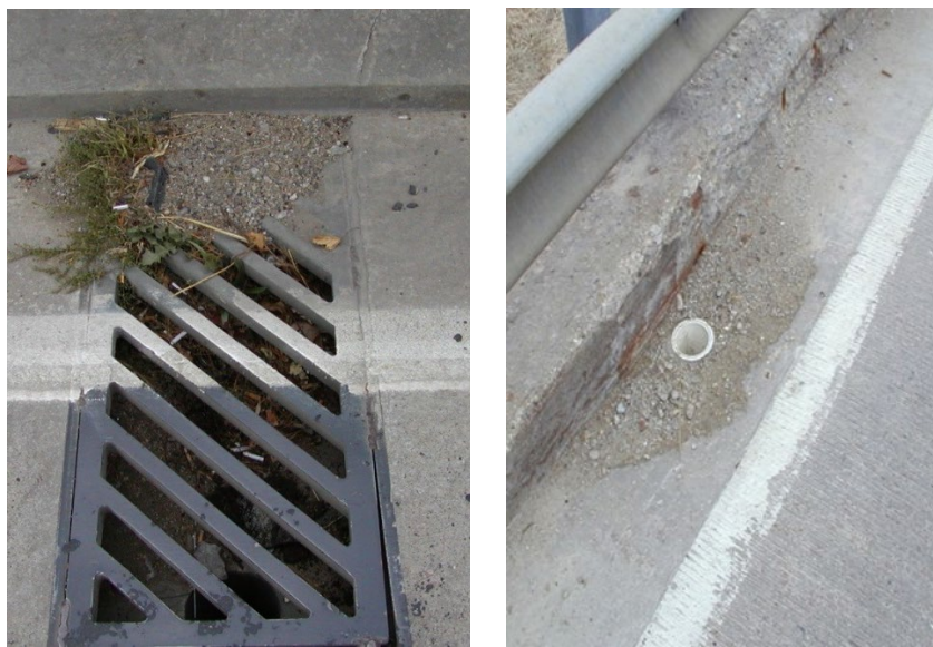
Figure 8.5.20 Bridge Deck Scupper (left) and Deck Drain (right)
