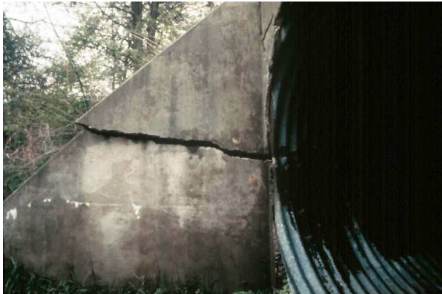
Figure 15.5.2 Cracking of Culvert End Treatment Due to Foundation Rotation
