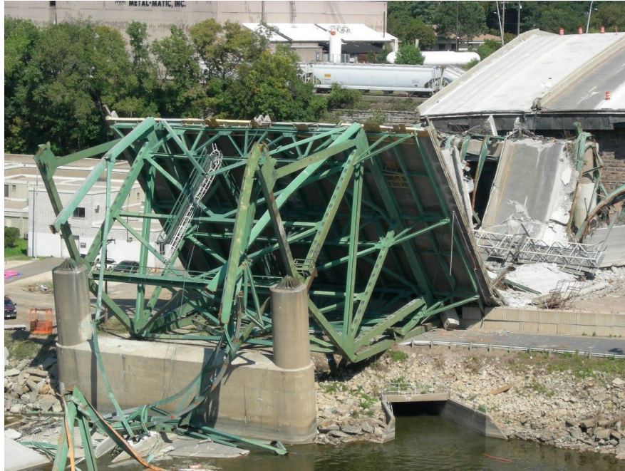
Figure 7.3.3 I-35W Mississippi River Bridge Collapse
