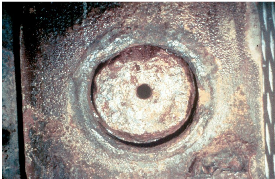
Figure 10.4.33 Corroded Pin-and-Hanger Assembly
