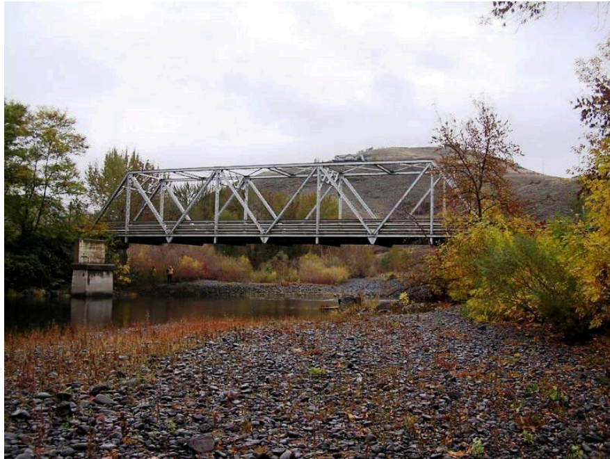
Figure 16.1.53 Stream Alignment Not Parallel with Abutments
