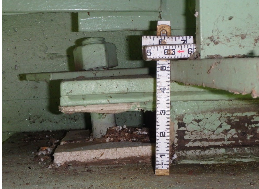
Figure 13.6.4 Bent Anchor Bolt due to Excessive Movement
