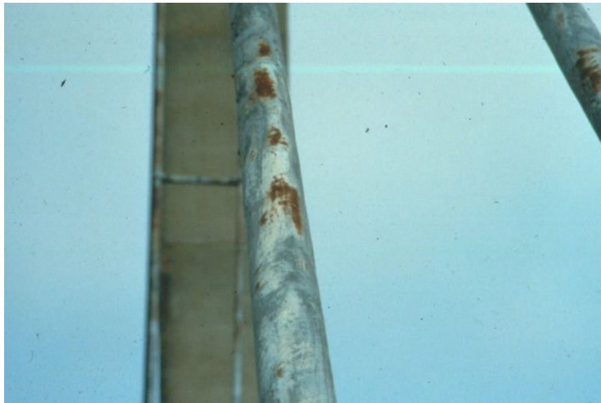
Figure 12.2.7 Corrosion of Steel Sheathing
