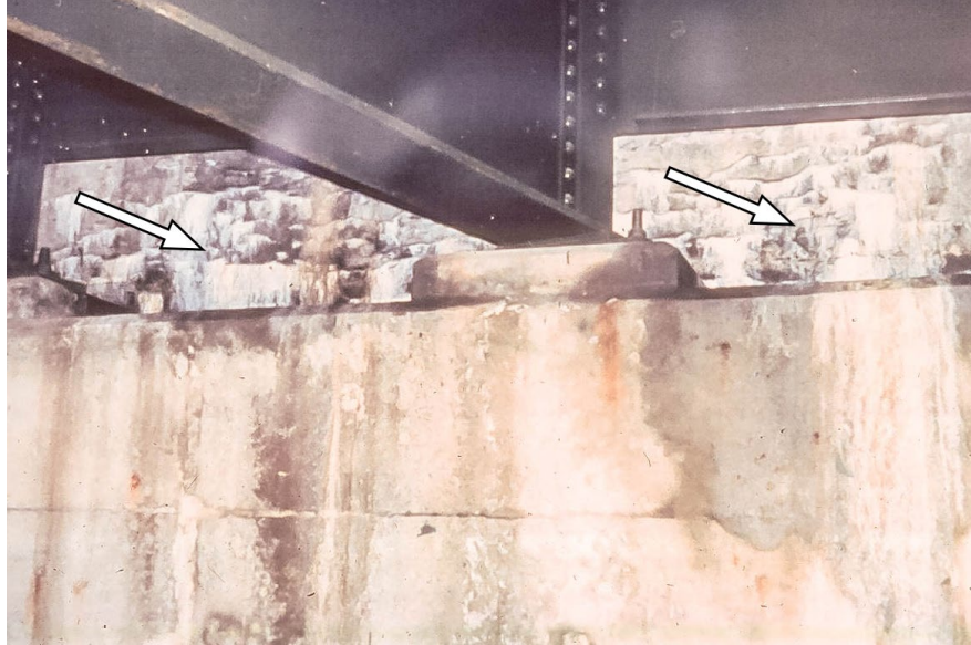
Figure 14.5.20 Cracking and Efflorescence in Backwall
