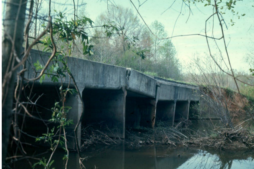
Figure 16.1.54 Rotational Movement and Failure Due to Undermining
