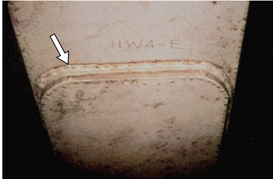
Figure 7.3.30 Part-through Crack Growth at Cover Plate Welded to Flange
