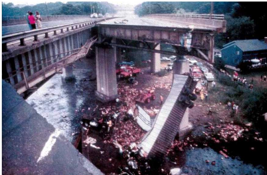
Figure 10.5.2 Mianus River Bridge Failure - From Deck
