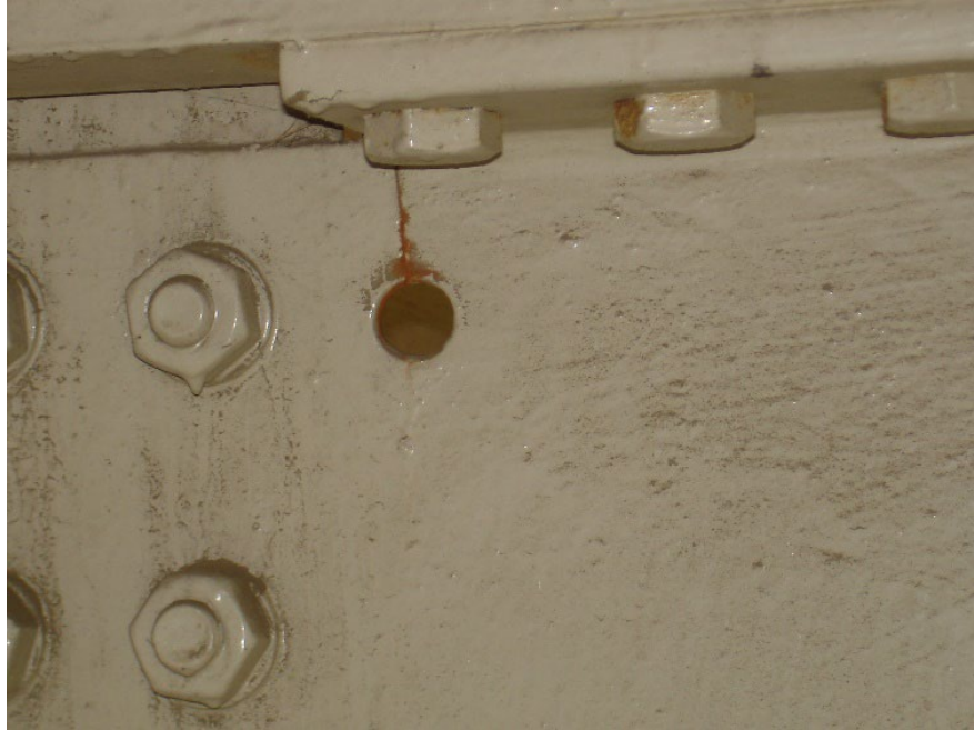
Figure 7.3.25 Crack Arrest Hole in Stringer Web at Coped Flange Location
