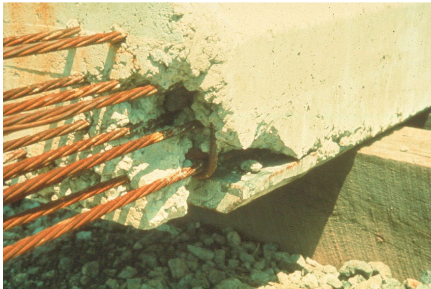
Figure 9.4.4 Bearing Area: Spalling Due to Poor Concrete and Steel Placement
