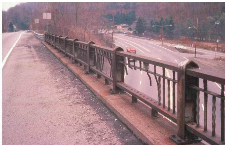
Figure 8.6.4 Steel Post Bridge Railing with Impact Damage
