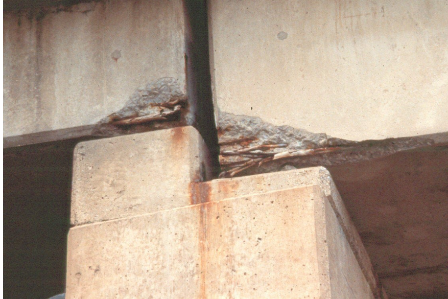
Figure 9.4.5 Bearing Area: Spalled Beam Ends with Exposed Prestressing Reinforcement
