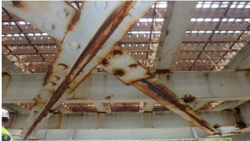
Figure 10.4.63 Sway Bracing with Pack Rust
