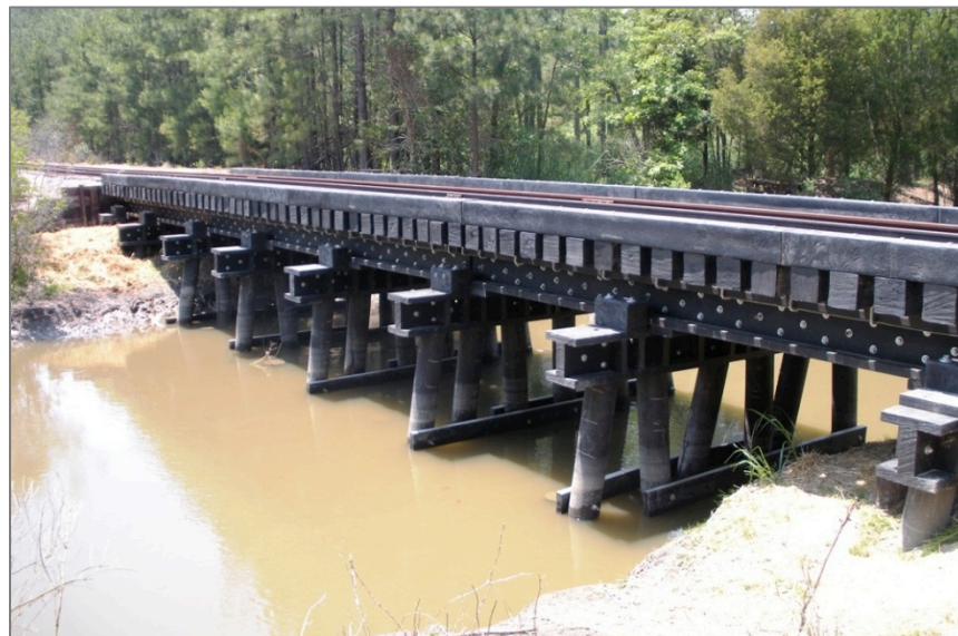
Figure 2.5.2-1. Prefabricated Thermoplastic Railroad Bridge.
