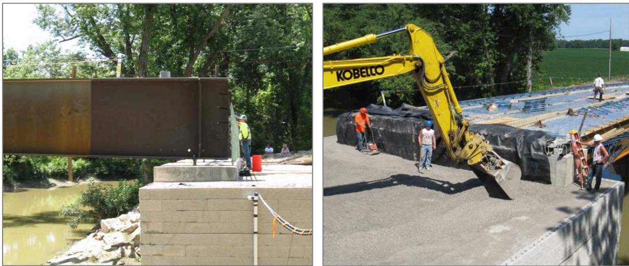
Figure 5.1.4-2. GRS-IBS Bridge Built with Steel Girders. Left: Concrete Footing Supporting Girders Right: Backfilling after casting of Integral Diaphragm (Source: FHWA).
