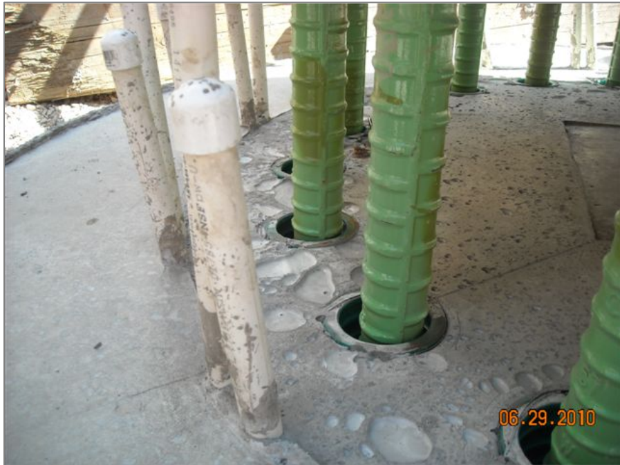
Figure 5.2.4-3. Inverted Grouted Reinforcing Splice Coupler Connection (Source: Hanson Structural Precast, Salt Lake City).
