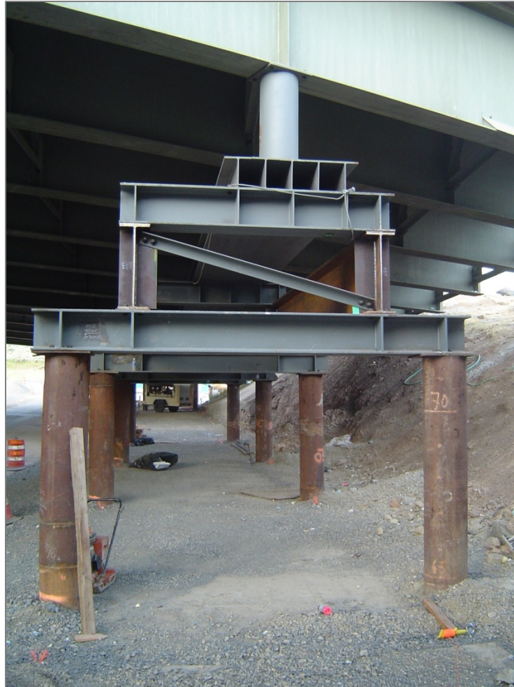
Figure 11.4.4-2. Temporary support frame on an SPMT move where the deck is cast in the “as lifted” position.
