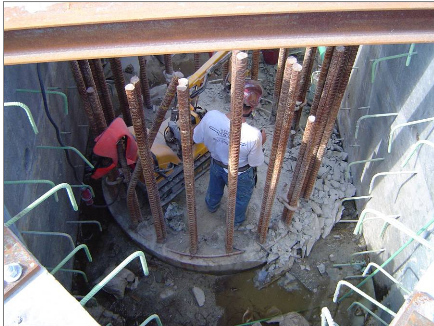
Figure 7.2.4-2. Top and Bottom photos: Precast Concrete Pier Box Cofferdam Installation in Rhode Island.
