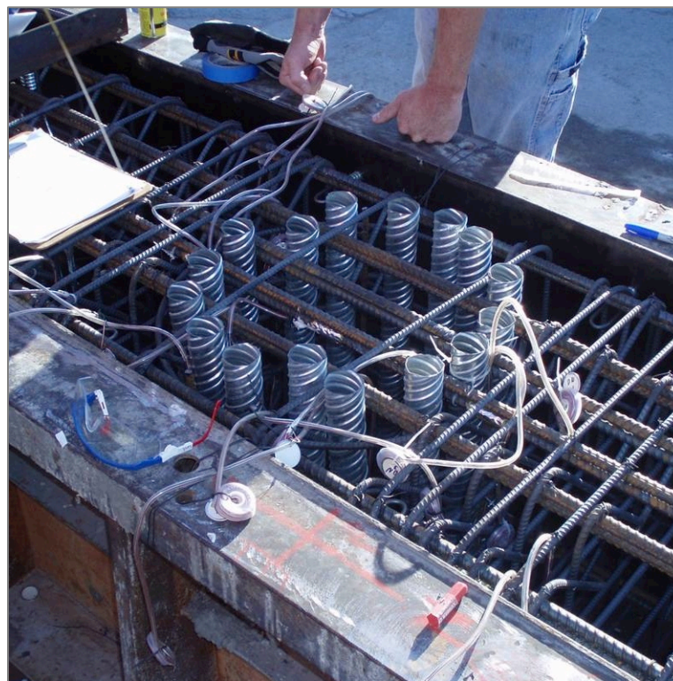
Figure 5.2.3.2-2. Column to Cap Connection using Grouted PT Ducts Connection (Source: NCHRP Project 12-74).
