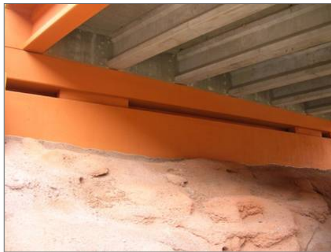
Figure 11.4.5-1. Lateral Slide Bridge in Utah Top Photo: Sliding pads on abutment seat with skid shoe to the right. Bottom Photo: Bridge in final position supported on integral skid shoes. (Source: HB Engineering)
