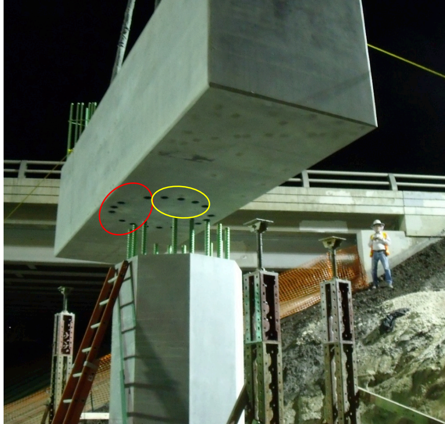
Figure 5.2.3-2. Layout of Bar Couplers in Pier cap (Source: Hanson Structural Precast, Salt Lake City).
