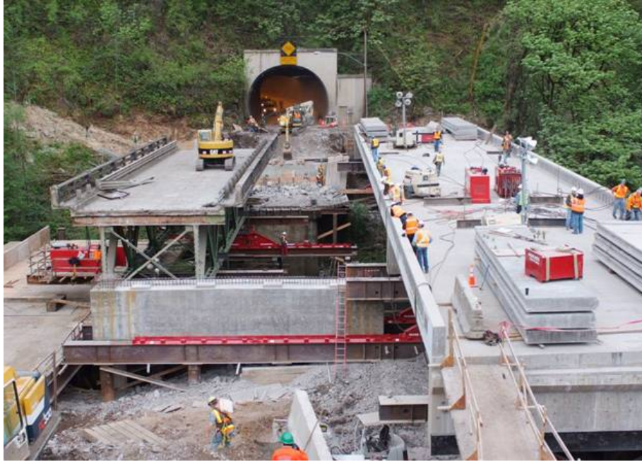
Figure 11.4.5-2 Lateral slide project in Oregon using independent skid frames (Source: Oregon DOT).
