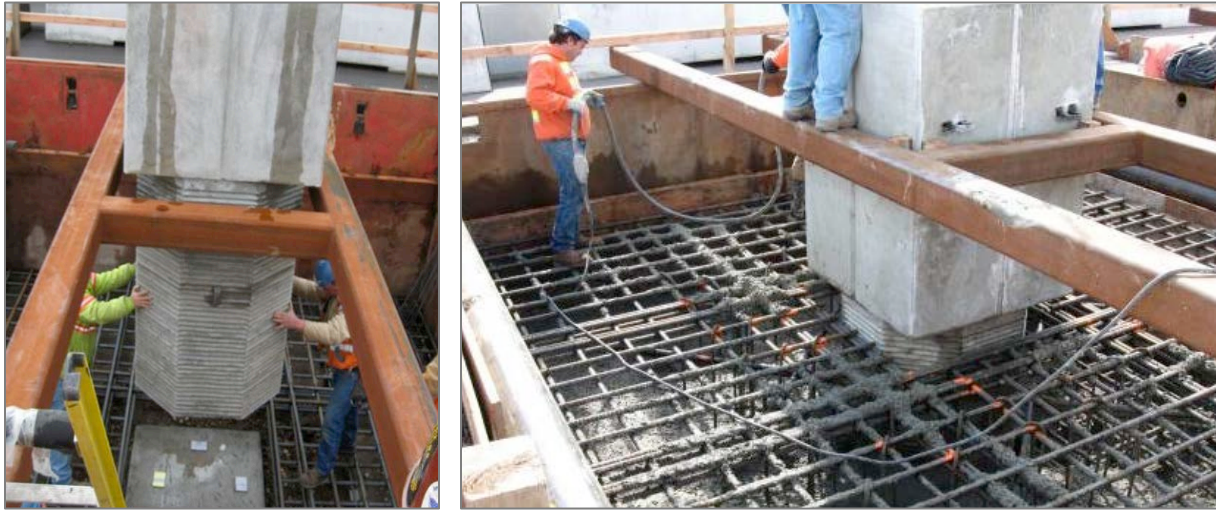
Figure 7.1.2-2 Corrugated Column End with Cast-in-place Concrete Footing. Left: Installation of column on temporary pad. Right: Placement of concrete after installation of top reinforcing mat. (Source: FHWA Highways for LIFE).
