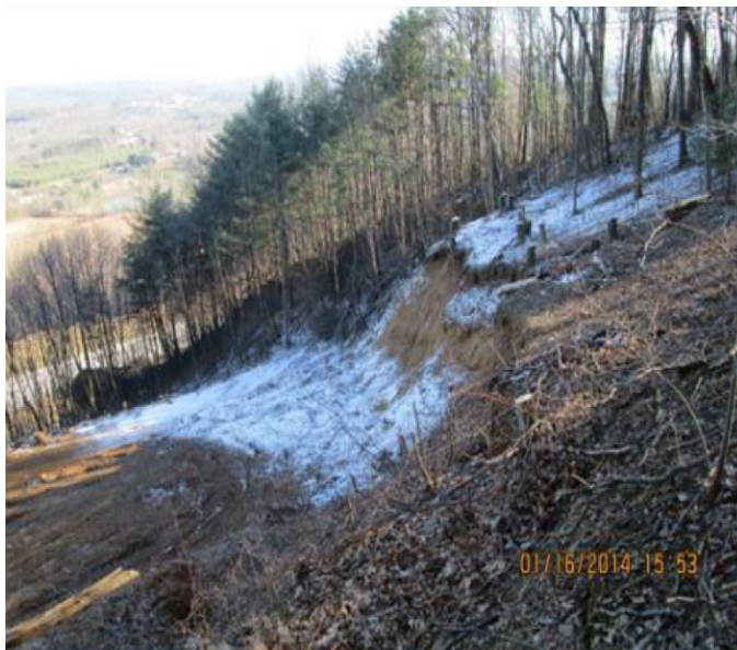
Figure 3-2: Soil slope along Virginia I-77.
