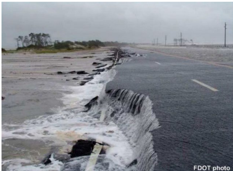
Figure 3-3: Damage to U.S. Highway 98 in 2005 due to a tropical storm (Okaloosa County, Florida).
