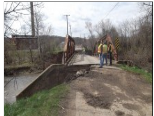
View of Township Road 82 Bridge looking at the South Abutment from on top of the road.
