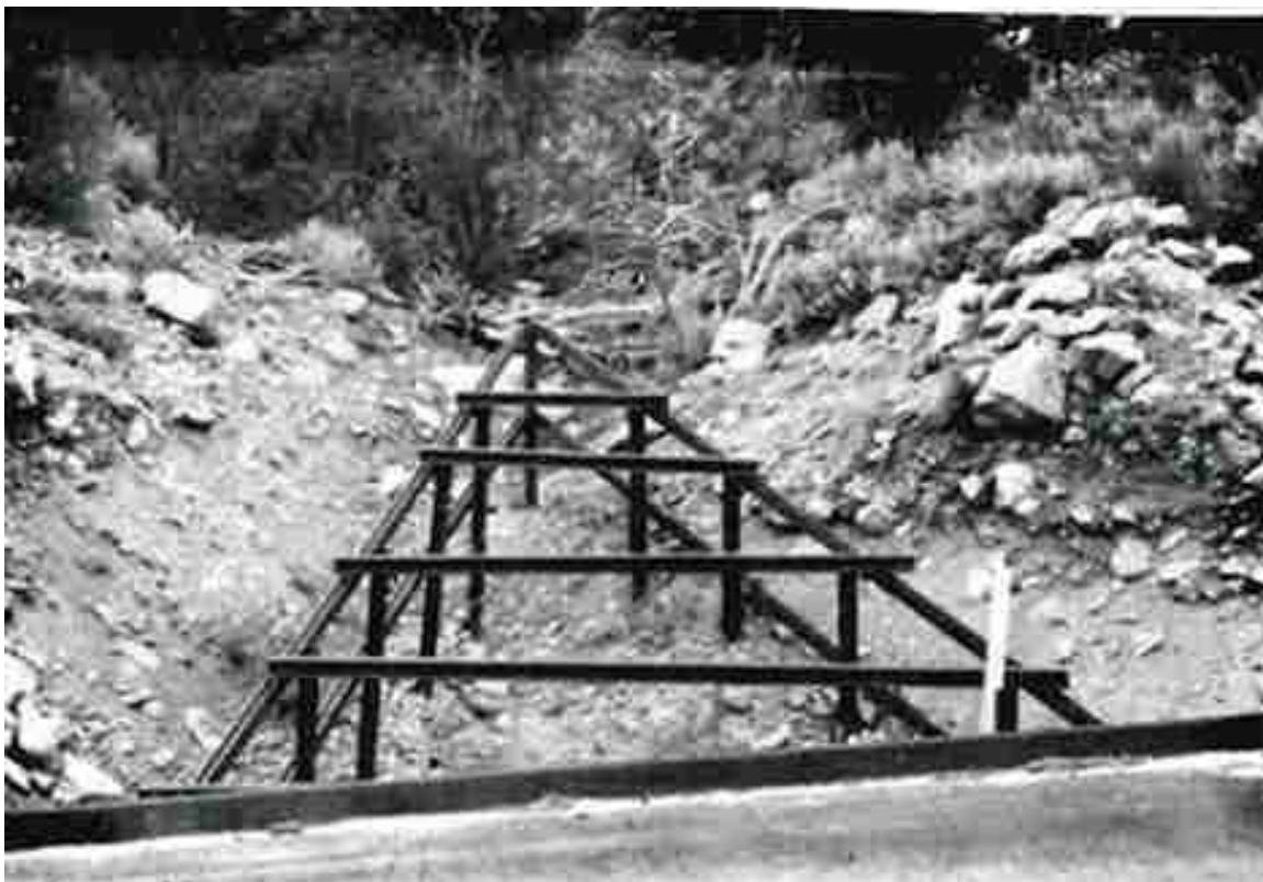
Figure 5.1. Steel rail debris deflector for large rock (looking upstream of culvert).
