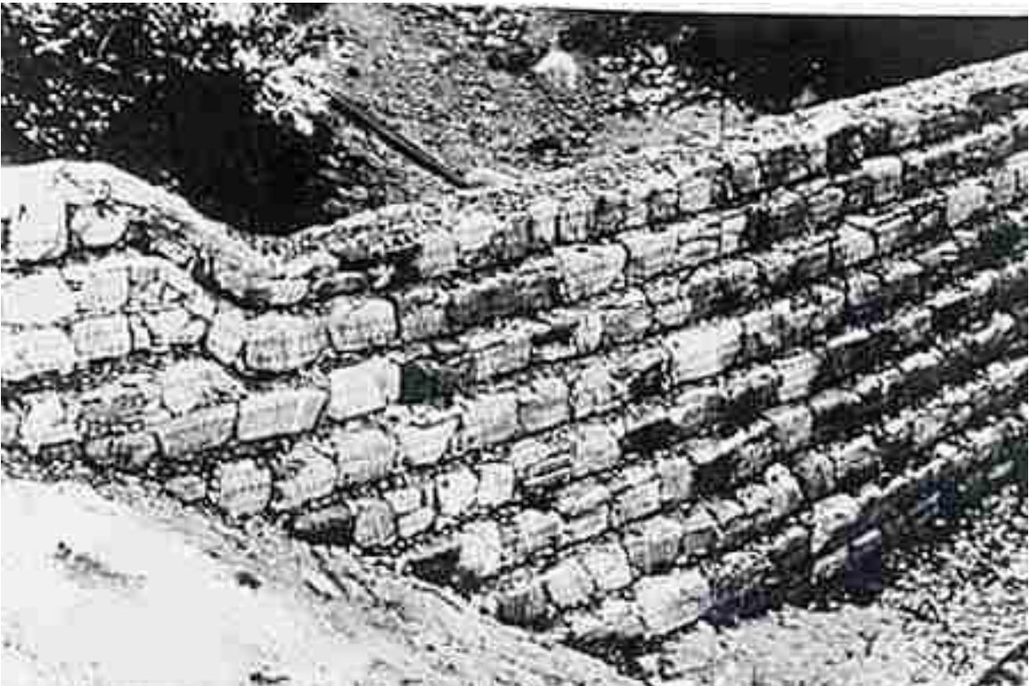
Figure 5.37. Gabion debris dam.
