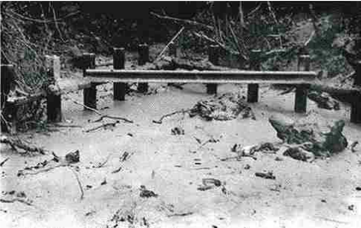
Figure 5.7. Steel rail debris deflector in area of heavy flowing debris (looking upstream).
