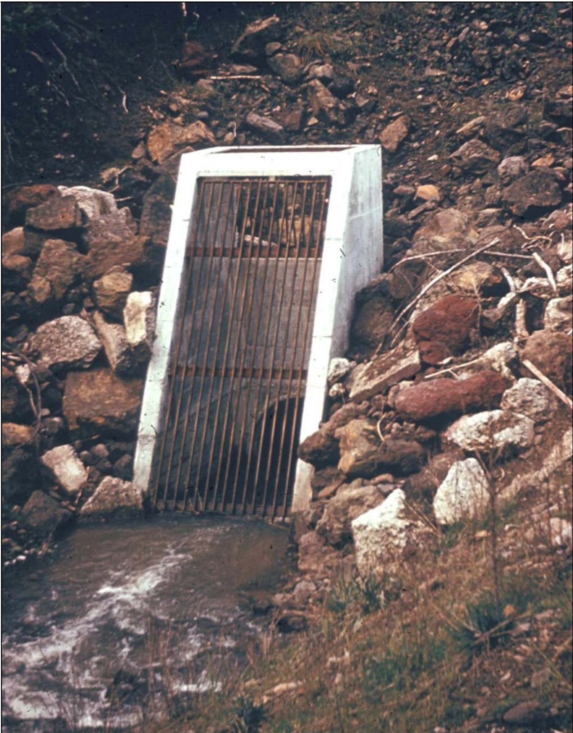
Figure 5.16. Debris rack used in State of Washington.
