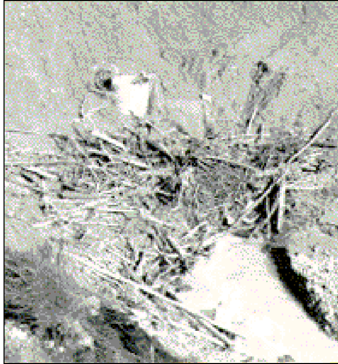
Figure 5.25. Installation shown in Figure 5.24 after flood. Riser conveyed large flows during flood. Fence partially surrounding riser was of no value for debris control.
