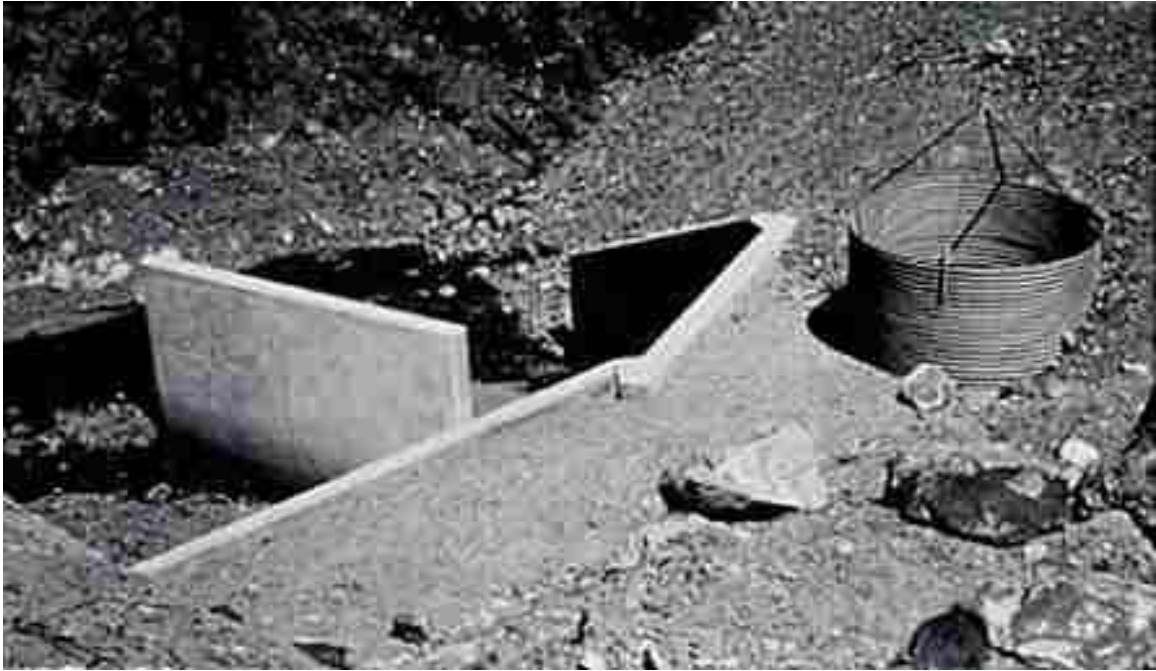
Figure 5.34. Debris fin and metal pipe debris riser in conjunction with single barrel culvert.
