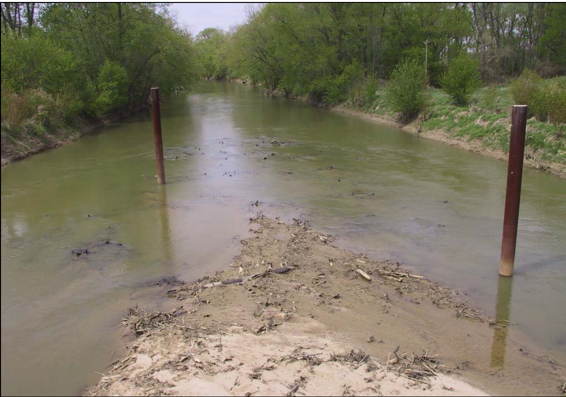
Figure 5.43. Debris deflectors installed at State Route 59 south crossing of the Eel River in central Indiana.
