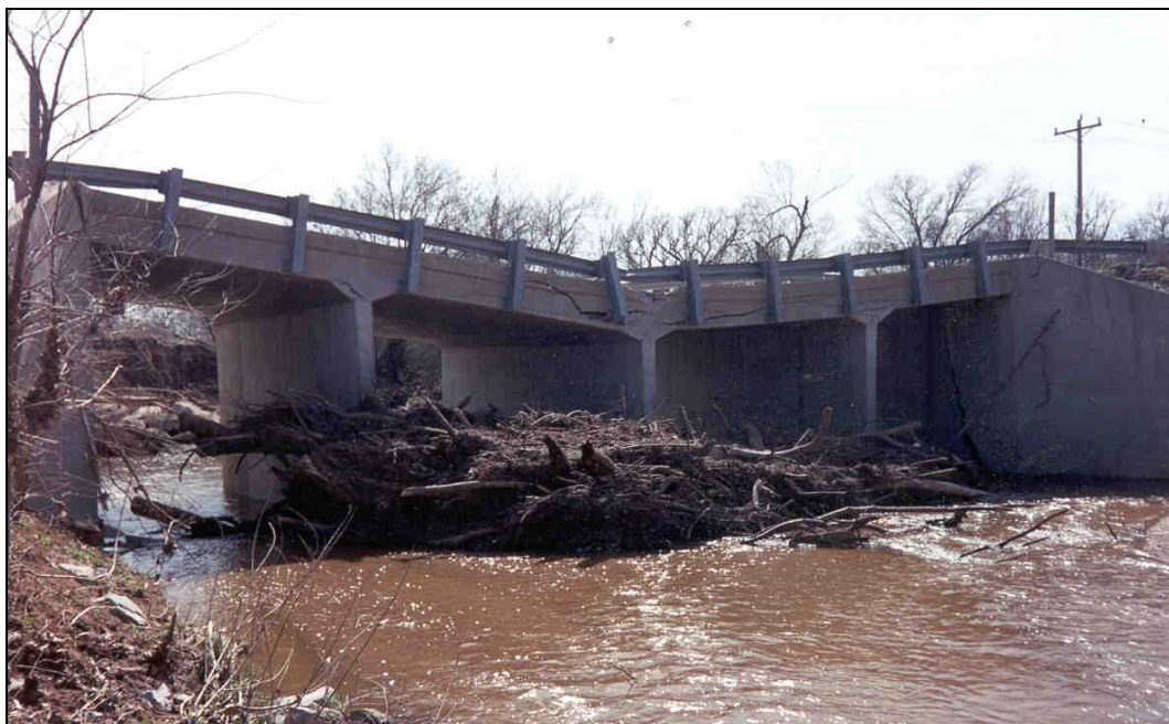
Figure 2.5. Debris accumulation failure at bridge located in Oklahoma.
