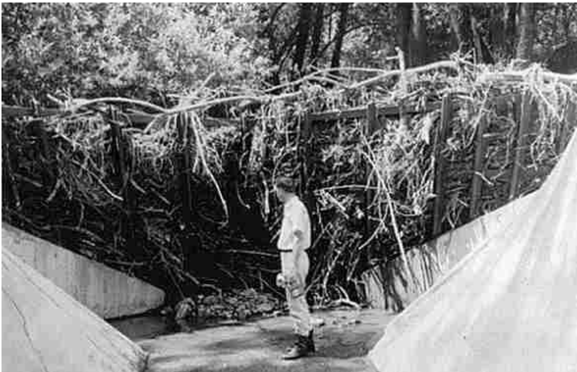
Figure 5.20. Steel debris rack probably saved the culvert from plugging.
