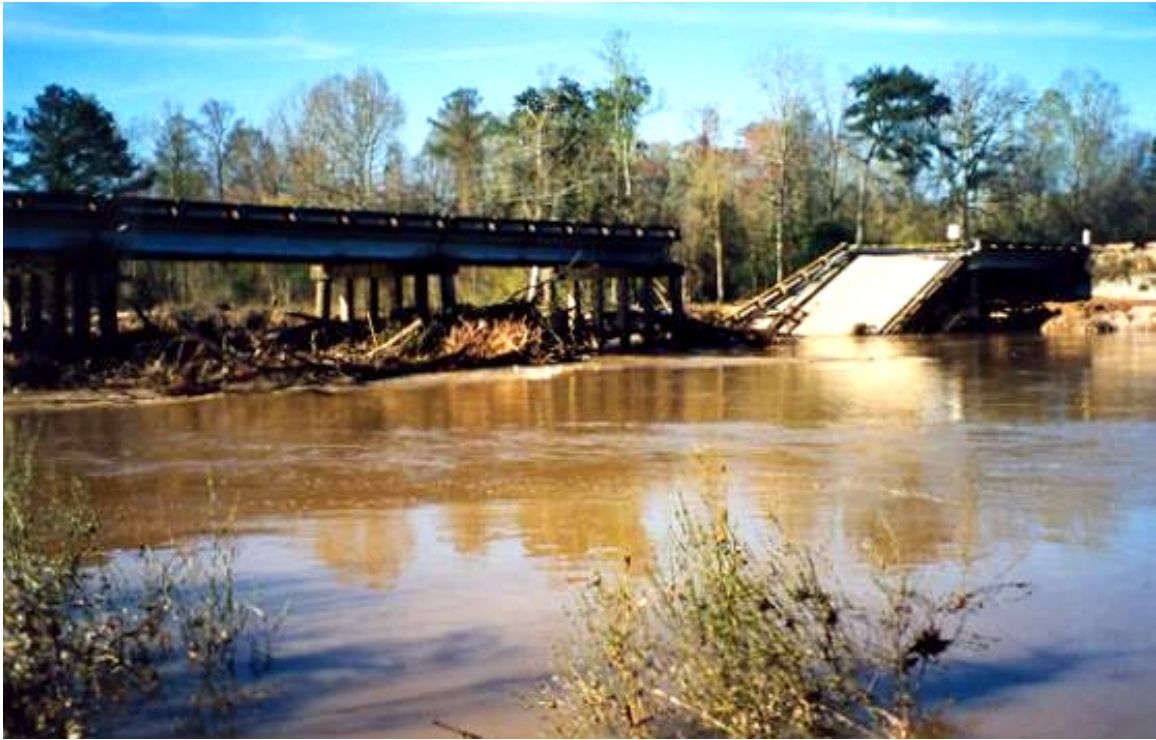
Figure 2.3. Span blockage accumulation bridge failure. (Louisiana)
