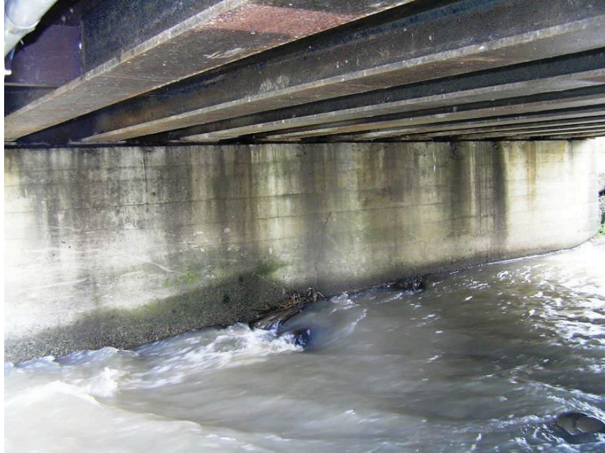
Figure 16.1.56 Accelerated Flow Due to Constricted Waterway
