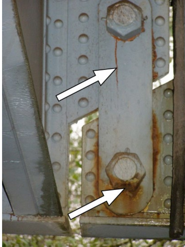
Figure 10.4.30 Rust Stains from Pin Corrosion
