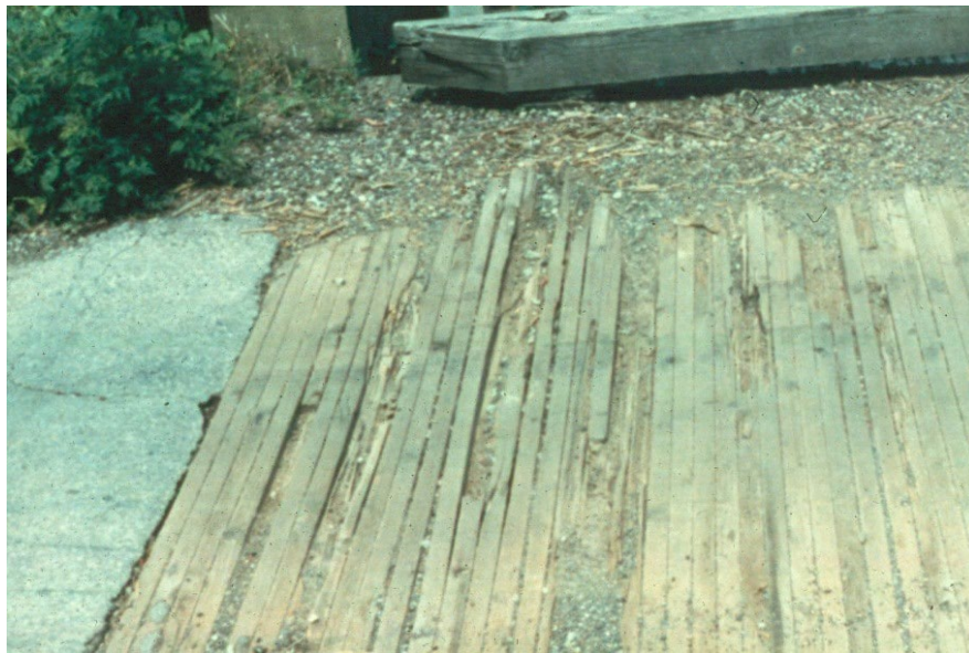
Figure 8.3.8 Wear and Weathering on a Timber Deck
