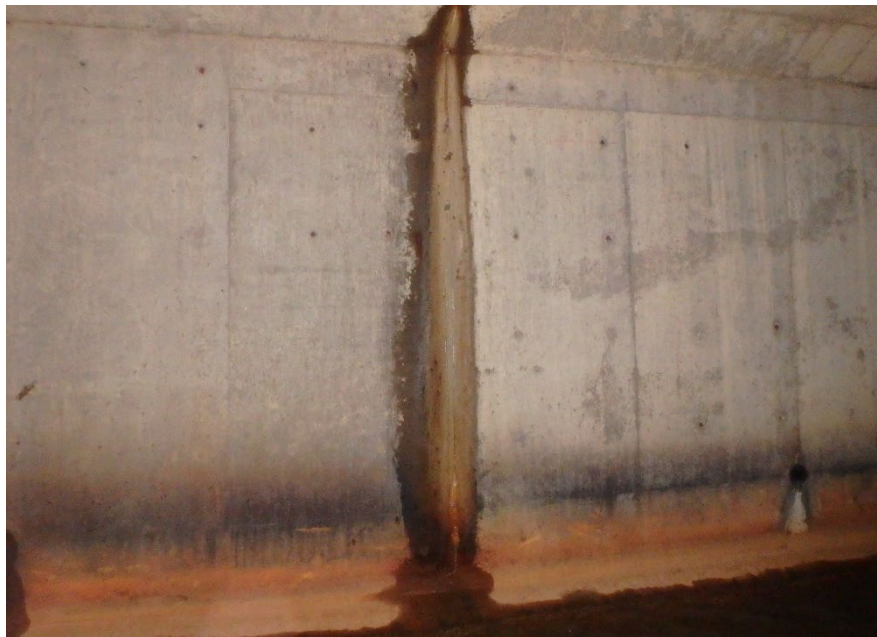
Figure 15.5.11 Precast Concrete Box Culvert Joint with Infiltration
