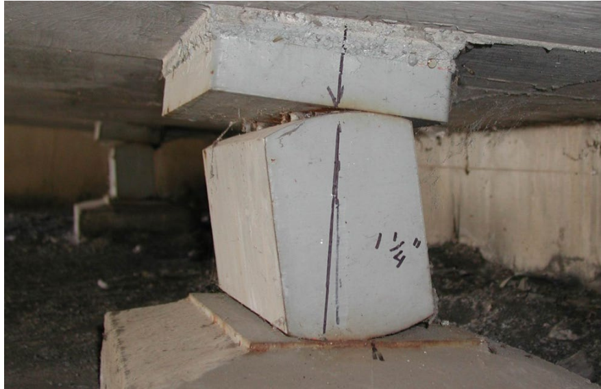
Figure 13.6.7 Excessive Tilt in a Segmental Rocker
