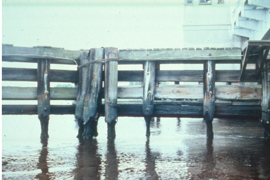
Figure 14.5.32 Timber Fender System with Deteriorated Piles
