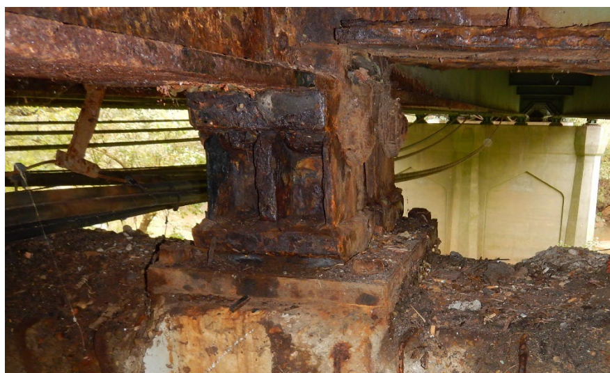
Figure 13.6.2 Heavy Corrosion on a Steel Rocker Bearing
