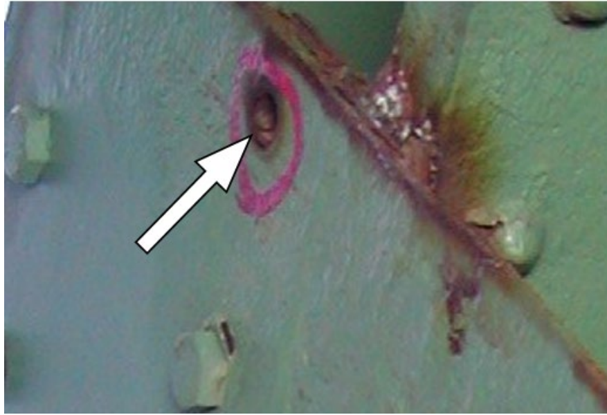
Figure 10.4.45 Missing Bolts on a Gusset Plate
