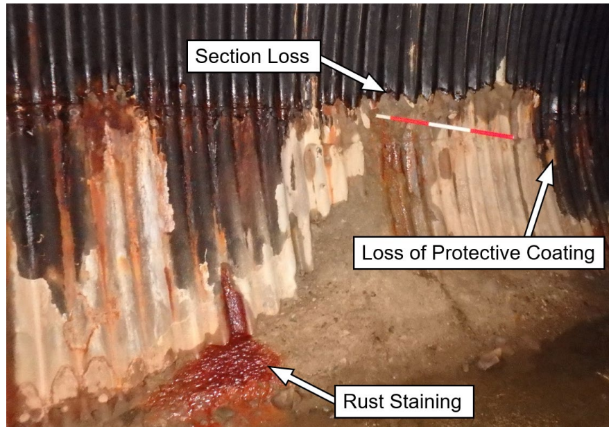
Figure 15.4.1 Advanced Deterioration of a Flexible Culvert Section
