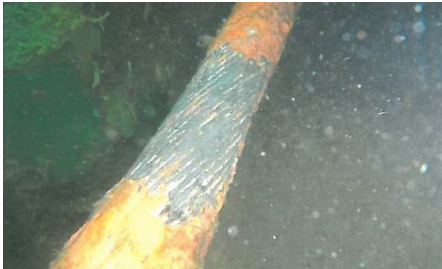
Figure 12.4.3 Cable Corrosion within Pontoon Port
