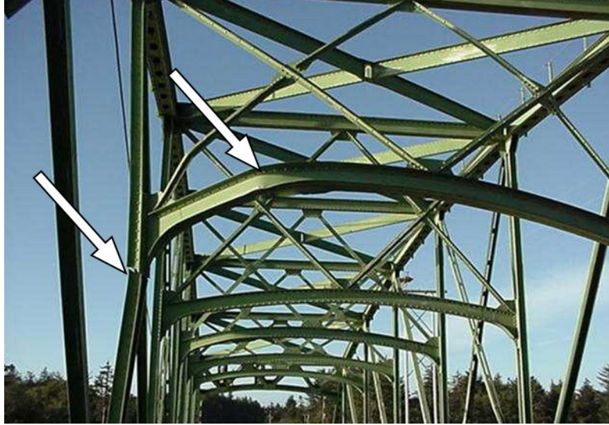
Figure 10.4.23 Collision Damage to Truss Members Due to Over-height Vehicle
