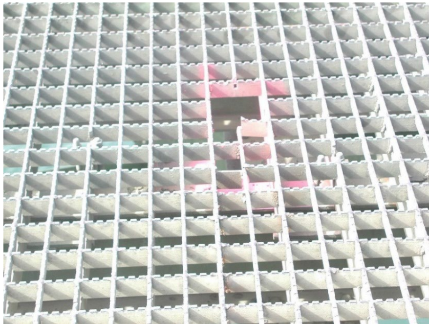
Figure 8.2.10 Broken Members of an Open Steel Grid Deck
