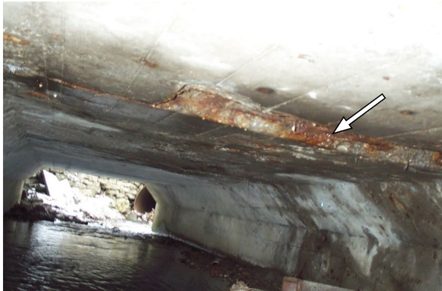
Figure 15.5.6 Spalls and Delaminations on Top Slab of Concrete Box Culvert
