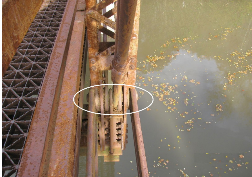
Figure 10.1.108 Loosely Packed Eyebar Connection
