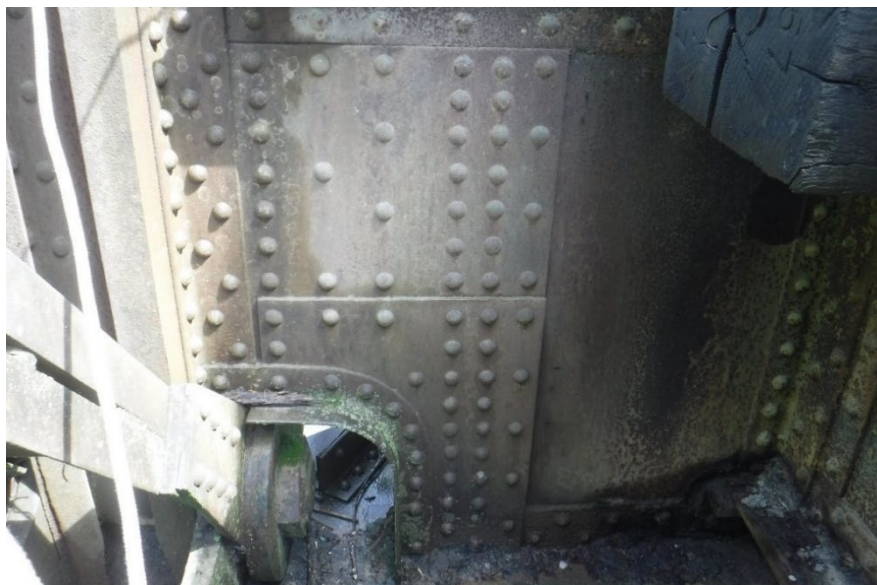
Figure 10.4.25 Corroded Floorbeam End Connection with Deicing Chemical Residue
