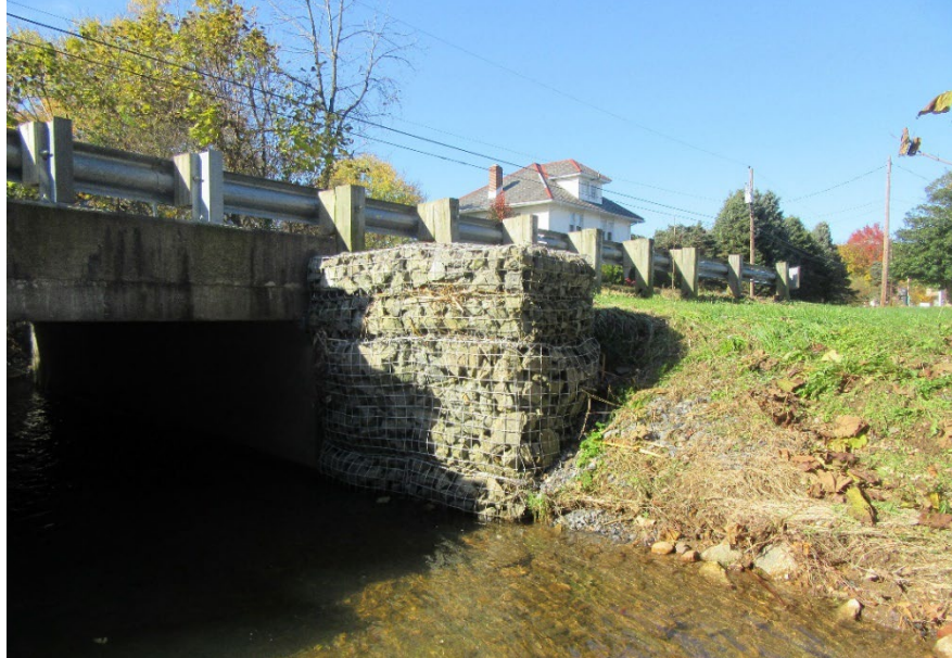
Figure 4.3.12 Gabion Basket Serving as Slope Protection
