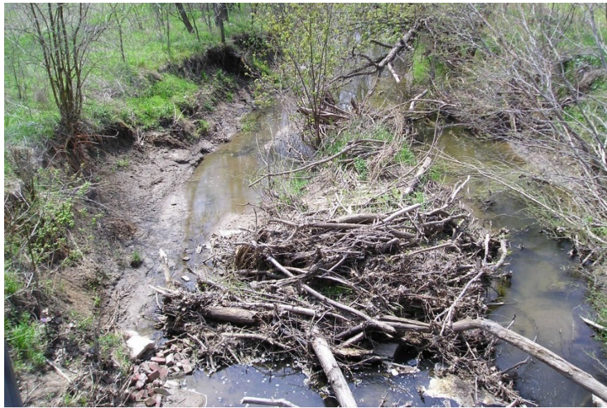
Figure 16.1.46 Debris and Sediment in the Channel
