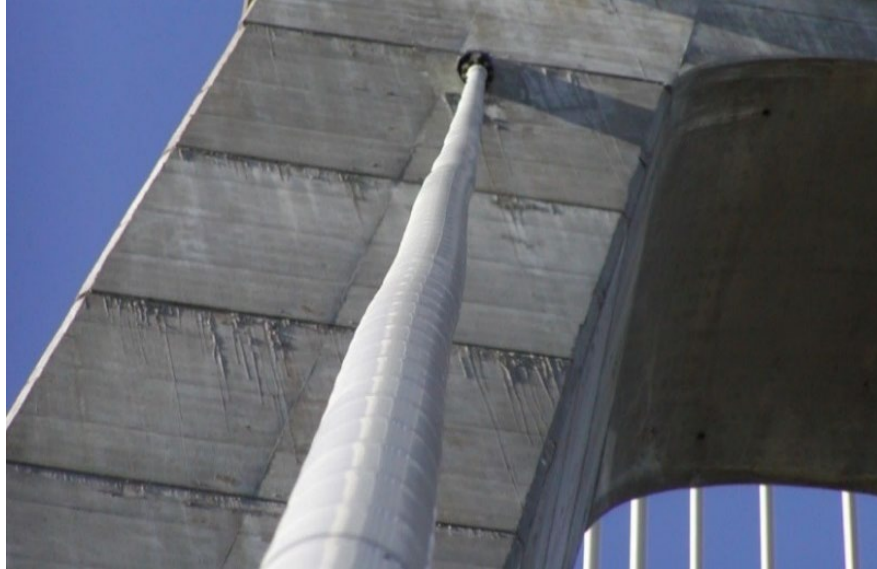
Figure 12.2.9 Bulging of Cable Sheathing
