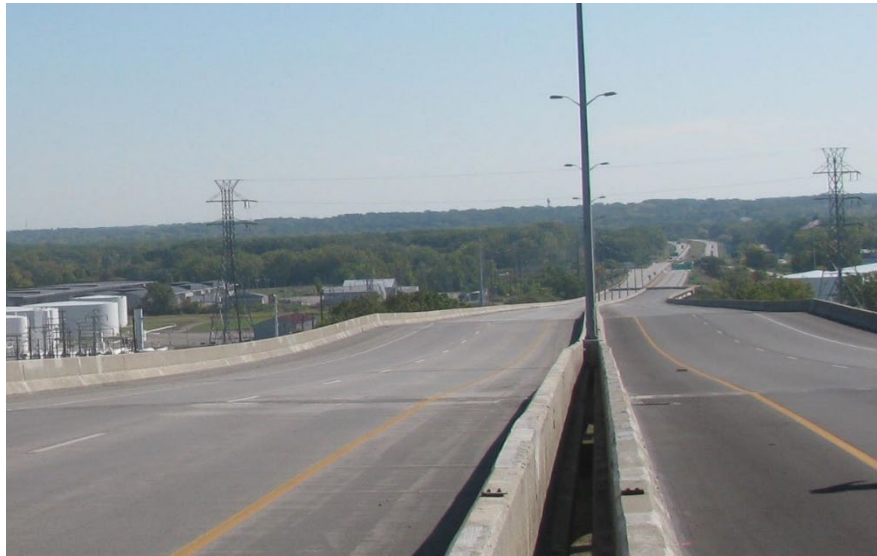
Figure 14.5.6 Deck and Railing Evidence of Pier Settlement
