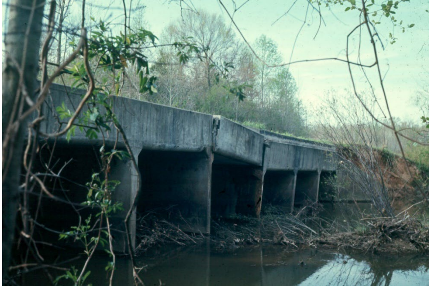
Figure 16.1.54 Rotational Movement and Failure Due to Undermining
