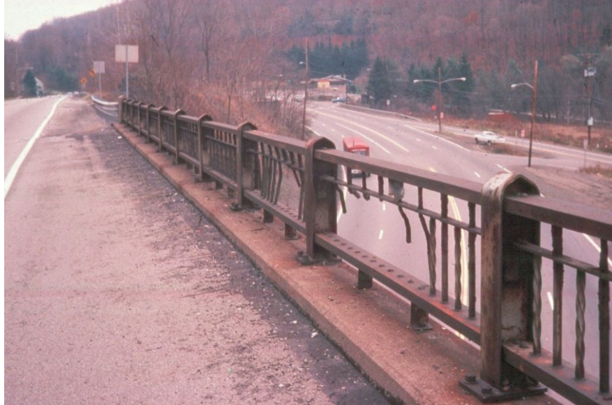
Figure 8.6.4 Steel Post Bridge Railing with Impact Damage
