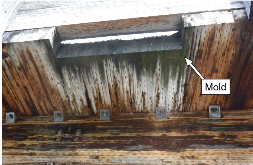
Figure 7.4.10 Mold and Stains on the Underside of a Timber Bridge
