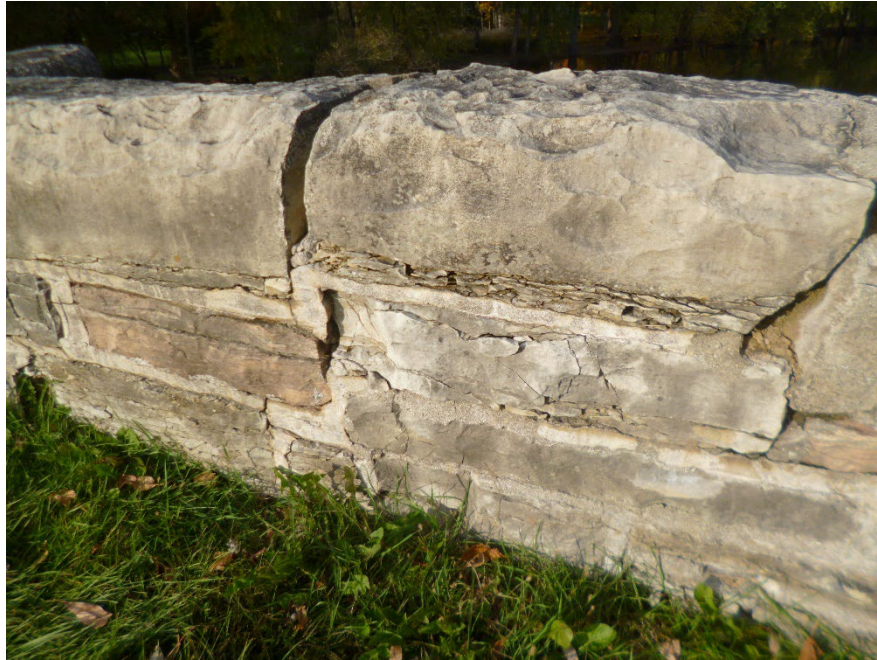
Figure 11.5.14 Top of Spandrel Wall Exposed to Traffic
