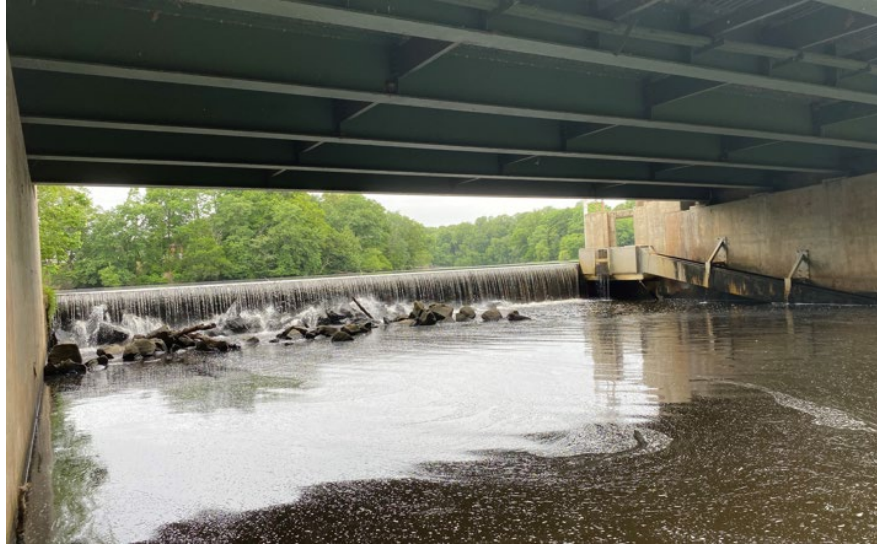
Figure 16.1.47 Upstream Dam Impacts Streamflow on Bridge
