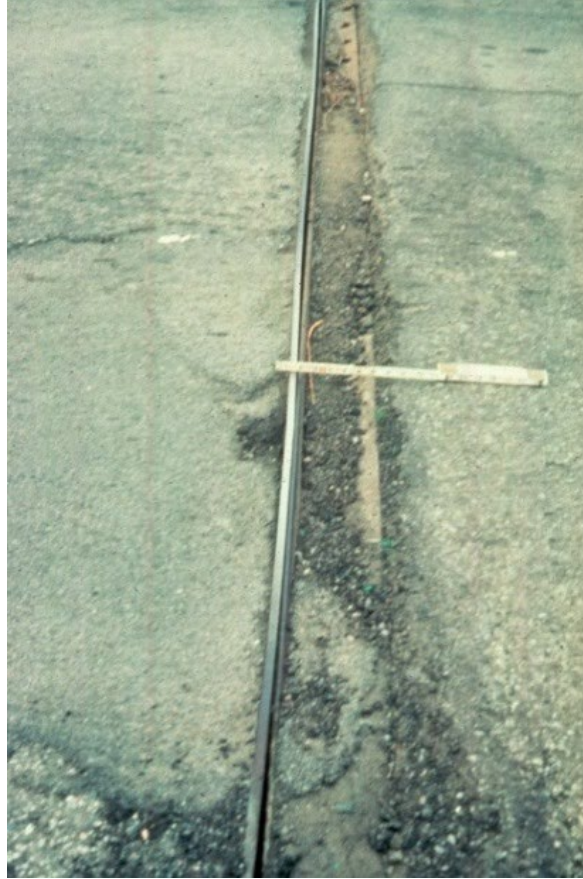
Figure 8.5.25 Deck Joint with Dirt and Debris Accumulation
