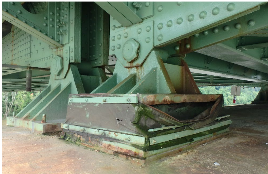
Figure 13.3.6 Failed Roller Nest Skirt
