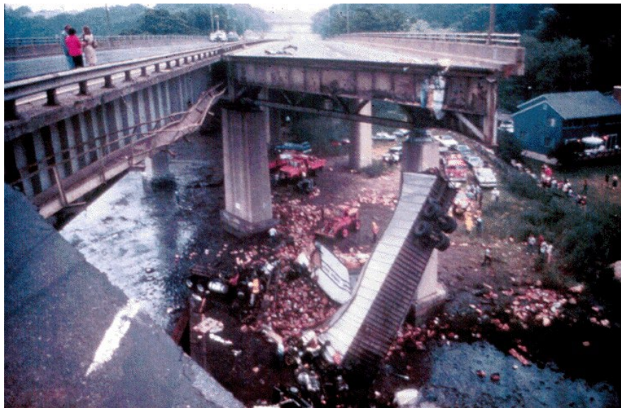
Figure 7.3.2 Mianus River Bridge Collapse
