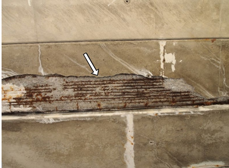
Figure 9.4.25 Spall and Exposed Corroded Reinforcement Strands, Mid-Span of Box Beam
