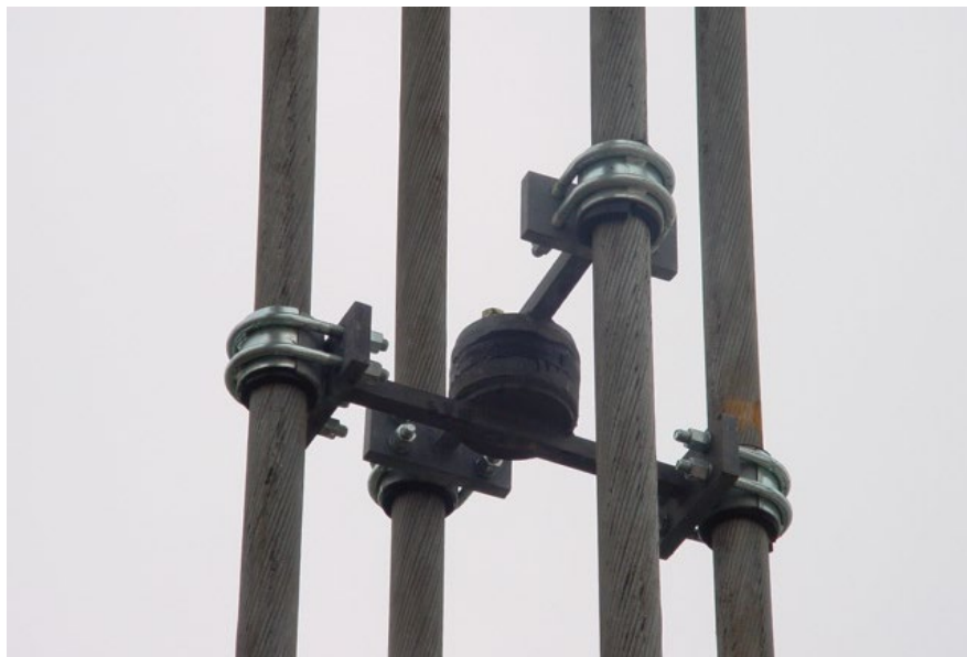
Figure 5.2.20 Cable Damper System
