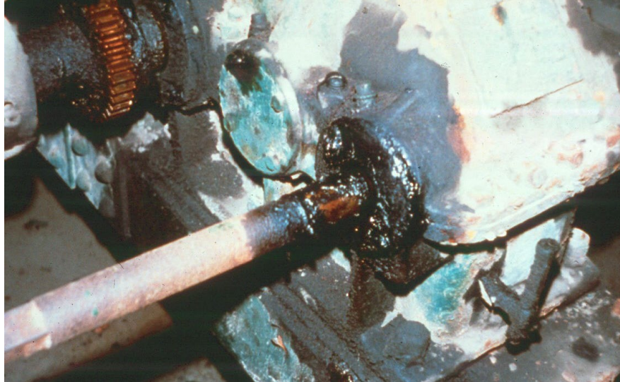
Figure 12.3.9 Leaking Speed Reducer
