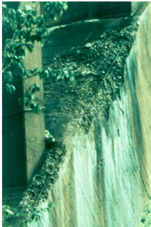
Figure 9.4.37 Scaling and Contamination on an Arch Rib Due to a Failed Drainage System
