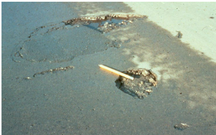
Figure 7.1.24 Spalling on a Concrete Deck
