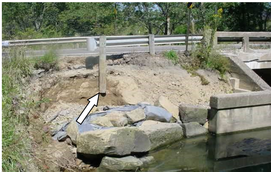
Figure 8.6.6 Exposed Transition Post due to Roadway Runoff Erosion
