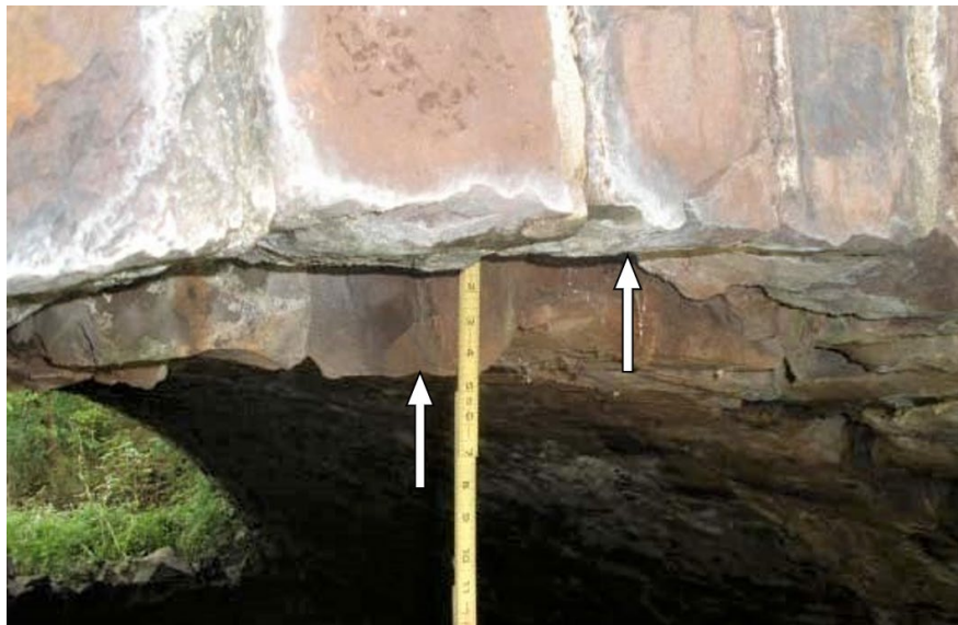
Figure 11.5.13 Downward Deflection of Masonry Arch
