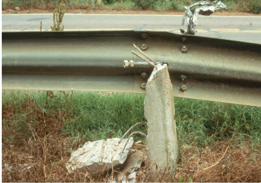
Figure 8.6.5 Approach Guardrail and Post with Collision Damage
