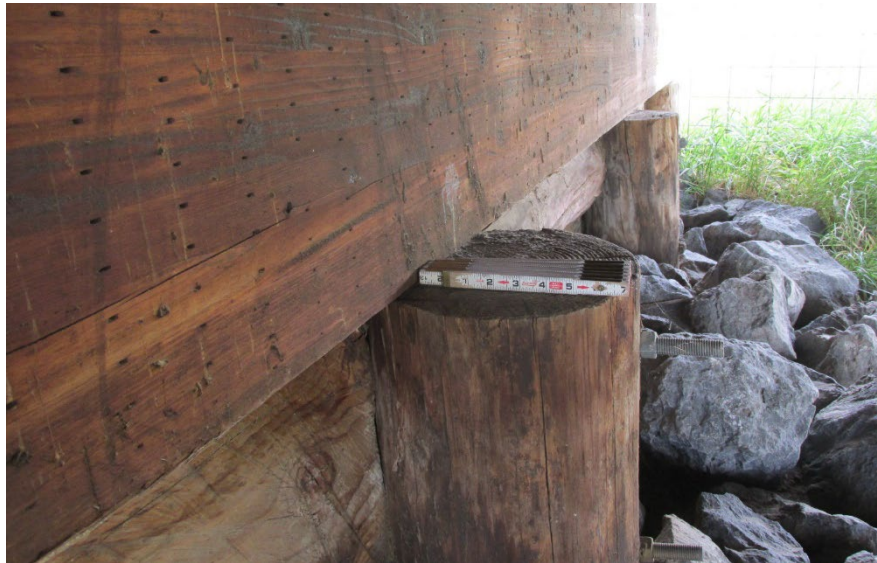
Figure 14.5.9 Local Failure in Timber Pile/Abutment Seat Interface Indicating Possible Movement of Abutment
