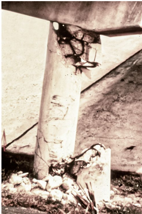
Figure 7.1.31 Concrete Column Collision Damage
