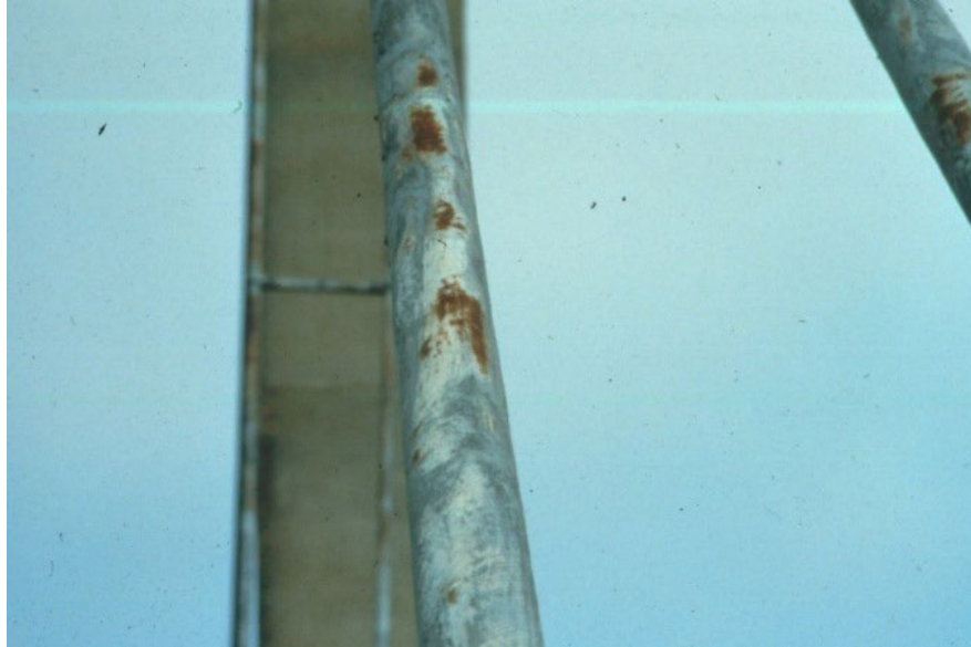
Figure 12.2.7 Corrosion of Steel Sheathing
