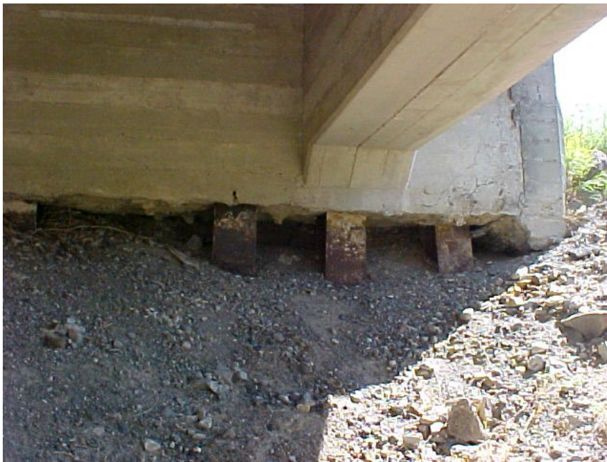
Figure 16.1.55 Exposed Piling Due to Scour
