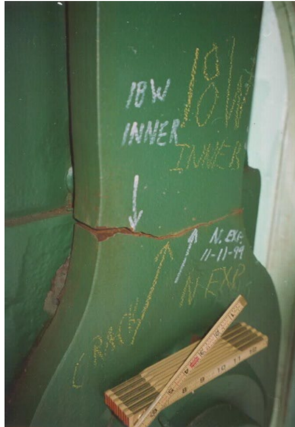
Figure 10.4.31 Cracked Forge Zone on an Eyebar
