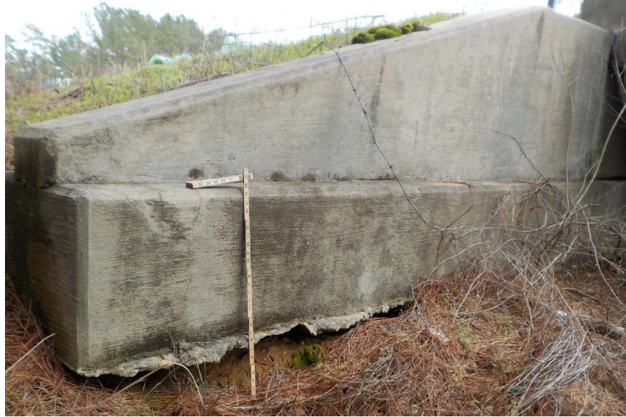
Figure 14.5.30 Undermining of Concrete Wingwall
