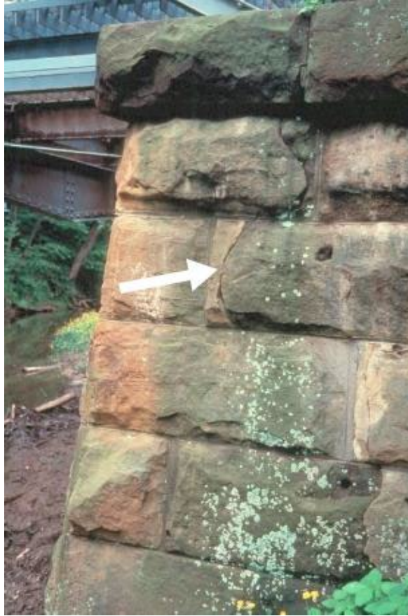
Figure 7.5.2 Splitting in Stone Masonry
