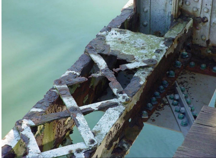
Figure 10.4.11 Corrosion and Section Loss on a Truss Bottom Chord
