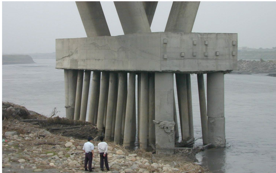
Figure 16.1.16 Pier Foundation Exposed by Scour
