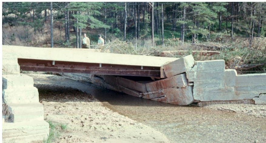
Figure 14.5.27 Abutment Failure from Undermining due to Scour
