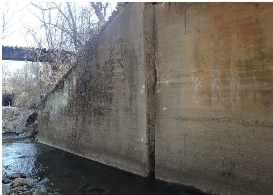
Figure 14.5.16 Rotational Movement of a Concrete Wingwall
