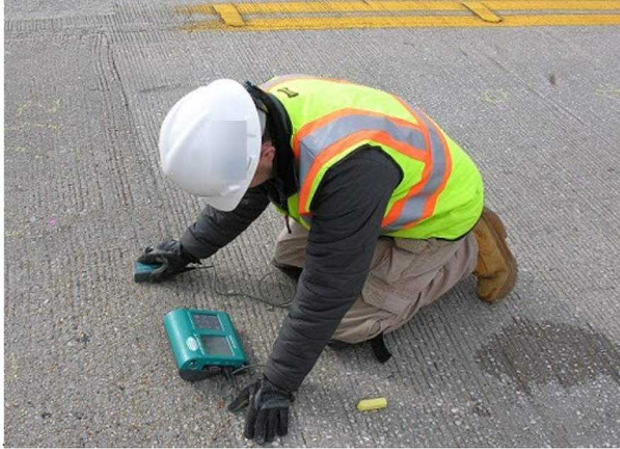
Figure 17.2.10 Locating Rebar with a Magnetometer
