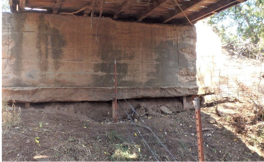
Figure 14.5.12 Erosion at Abutment Exposing Piles
