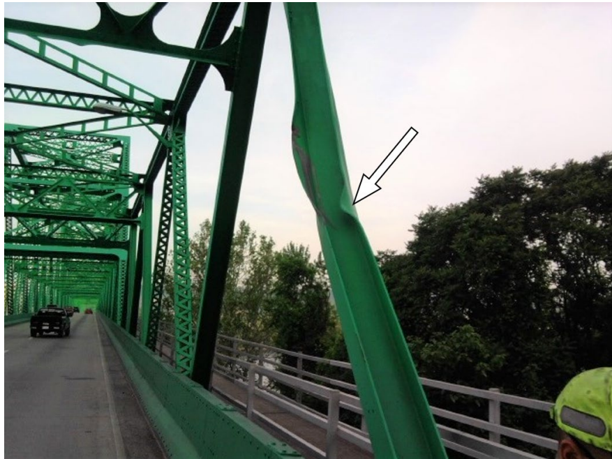
Figure 10.4.17 Buckled End Post
