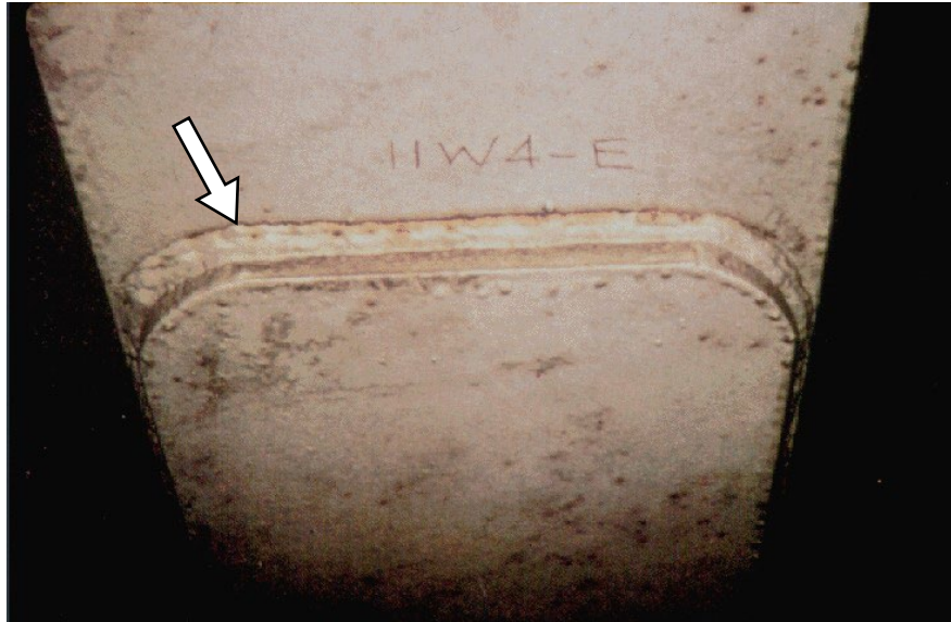
Figure 7.3.31 Part-through Crack Growth at Cover Plate Welded to Flange
