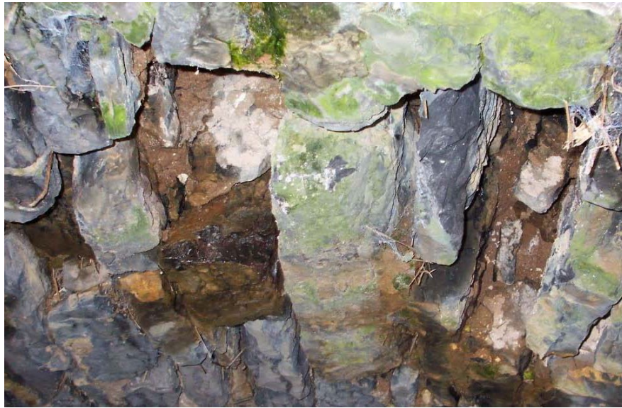
Figure 15.5.8 Drainage Through Missing Stones in Masonry Culvert
