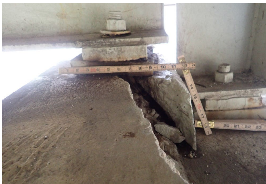
Figure 13.6.1 Spalling of Concrete Bridge Seat Due to High Edge Stress
