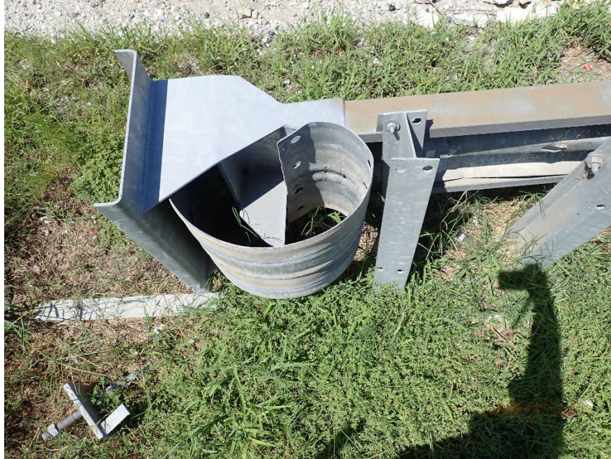
Figure 8.6.8 Boxing Glove Damaged by Impact
