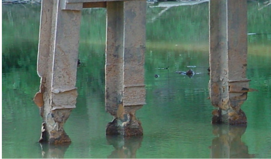
Figure 16.2.13 Steel Pile Deterioration Visible at Low Water Flow
