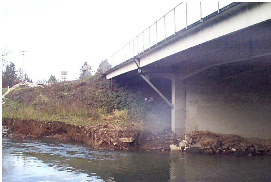
Figure 16.1.22 Channel Degradation due to Lateral Migration
