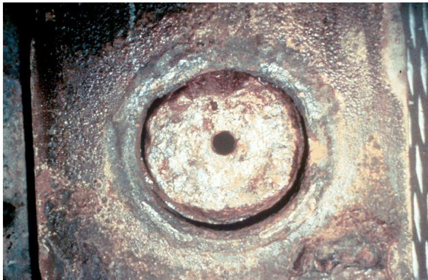
Figure 10.4.33 Corroded Pin-and-Hanger Assembly
