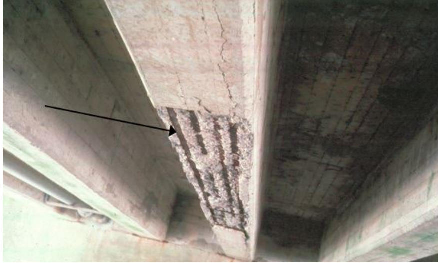
Figure 7.1.3 Spalled Concrete Member with Exposed Tensile Steel Reinforcement
