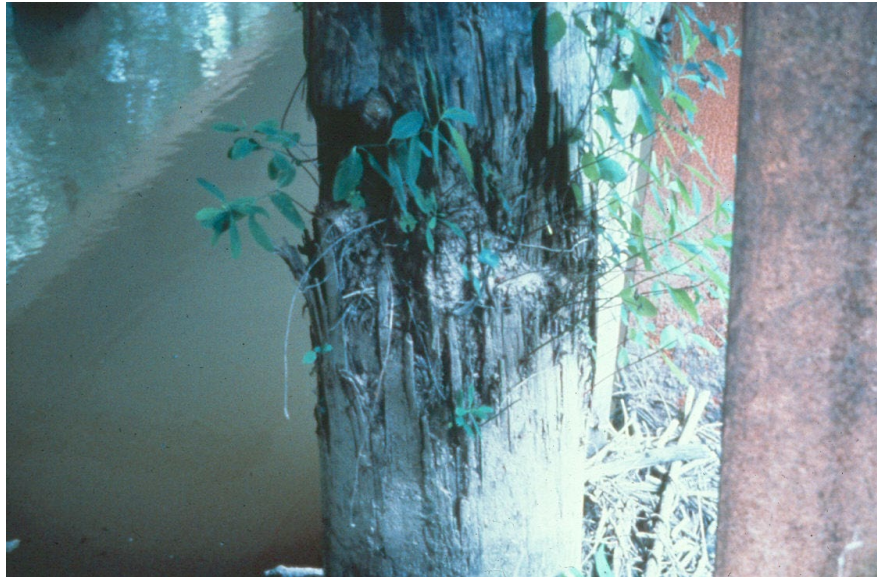
Figure 16.2.12 Timber Pile Deterioration
