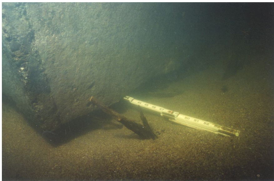
Figure 16.2.8 Local Scour - Causing Undermining of a Pier Footing
