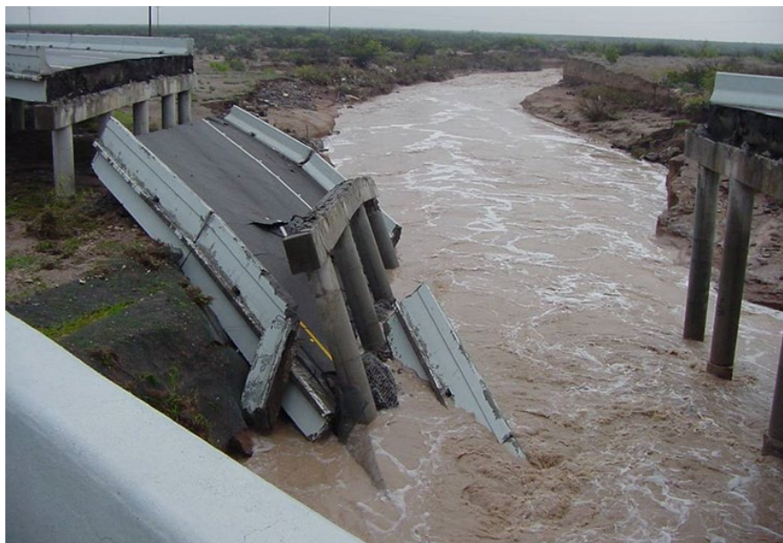
Figure 4.3.3 Pier Foundation Failure
