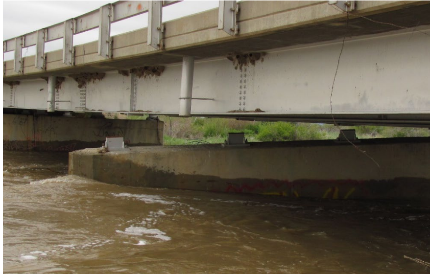
Figure 16.1.3 Pier Settlement due to Undermining
