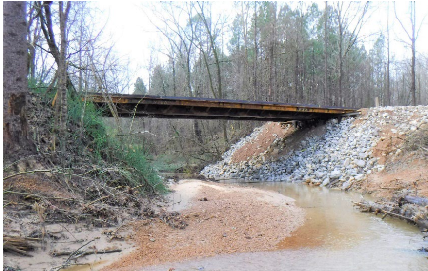
Figure 10.1.114 Railroad Car Converted Bridge without Bridge Railing
