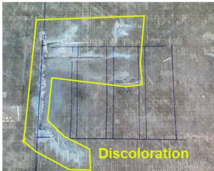
Figure 7.6.16 Cracks and Discoloration Around Punched Area
