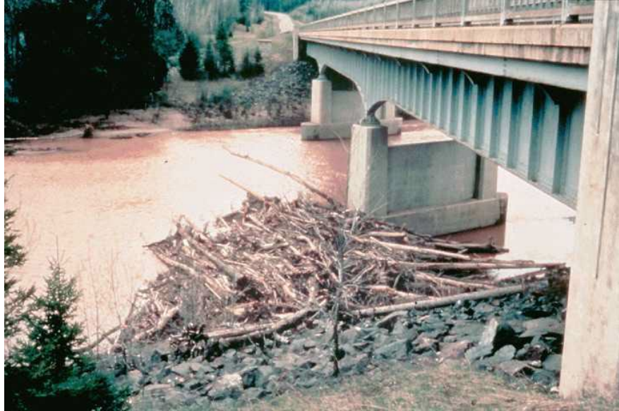
Figure 16.1.12 Debris Build-up in the Waterway
