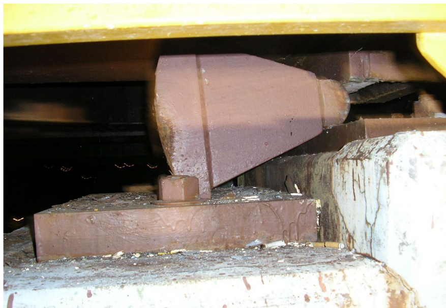
Figure 13.6.9 Overturned Rocker Bearing
