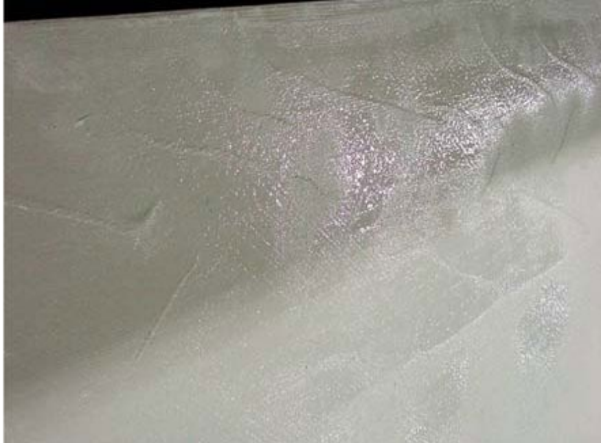
Figure 7.6.14 Wrinkling of FRP Fabric
