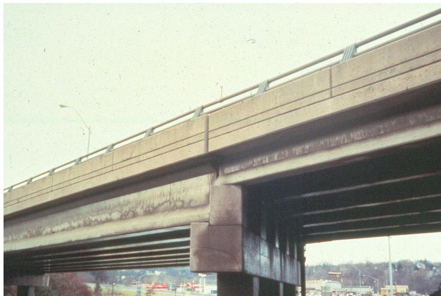
Figure 9.4.39 Water Leakage at Deck Joint Between Spans
