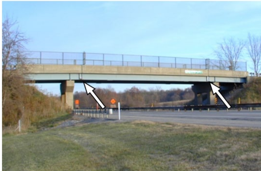
Figure 10.1.74 Typical Pin-and-Hanger Assemblies at Locations Relative to Piers
