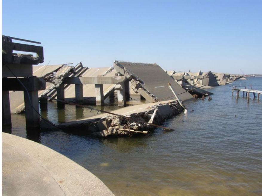
Figure 4.3.2 Failure Due to High Water Levels During Hurricane: Close-Up View
