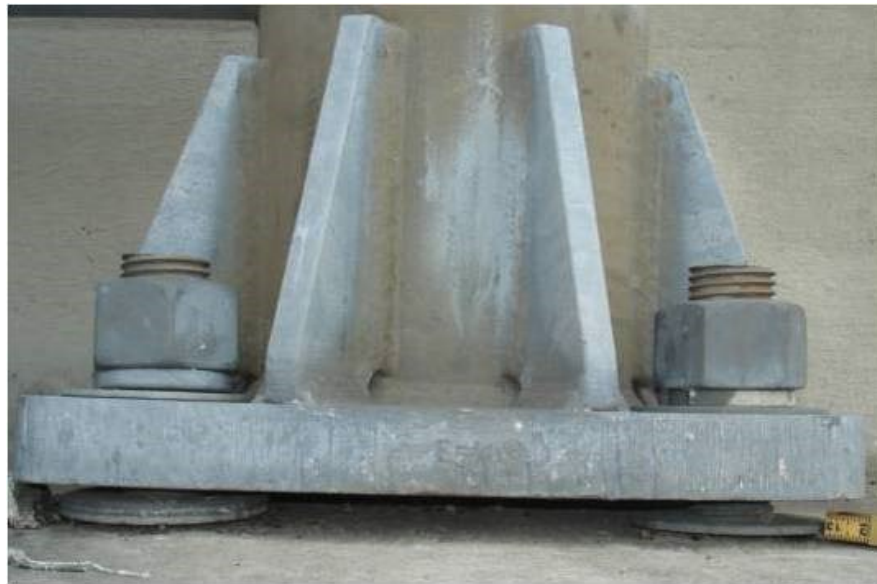
Figure 8.5.35 Sign Attachment Exhibiting Anchor Pullout
