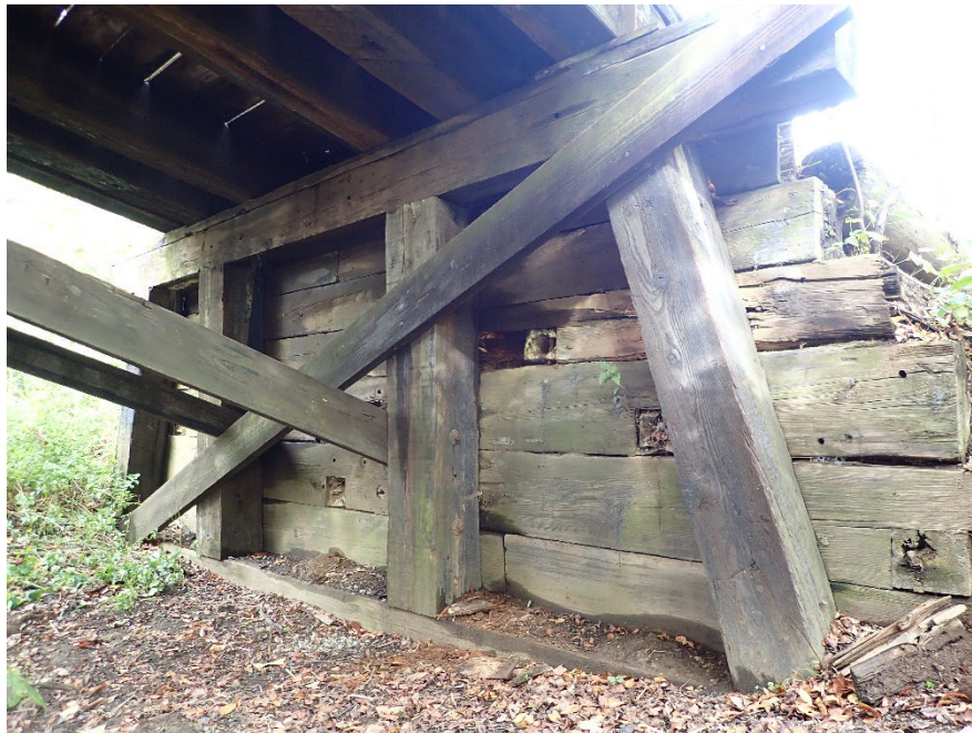
Figure 14.5.34 Decay on Timber Abutment
