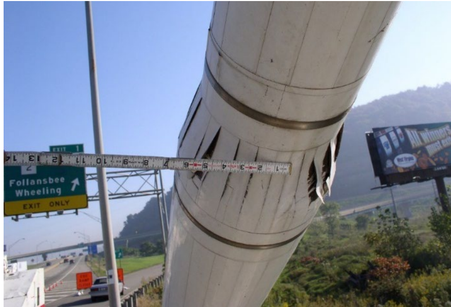
Figure 12.2.5 Deformed Cable Wrapping – Possible Broken or Corroded Wires
