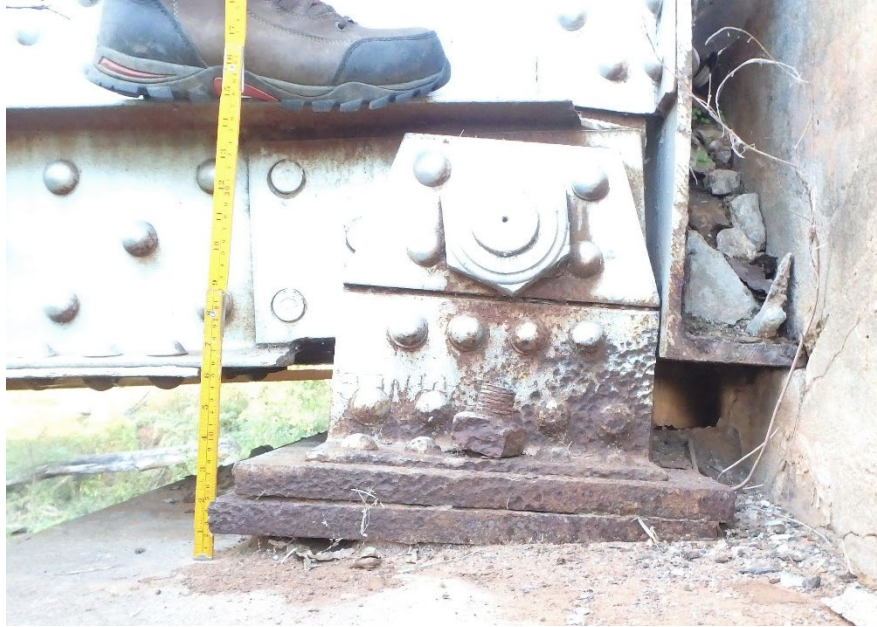
Figure 14.5.8 Bearing Displacement Indicating Possible Movement of Abutment
