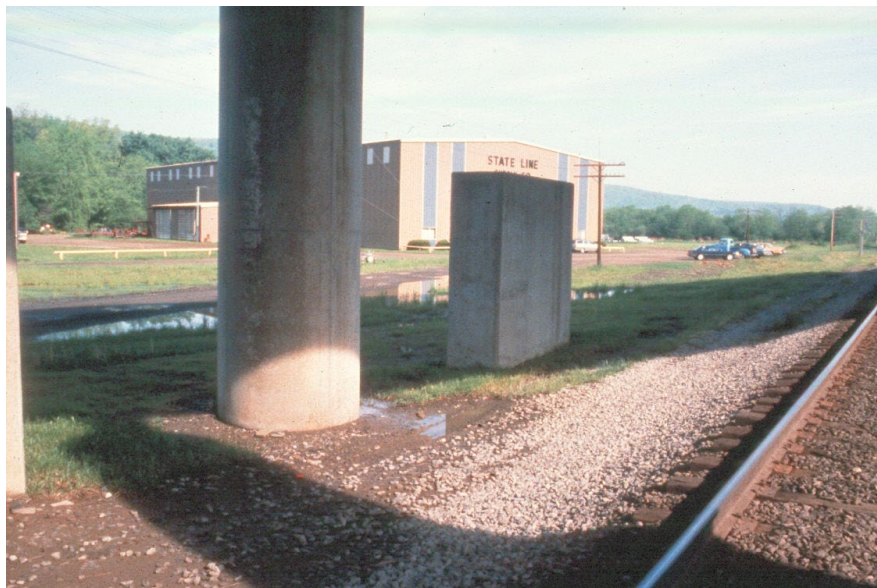
Figure 14.2.62 Concrete Collision Protection Block
