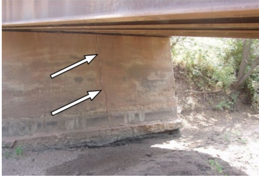
Figure 14.5.5 Crack in Abutment due to Differential Settlement
