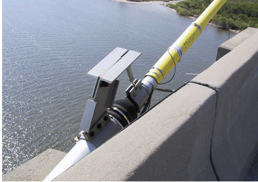
Figure 12.2.15 Small Shock Absorber Damper
