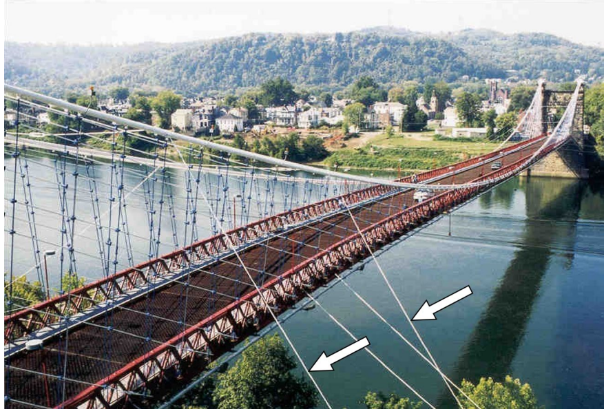
Figure 5.2.19 Cable Damping System for Suspension Bridge
