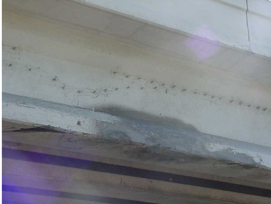
Figure 9.4.45 Collision Damage Repair on Prestressed Concrete I-Beam
