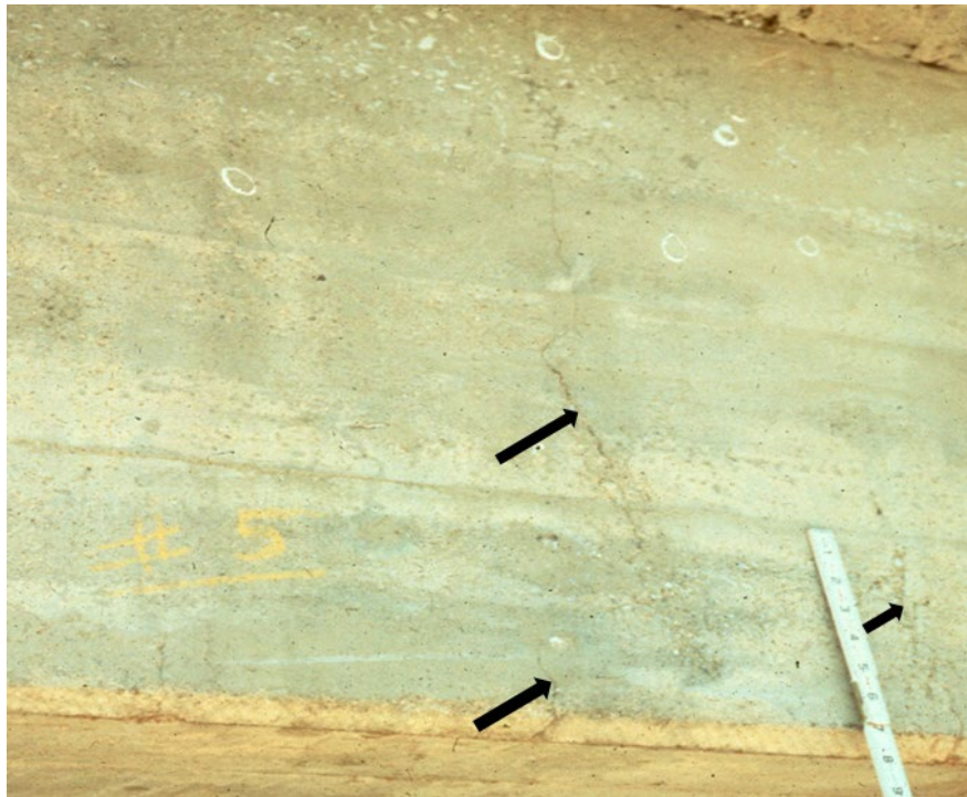
Figure 7.1.11 Flexural Cracks on a Tee Beam
