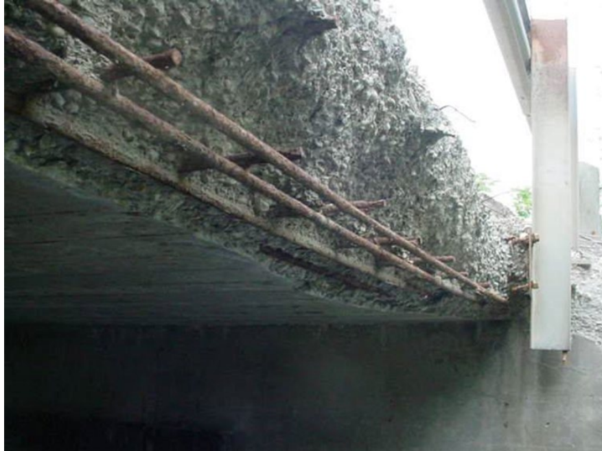
Figure 7.1.34 Corroded Reinforcing Bars with Severely Spalled Concrete
