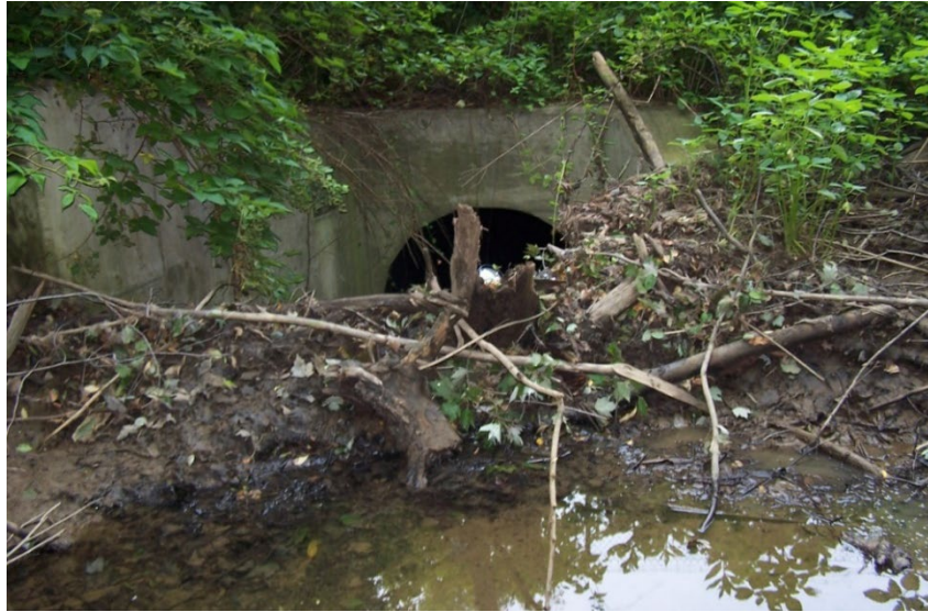
Figure 15.5.23 Debris and Sediment Build-up
