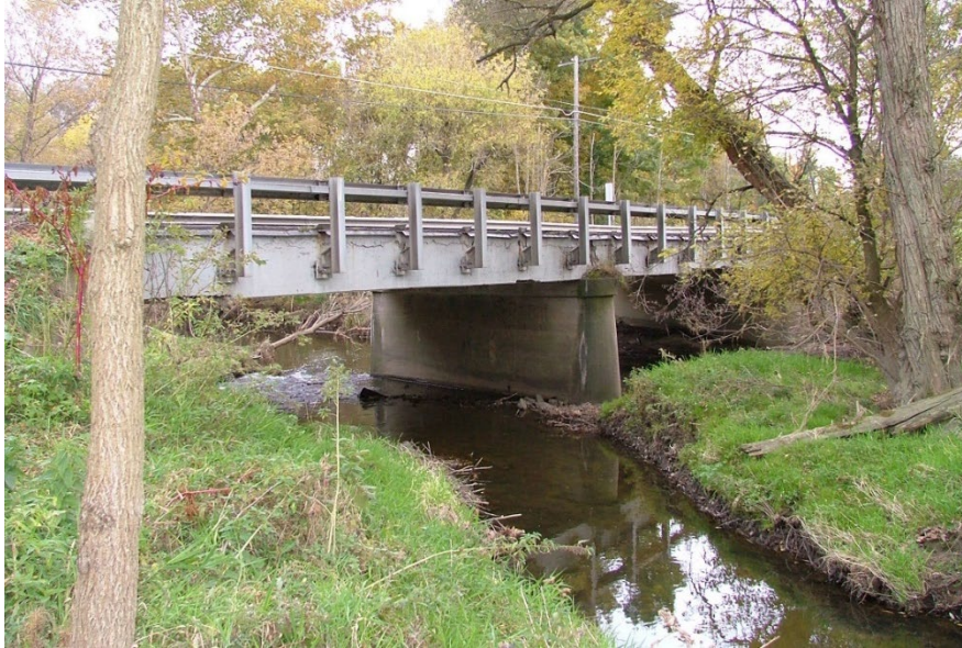
Figure 16.1.42 Sediment Accumulation Redirecting Streamflow
