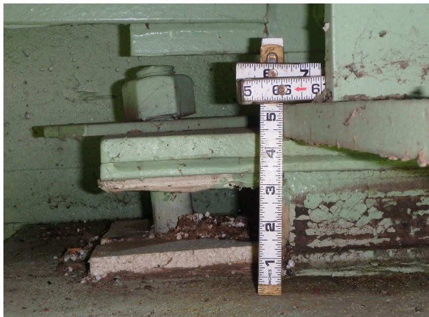
Figure 13.6.4 Bent Anchor Bolt due to Excessive Movement
