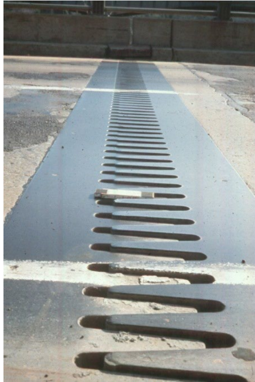
Figure 8.5.27 Improper Vertical Alignment at a Finger Plate Joint
