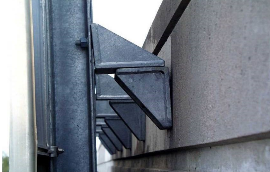
Figure 8.5.36 Sign Mount with Loose Adhesive Anchorage
