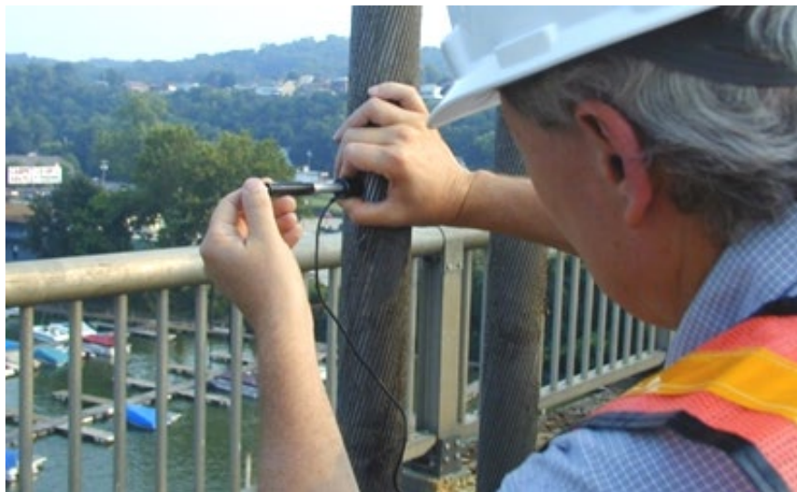
Figure 10.4.16 Hardness Test on Fire Damaged Arch Cables
