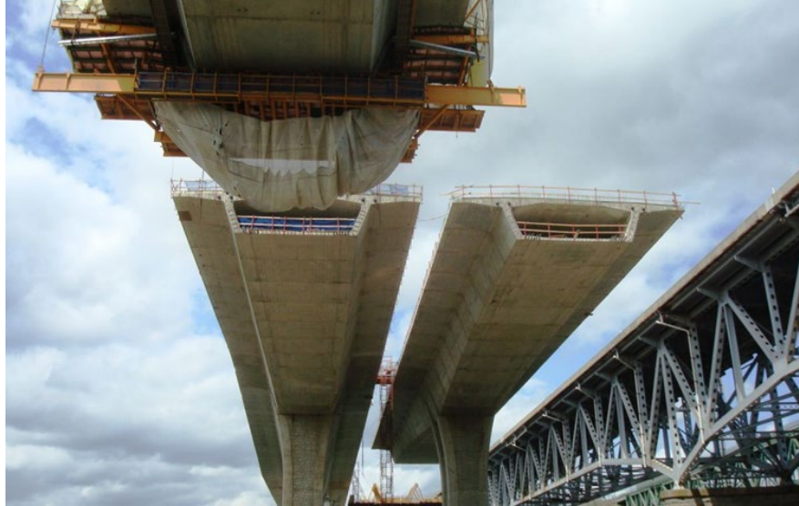
Figure 7.1.8 Post-tensioned Concrete Segmental Box Girders
