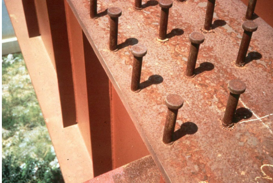
Figure 4.1.29 Shear Studs on Top Flange of Girder (before Concrete Deck is Placed)
