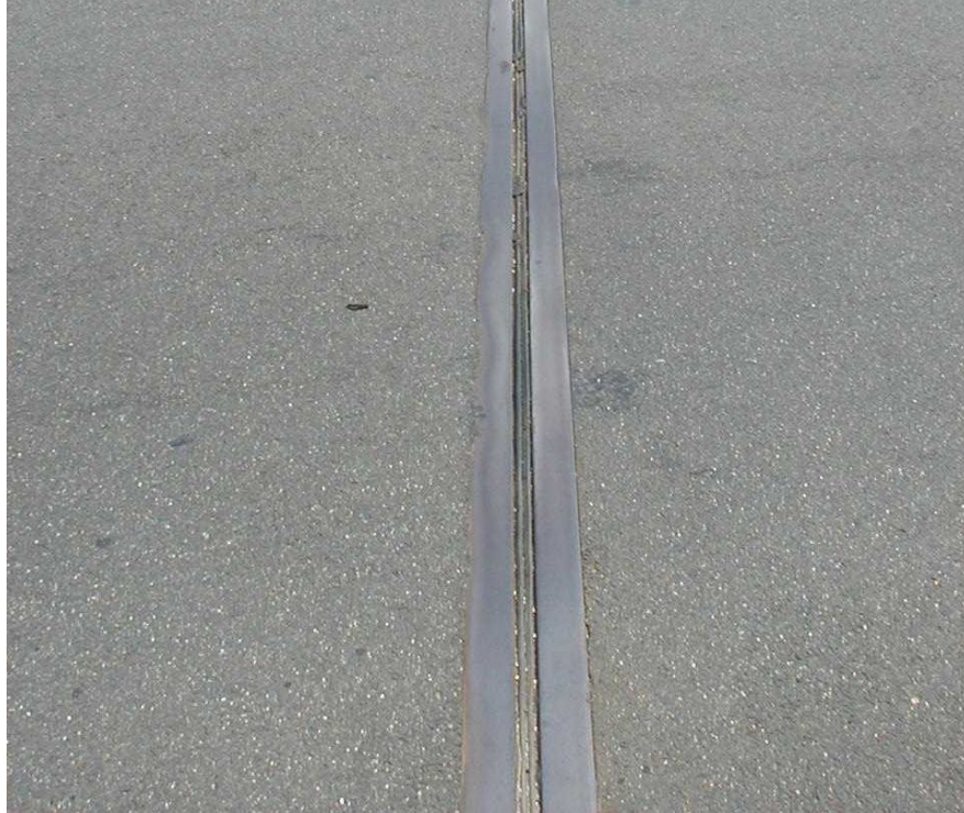
Figure 4.1.35 Top View of an Armored Compression Seal in Place
