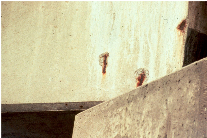
Figure 9.4.10 Exposed Shear Reinforcement at End of Box Beam
