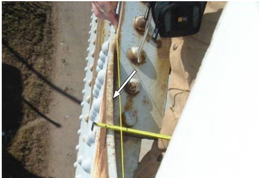
Figure 10.4.44 Gusset Plate Out-of-Plane Distortion
