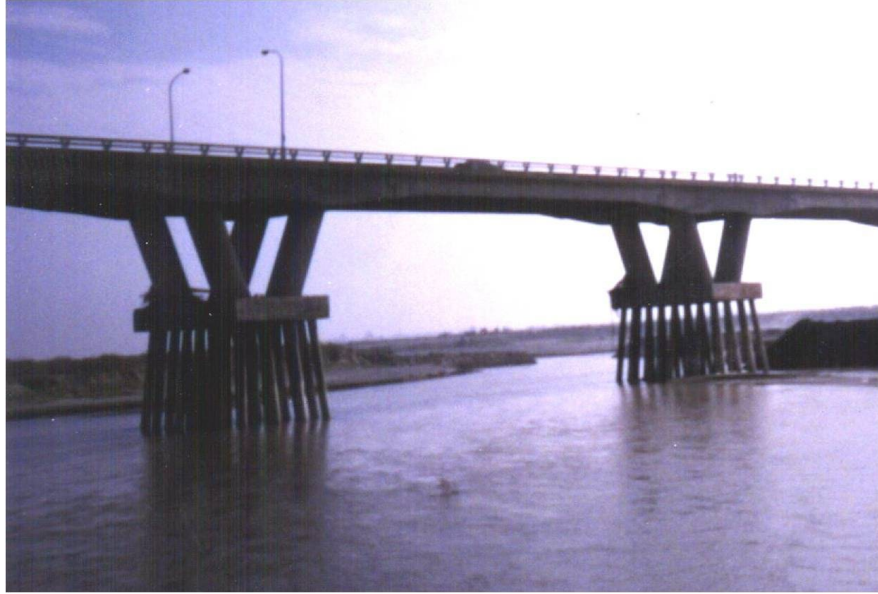
Figure 16.1.15 Micro-piles Exposed by Scour
