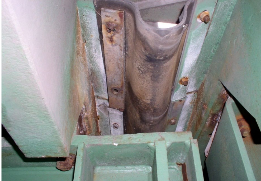
Figure 8.5.23 Drainage Trough with Missing Bolts
