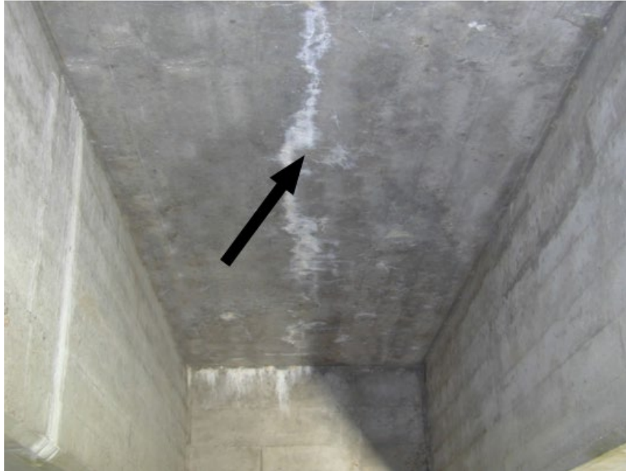
Figure 8.1.8 Underside View of Concrete Deck Longitudinal Crack and Efflorescence
