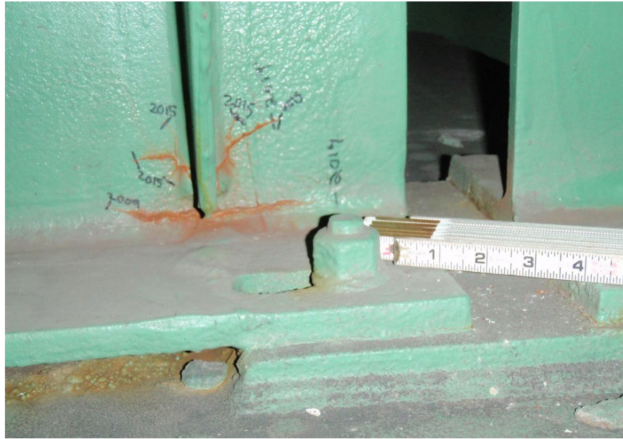
Figure 7.3.37 Web Gap Crack between Bottom Flange and Vertical Stiffener
