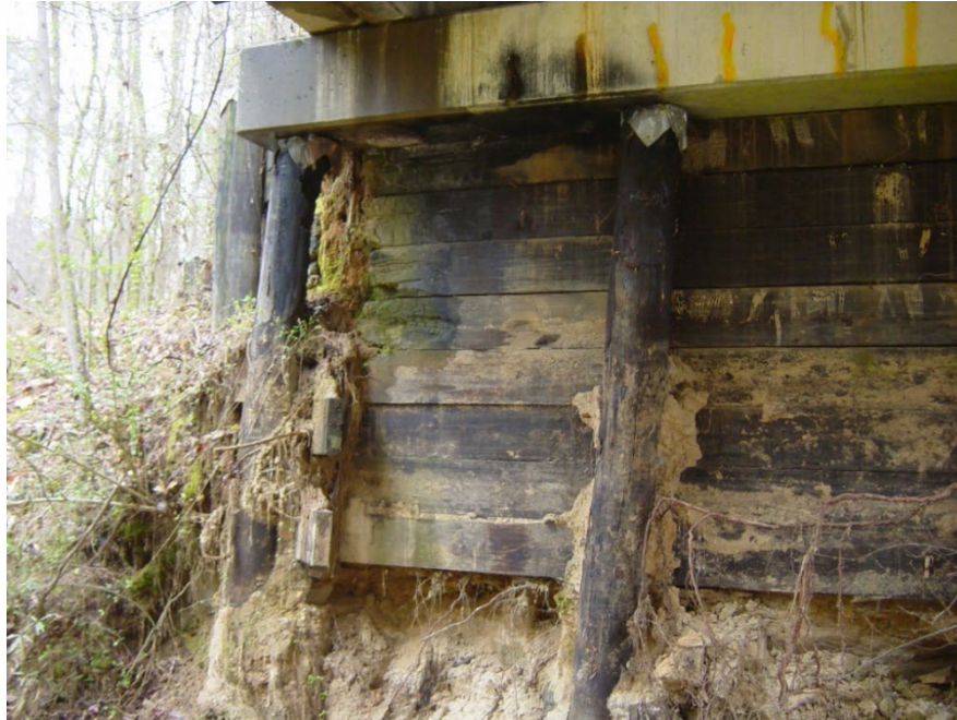
Figure 16.1.48 Bridge Abutment Affected by Scour
