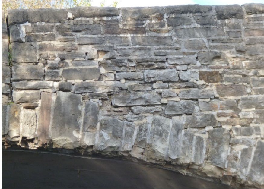
Figure 11.5.12 Masonry Arch Spandrel Wall with Widespread Mortar Deterioration
