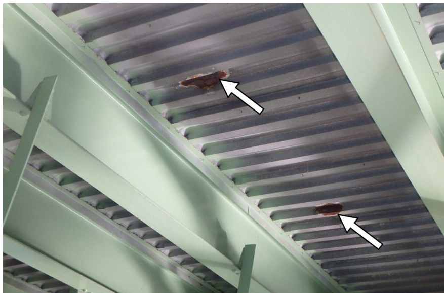
Figure 8.1.9 Stay-in-Place Form with Isolated Rusting
