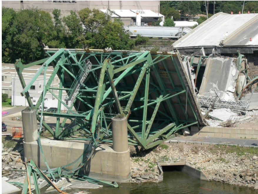
Figure 7.3.3 I-35W Mississippi River Bridge Collapse
