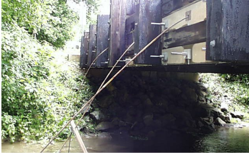
Figure 11.5.9 Broken Stressing Rods
