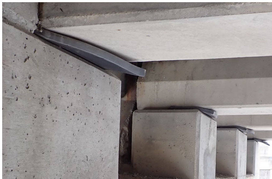
Figure 13.6.15 Plain Bearing Pads Walking Out from Under Beams
