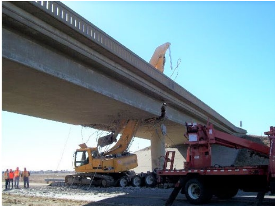
Figure 18.5.1 Bridge Damage from Construction Equipment
