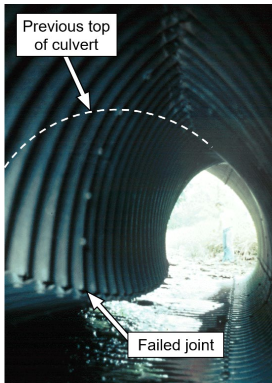
Figure 15.5.7 Flexible Pipe Culvert Bending Failure
