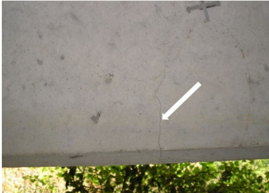
Figure 9.4.18 Flexure Cracks on a Tee Beam Stem
