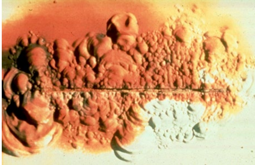
Figure 7.2.16 Rust Undercutting at Scratched Area
