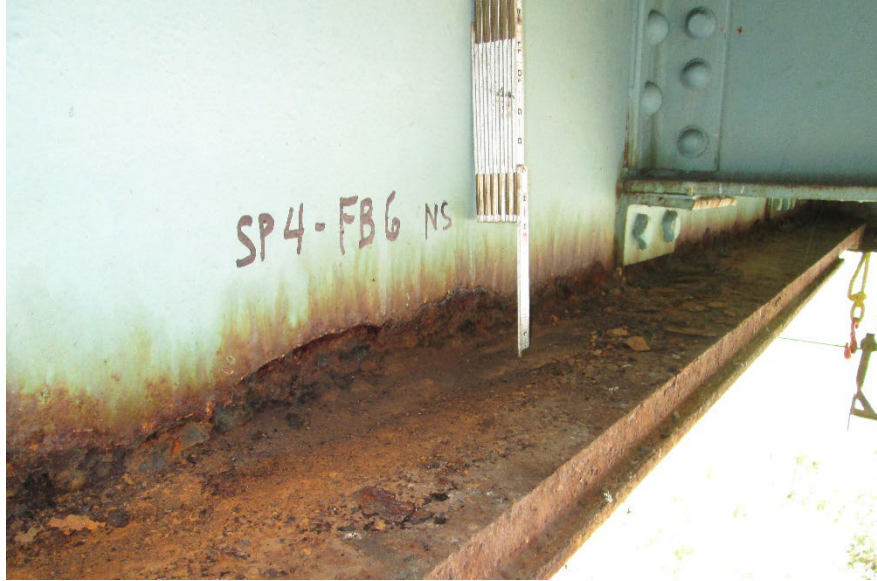
Figure 10.4.19 Corrosion on Top of Floorbeam Bottom Flange
