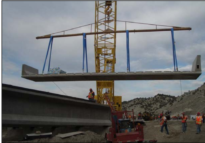
Figure 2.1.1.7-1. Eight Point Pick of a Precast Concrete Deck Panel. (Source: Utah DOT).
