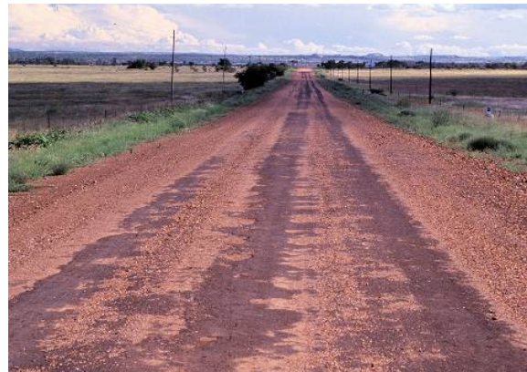
Figure 70. Photo. Insufficient additive application.
