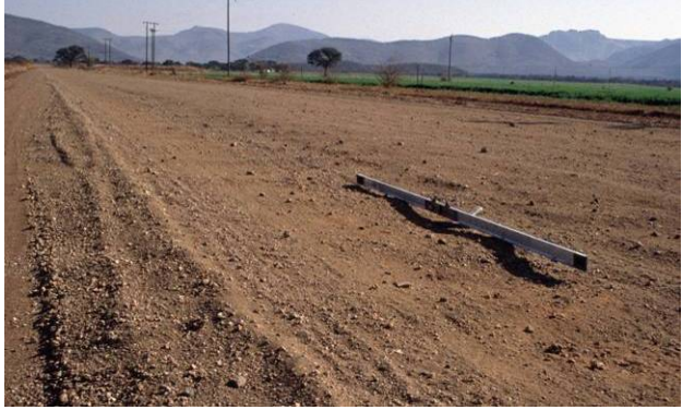
Figure 39. Photo. Washboarding and raveling.
