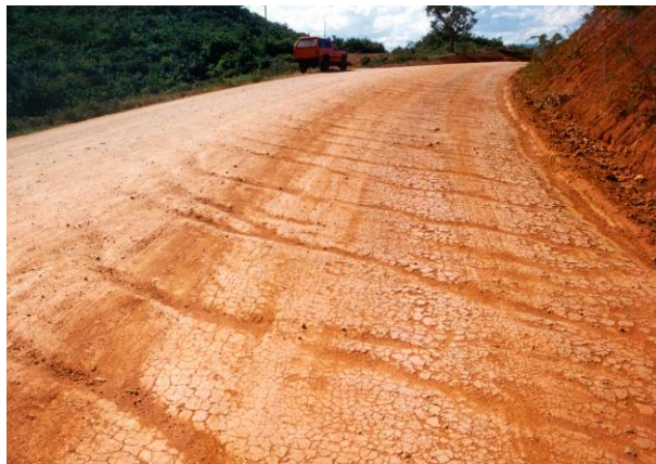
Figure 36. Photo. Transverse erosion.
