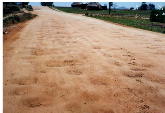
Figure 23. Photo. Potholes caused by poor drainage.
