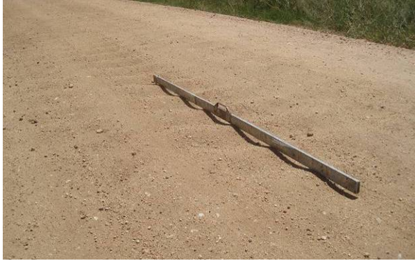
Figure 38. Photo. Washboarding (corrugation).
