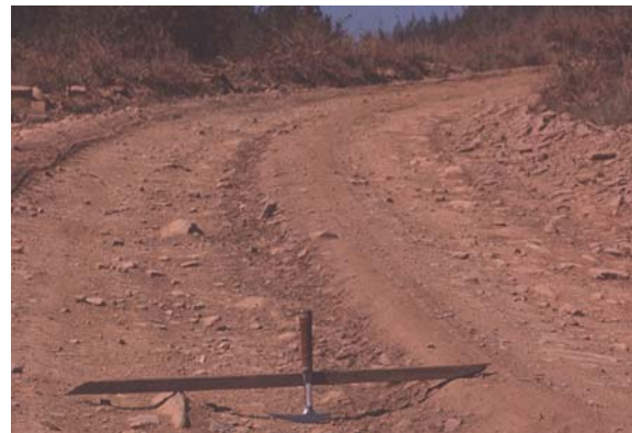
Figure 2. Photo. Poor unpaved road.
