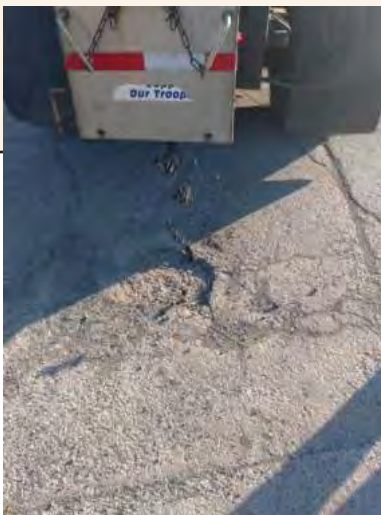
© 2023 Town of Rutland Highway Dept., NY
