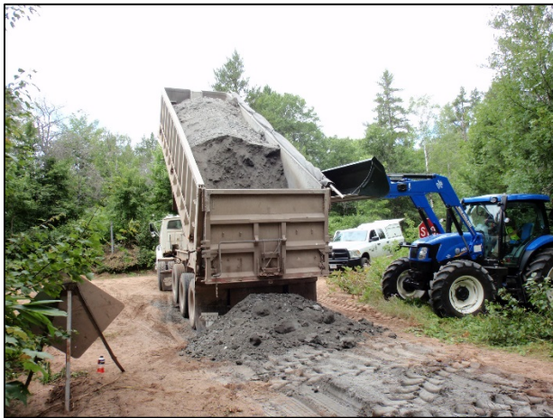
Ash delivered to unstable road.
