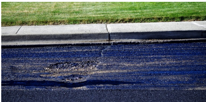
Figure 14: Irregularities in the base affect asphalt yields
