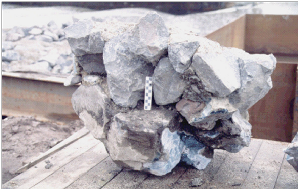
Figure 5.21. "Conglomerate" of partially grouted riprap, Federal Waterway Engineering and Research Institute, Karlsruhe, Germany (Heibaum 2000).
