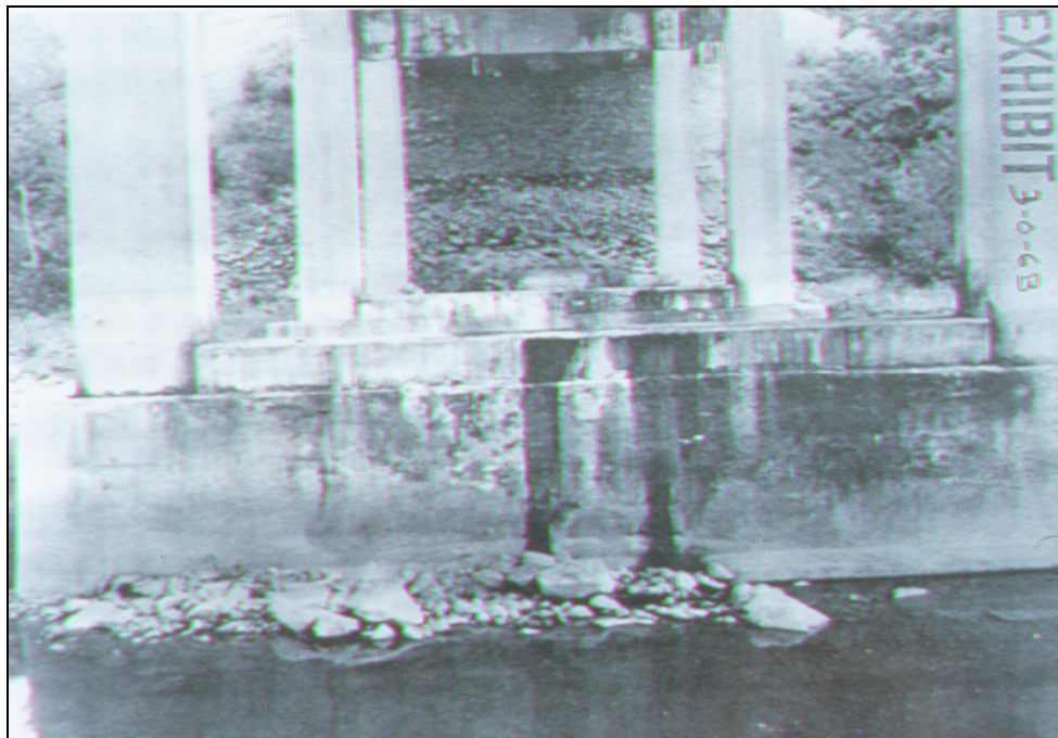
Figure 5.19. Photograph of riprap at pier 2, August 1977 (flow is from right to left).
