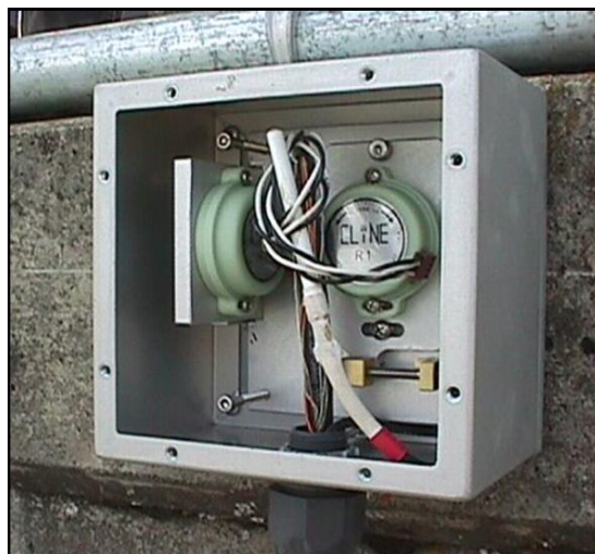
Figure 9.19. Detail of tilt meter.
