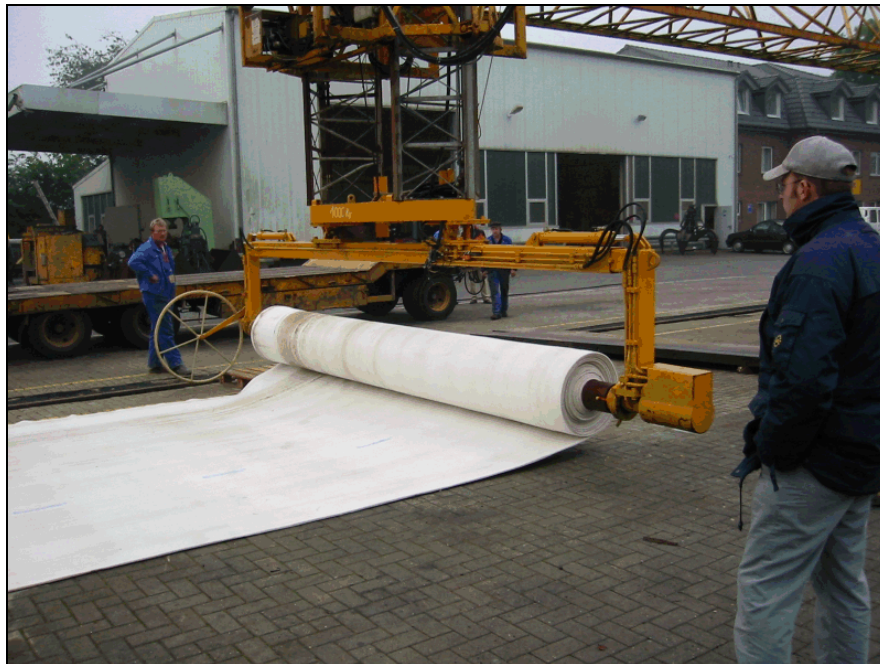
Figure 5.3. SandMat™ geocomposite blanket being unrolled. (photo from NCHRP Project 24-07(2), courtesy Colcrete – Von Essen Inc.)
