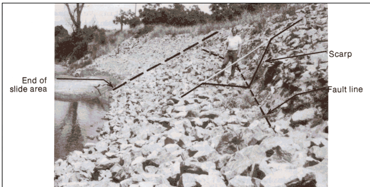
Figure 5.11. Riprap on Cosumnes River at Site 2 near Sloughouse, CA, looking downstream, showing translational slide failure (photographed May 31, 1983) (Blodgett & McConaughy 1986).
