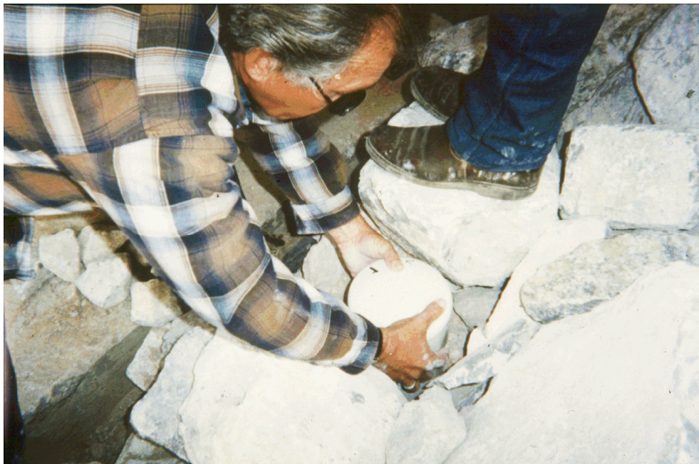
Figure 9.32. Installation of a float out device by Nevada DOT to monitor riprap stability.
