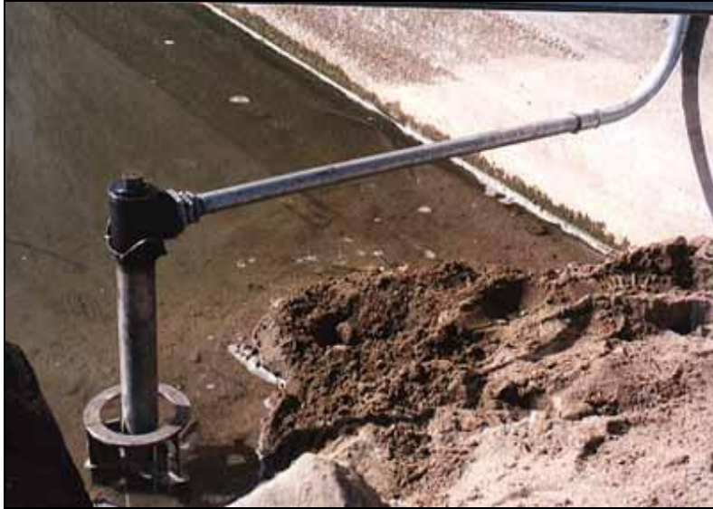
Figure 9.16. Detail of magnetic sliding collar on the streambed.
