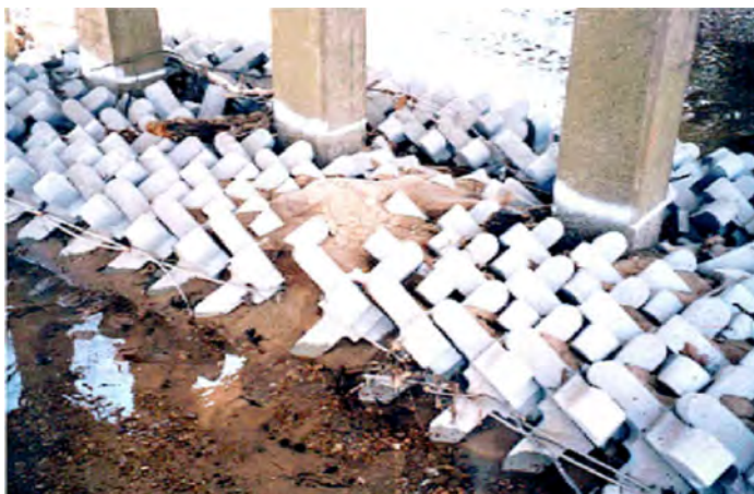
Figure 19.5c. Close-up of armor units after several flow events at Bridge 133, Graves County, KY
