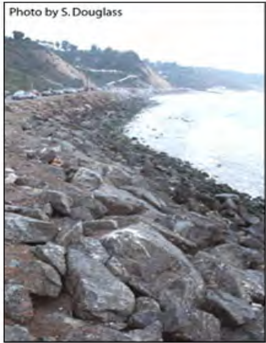
Figure 17.1. Riprap revetment in a wave environment, Pacific Coast Highway, California. (from HEC-25, 2nd Edition)
