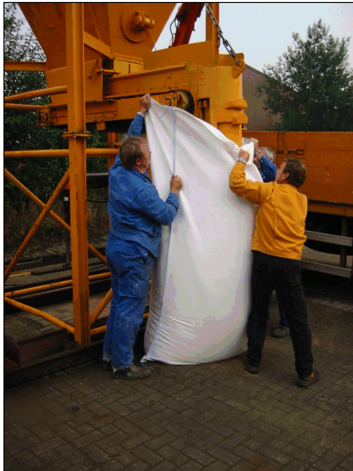
Figure 11.19. Filling geotextile container with sand. (photo from NCHRP Project 24-07(2), courtesy Colcrete – Von Essen Inc.)
