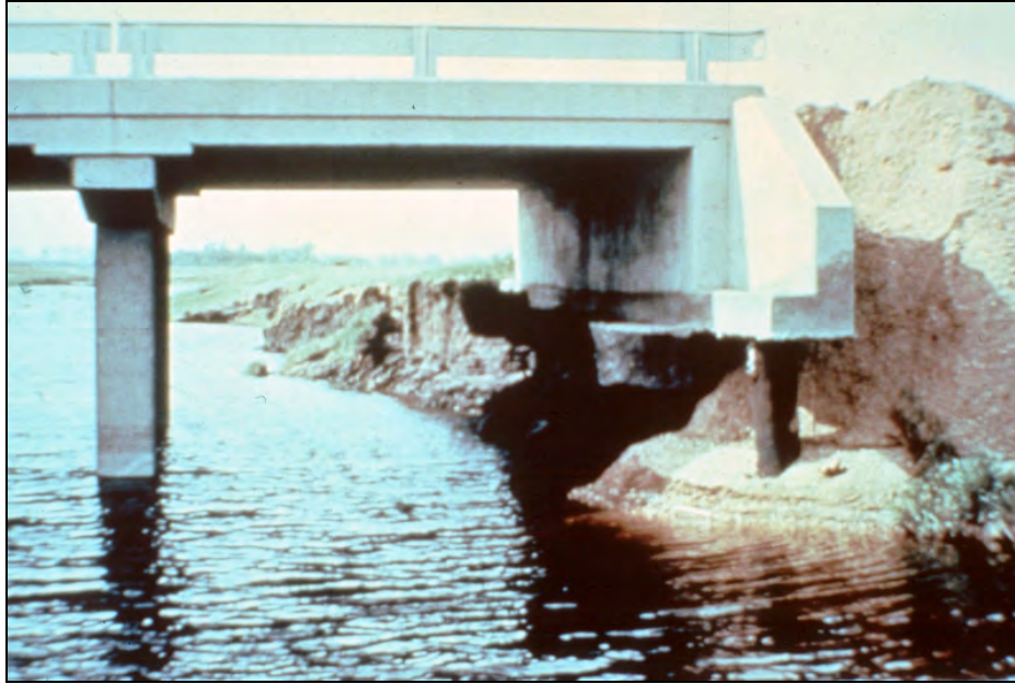
Figure 14.1. Scour of bridge abutment and approach embankment.
