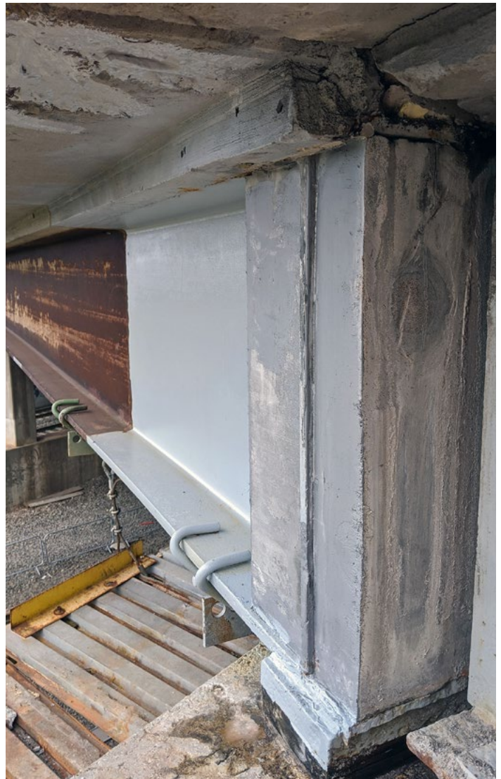
In this bridge beam end repair, the load is transferred from welded shear connectors to the UHPC and down to the pier.
