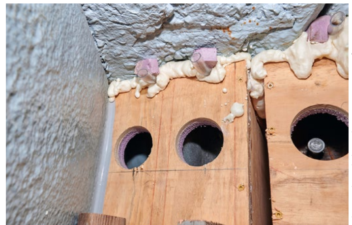
UHPC repair adapts well to working within the tight geometric restraints of beam end supports. This photo shows formwork in place prior to encasing the repair area in UHPC.
