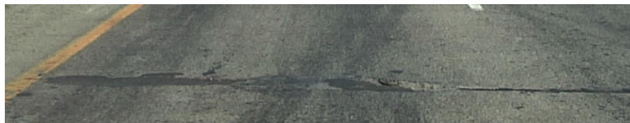
Figure 15. Image. Deteriorated bridge joint.
