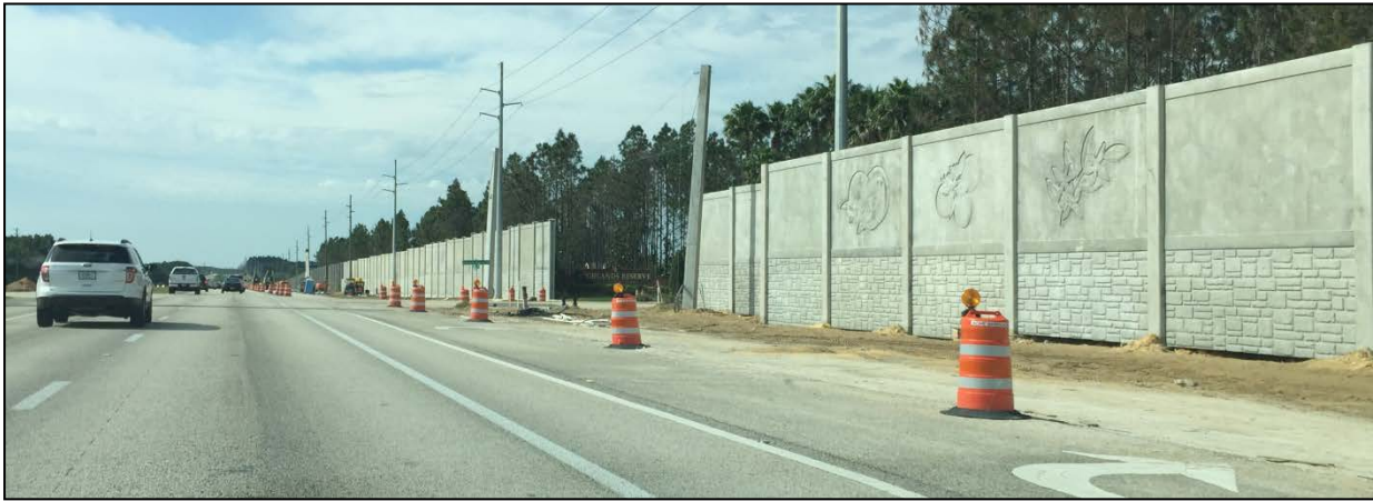
Figure 34. Nearly completed barrier at the entrance to Highlands Reserve along US 27 in Davenport, FL (Courtesy of FDOT).
