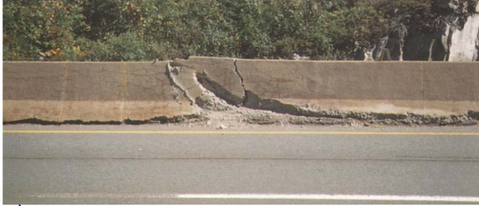
Failure of Jersey barrier due to expansion of concrete
