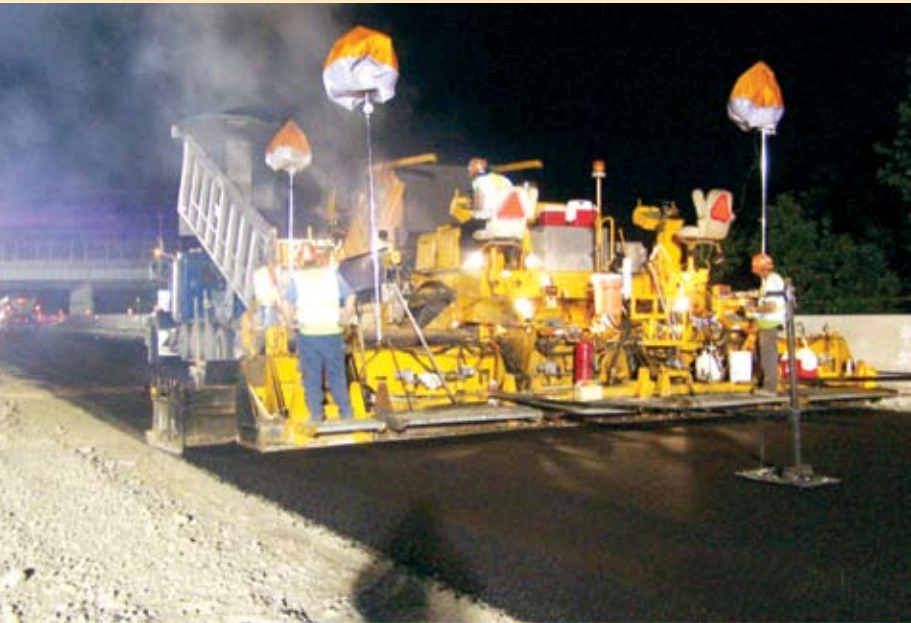
Rehabilitating existing roads while maintaining increasingly high levels of traffic requires innovative solutions such as night paving.
