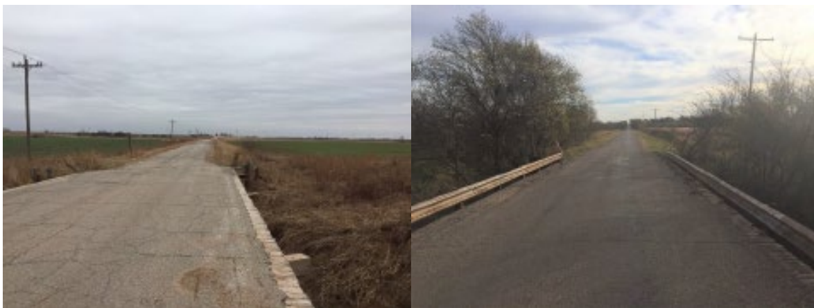
Image Source: Circuit Engineering District 8, Oklahoma. Existing bridge decks on two of the seven bridges.
