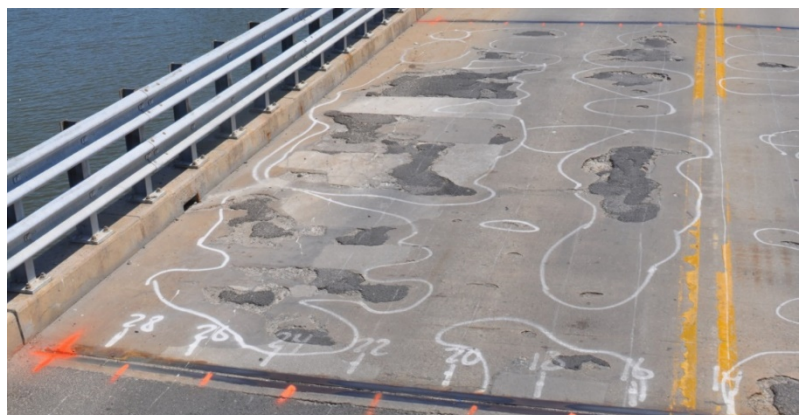
Figure 1. Example of a concrete bridge deck showing significant deterioration in the form of corrosion and delaminations. Photo courtesy by Thomas Schumacher.
