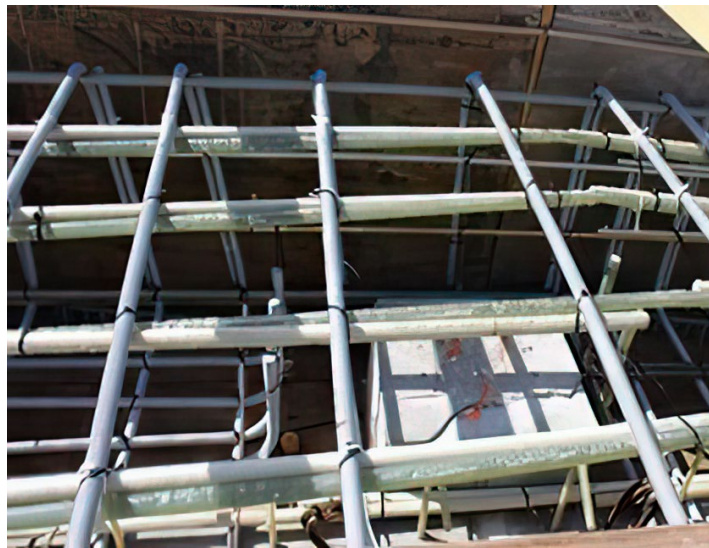
Figure 20. Photo. GRFP rebars in a pile bent cap. (Source FHWA).
