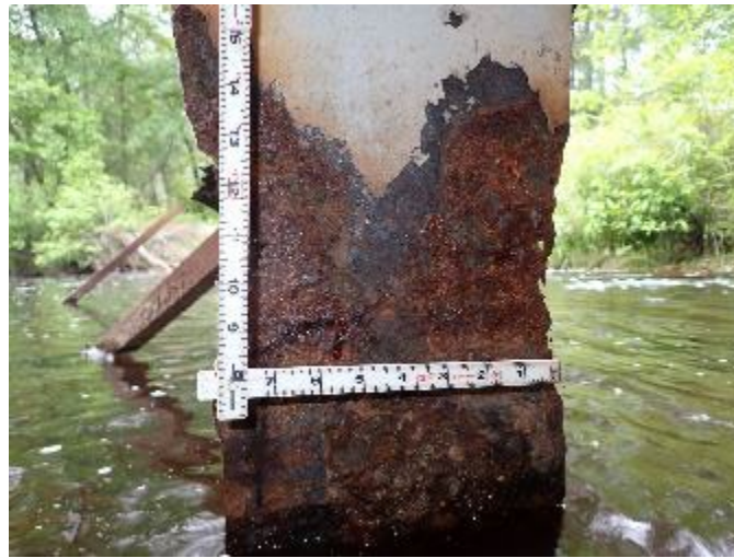
Figure 14. Photo. Steel pile corrosion at the waterline. (Source FHWA).
