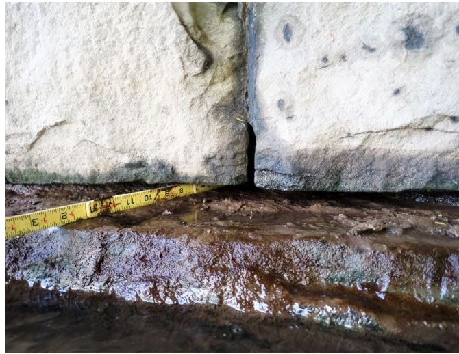
Figure 4. Photo. Masonry pier with weathered stone and mortar loss. (Source FHWA).
