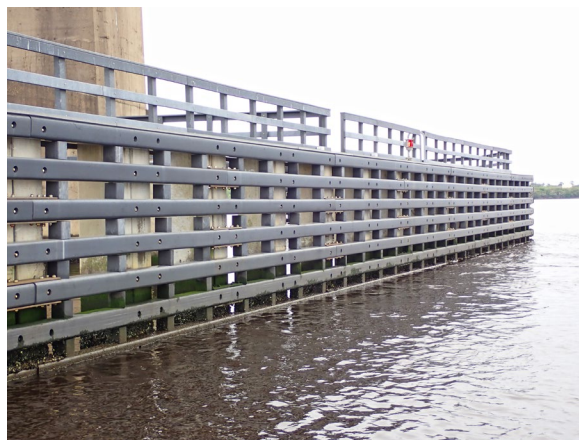
Figure 21. Photo. Composite fender system. (Source FHWA).
