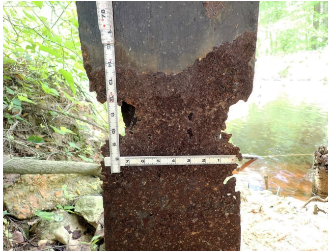
Figure 3. Photo. Extreme section loss in a steel pile. (Source FHWA).
