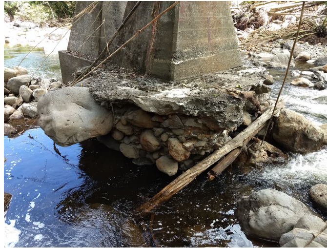
Figure 5. Photo. Undermined spread footing. (Source FHWA).
