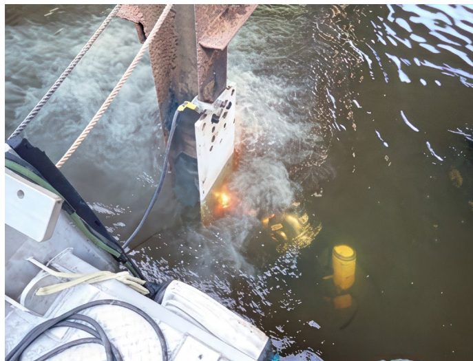
Figure 45. Photo. Diver cutting steel underwater with dangerous gasses forming on the surface. (Source FHWA).
