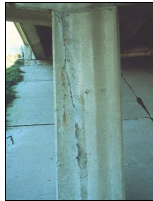
Figure 139. Crack in Pier 3 column. Location 3.
