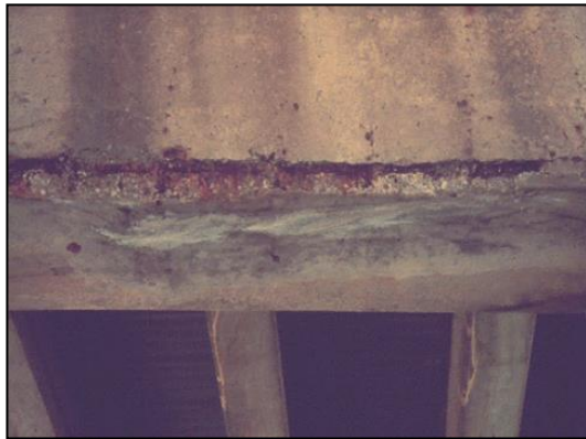
Figure 138. Spall in Pier 2 cap beam. Location 1.
