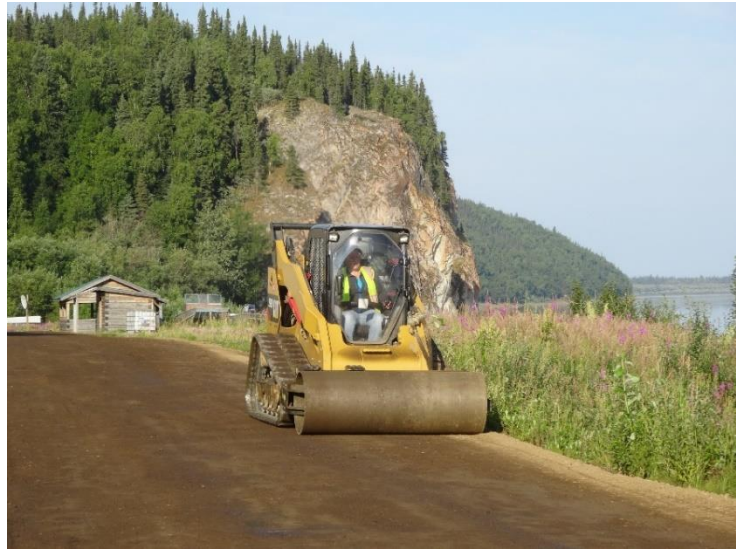
Figure 5. Compacting the finished roadway with a skid steer-mounted roller. Source: Native Village of Ruby
