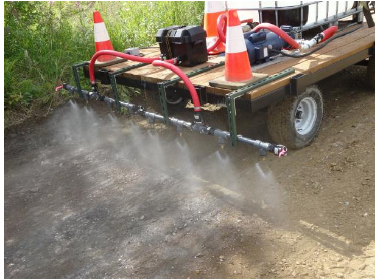
Figure 3. Spray bar applying the dust control product. Source: Native Village of Ruby
