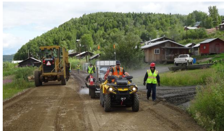
Figure 4. Application of the dust control product onto a prepared roadway surface. Source: Native Village of Ruby
