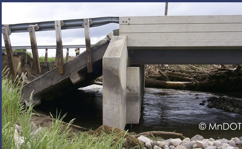
Figure 4: Flood damage at a bridge abutment.
