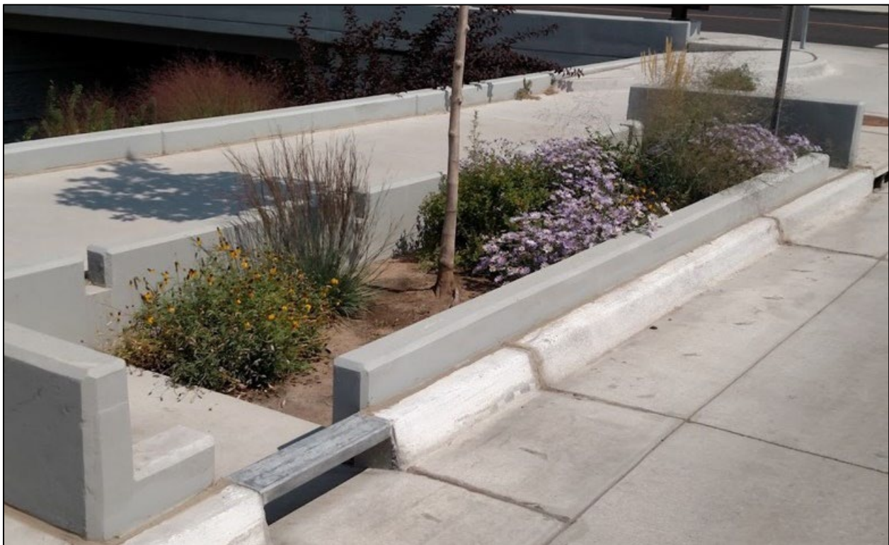
Figure 11.7. Green infrastructure practice: bioretention (rain garden). Source: Roger Kilgore.
