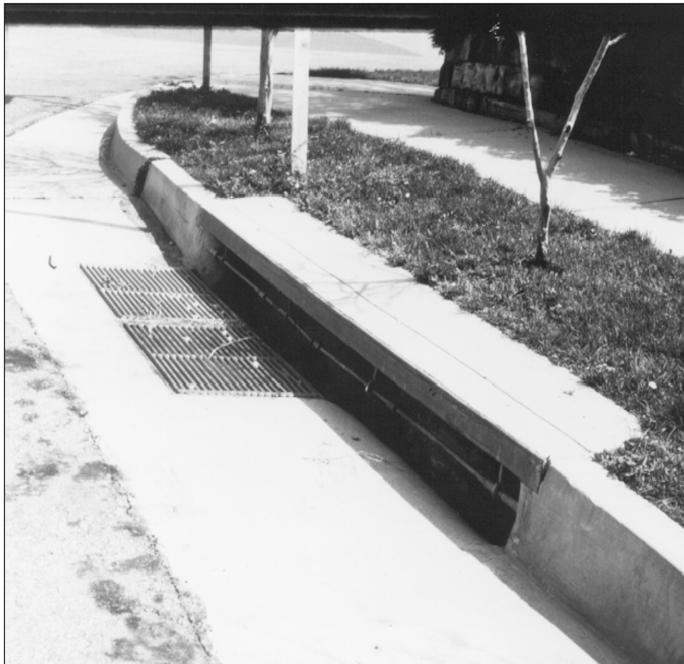
Figure 7.12. Sweeper combination inlet.
