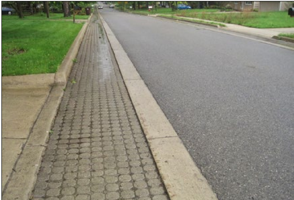
Figure 11.10. Green infrastructure practice: permeable pavers (USEPA 2021).
