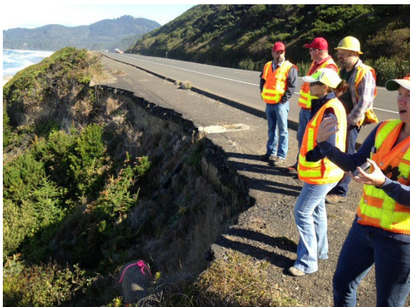
Figure 2. Evidence of road erosion (Source: Oregon DOT).
