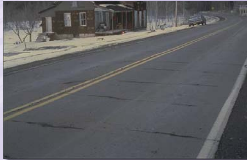
Low temperature thermal cracking
