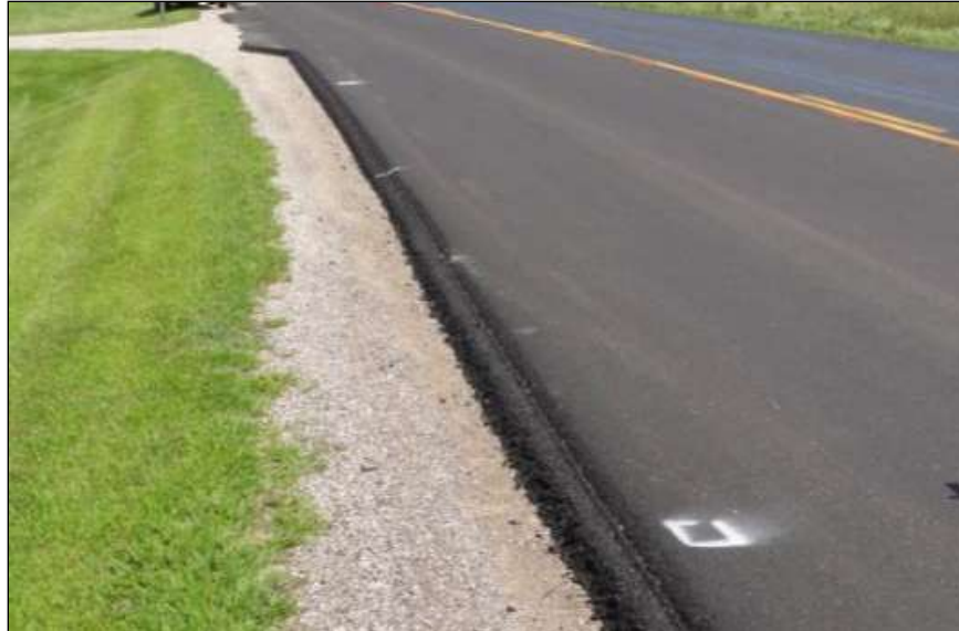
Figure 15. Typical view showing the base and intermediate course with Safety Edge SM and granular shoulder material. Image taken east of Sully.
