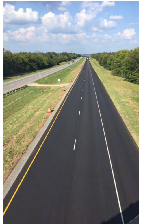
The Alabama Department of Transportation used microsurfacing for the first time on a project on Interstate 59.
