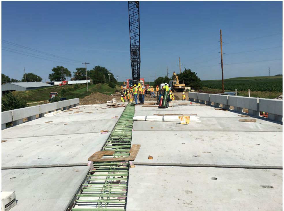
The Nebraska Department of Transportation chose UHPC to make the transverse connections between precast concrete deck panels on the Belden-Laurel bridge replacement.
