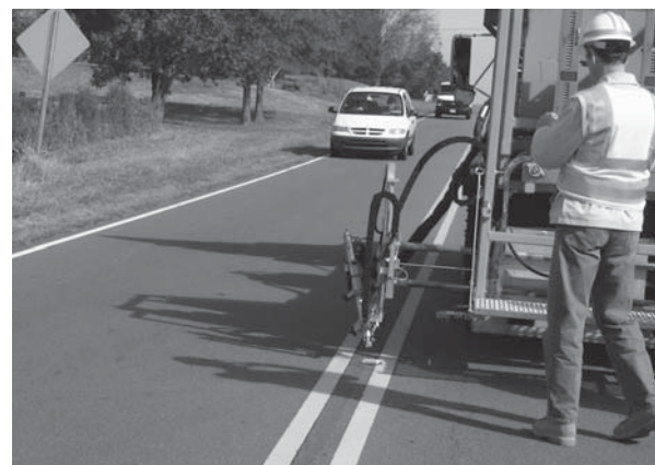
FHWA's Carl Andersen observed the operation of the automated pavement marker placement system during a field test.
