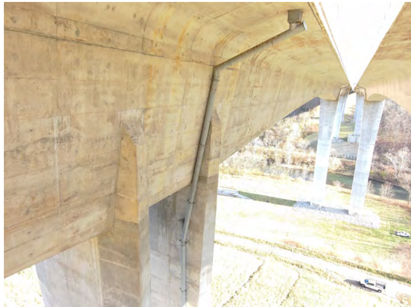
Drone Bridge Inspection of the Jeremiah Morrow Bridge, Warren County, Ohio - Ohio Department of Transportation
