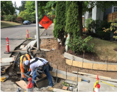
Figure 2: Lake Oswego DPW repairing a curb ramp. Image courtesy of Lake Oswego DPW.
