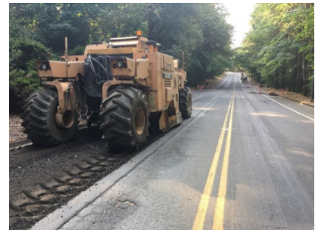
Figure 1: Lake Oswego's DPW repaves a section of road. Image courtesy of Lake Oswego DPW.
