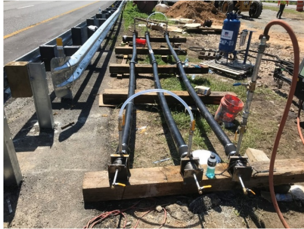
Figure 29. Photo. Mockup to simulate the ducts in the panels and the grouting process.
