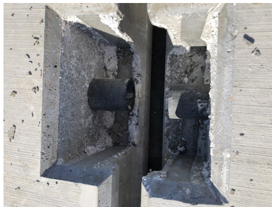
Figure 14. Photo. Close-up detail of the longitudinal joint at the tendon duct location.
