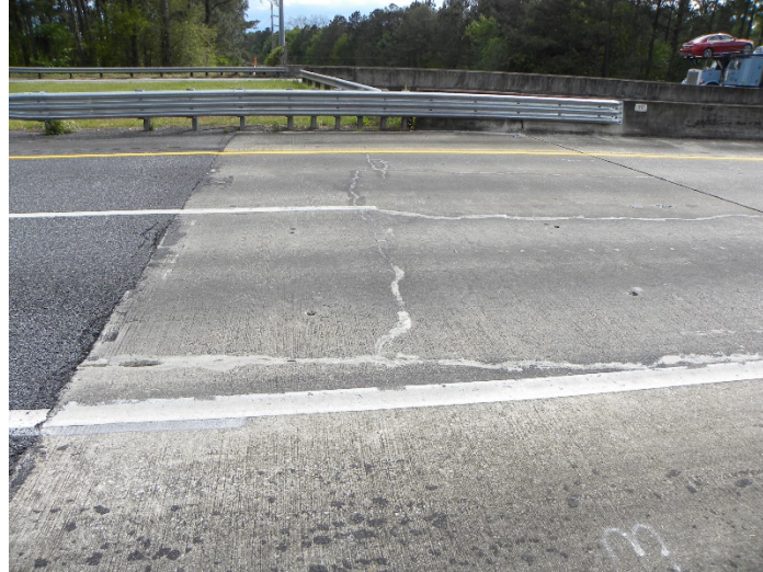
Figure 3. Photo. Condition of the existing bridge approach slab.
