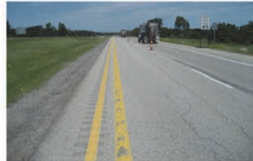
Load-Related Longitudinal Cracking
