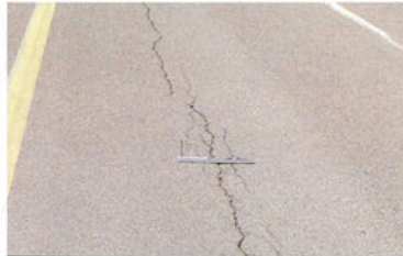
Longitudinal Cracking In the Wheel Path
