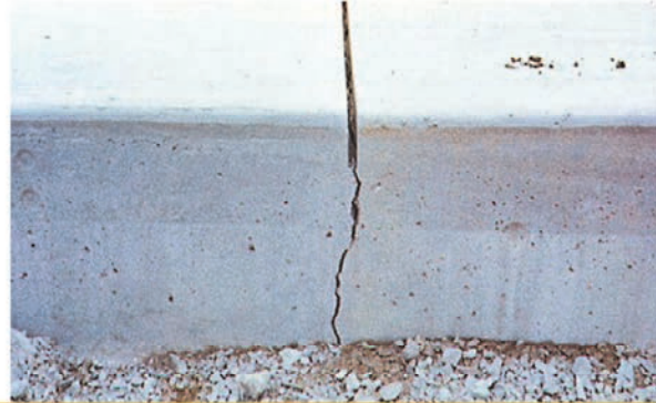
Sawed contraction joint with restrained shrinkage-induced crack.
