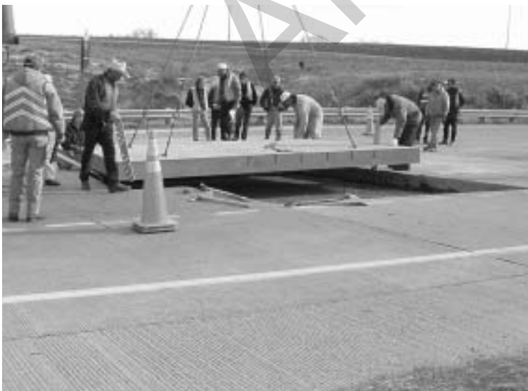
Full depth restoration is performed on US 287 near Fort Collins, Colorado, using precast concrete panels.
