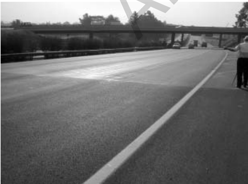
A surface treatment has been applied to this highway near Johannesburg, South Africa.
