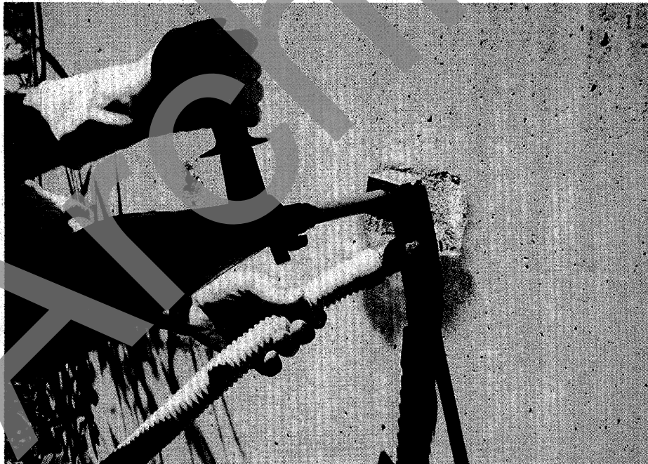
Fig 2-18 Bushhammering treated surface to remove uranyl acetate contaminated layer. Note hose attached to vacuum to collect powder and chips generated by bushhammering.
