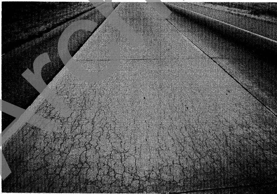
Fig 1-2 More generalized map cracking due to ASR in a jointed pavement.
