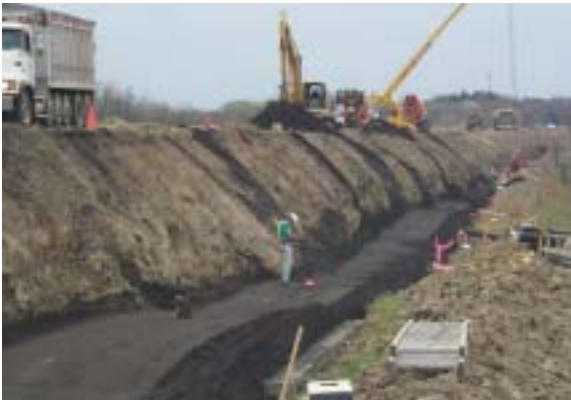
Figure 7. Embankment with foundry sand subbase (Ohio Turnpike, sand from Ford Motor Company supplied by Kurtz Bros. Inc.)
