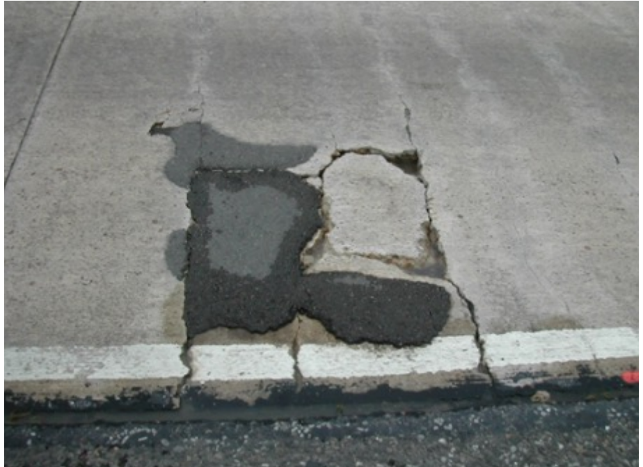
Figure 2. Punchouts require FDR. Source: TxDOT Pavement Manual 2021
