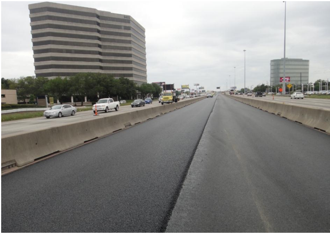
Figure 15. Construction surfaces of TOM (left) and CAM interlayer (right). Source: Tom Scullion, TTI
