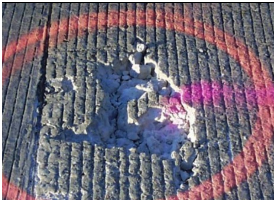
Figure 3. Deep spalling is typically rehabilitated using FDR. Source: TxDOT Pavement Manual 2021
