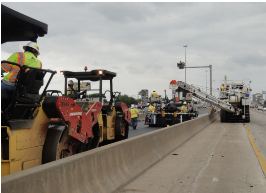
Figure 1. Construction of the Interstate 69 overlay system. Source: Tom Scullion, Texas A&M Transportation Institute.
