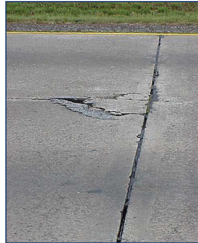
Figure 10. Example of corner breaks. (Source: TxDOT PMIS Rater's Manual 2016)
