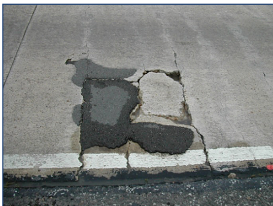
Figure 11. Punchouts require FDR. (Source: TxDOT Pavement Manual 2021)
