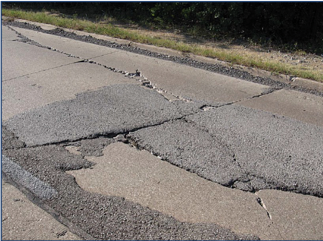
Figure 9. Shattered slabs need full-depth repair. (Source: TxDOT PMIS Rater's Manual 2016)
