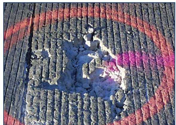
Figure 12. Deep spalling requires FDR. (Source: TxDOT Pavement Manual 2021)
