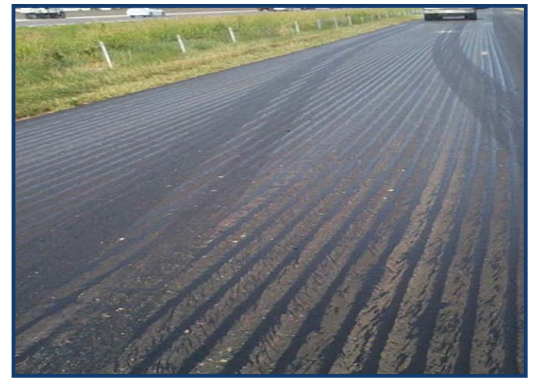
Figure 13. Inadequate tack coat application. (Source: FHWA)
