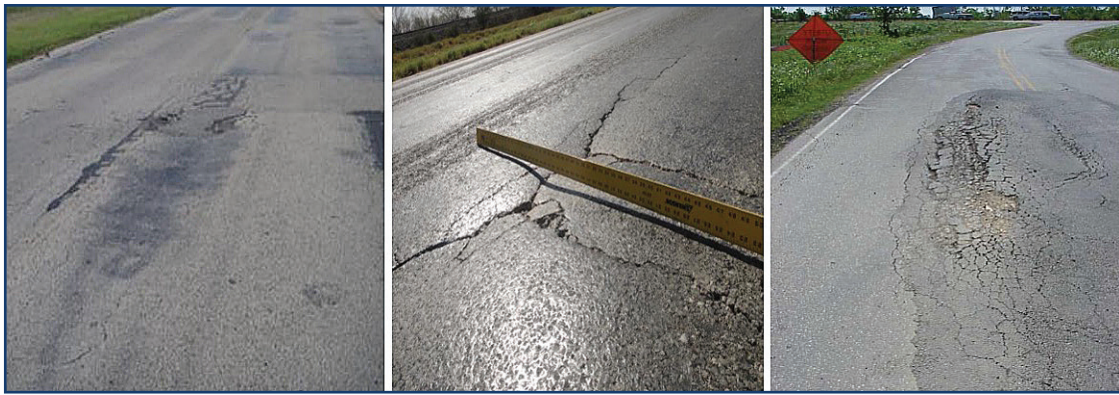
Figure 5. Poor candidates for HPTO. (Source: TxDOT)
