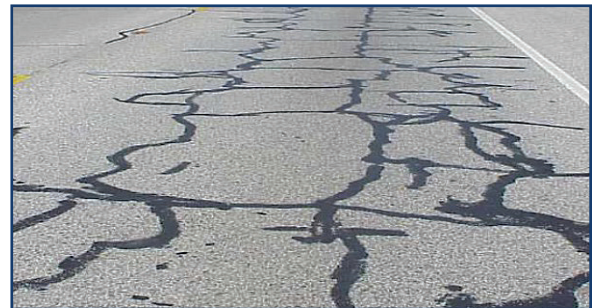
Figure 7. Pavement with existing block cracking good HPTO (TOM) candidate. (Source: TxDOT)
