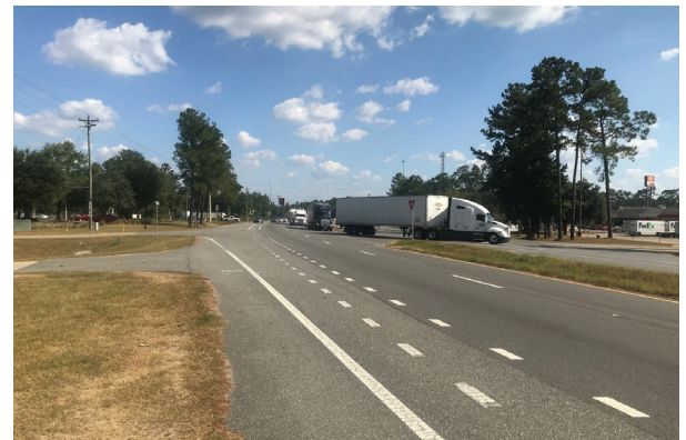
FDOT has monitored and evaluated HiMA overlay performance on U.S. 90 North in Midway since construction in 2015. Source: Gary Fitts.
