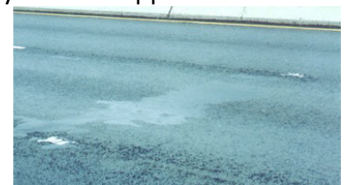
Figure 8: Transverse “rich” spot caused by a paver stop. (Source: D. Watson)
