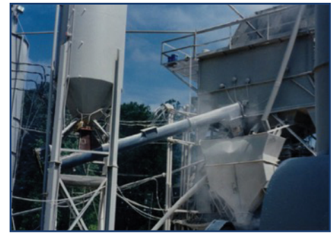
Figure 7: Silo modified with a larger opening for feeding mineral filler. (Source: NCAT)
