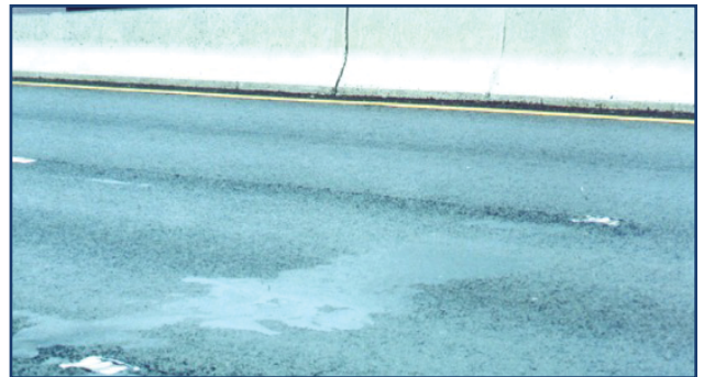
Figure 11: Transverse “bleeding” caused by paver stop. (Source: NCAT)
