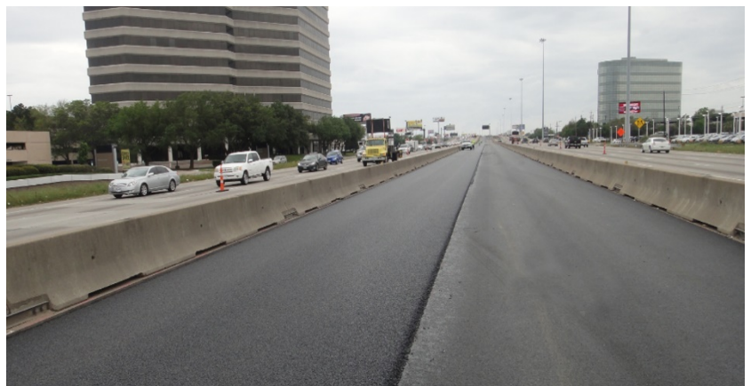
Crack attenuating mix on Houston's IH-69 project. Source: Tom Scullion, Texas A&M Transportation Institute
