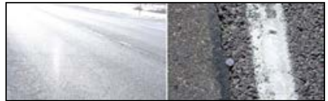
Figure 8. Transverse cracking (left) and longitudinal edge cracking (right). (Source: Musa Ruranika and Geib)
