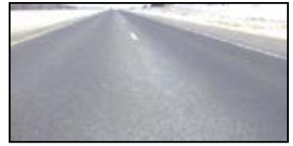
Figure 7. UTBWC overlay section after seven years of service. (Source: Musa Ruranika and Geib)
